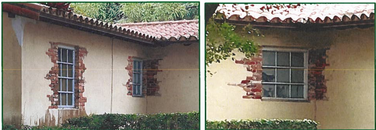
Figures 16: Brick ‘Shutter’ Wrapping the Corner at South Façade 1937 Home & West Façade 1940 Addition, 2024
