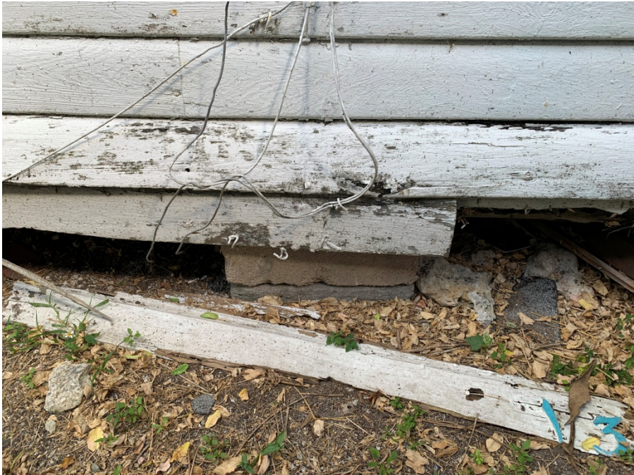
Picture #8 The house is on a crawl space supported by block pedestal without any structural connection
