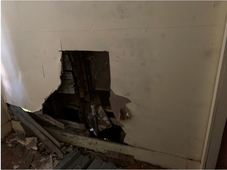
Picture #7 Wood partition rotten inside the house.
