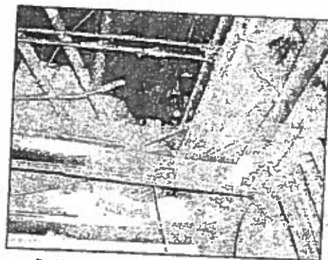
PHOTO #30 FIRST FLOOR ELECTRICAL ROOM PROVIDE CEILING AT THIS ROOM
