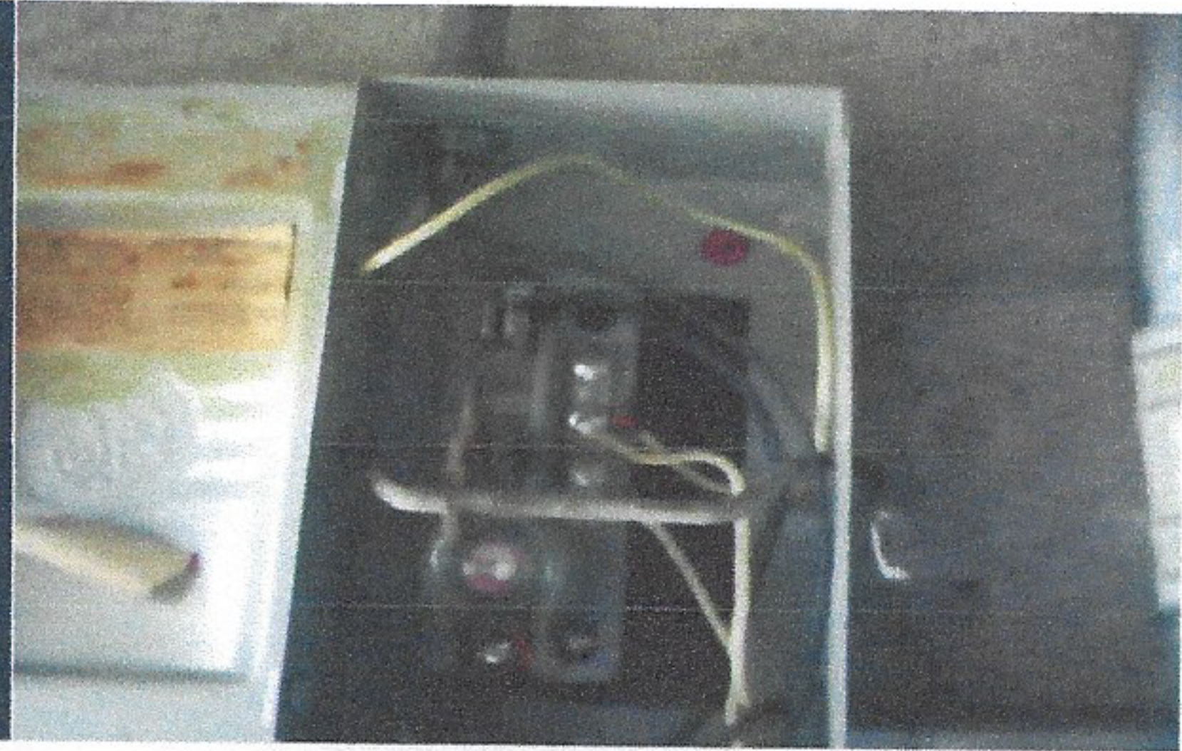
4800 Cab Light Sub.jpegAligned Visual Image
