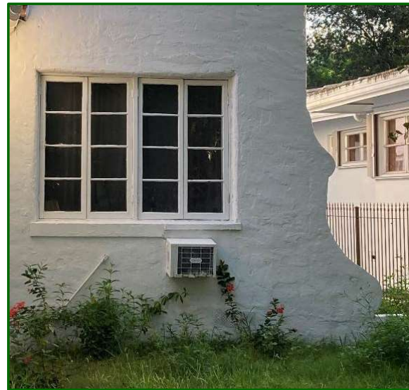
Figure 15: Front (South) Façade, sill cut to accommodate air-conditioning unit, 2021
