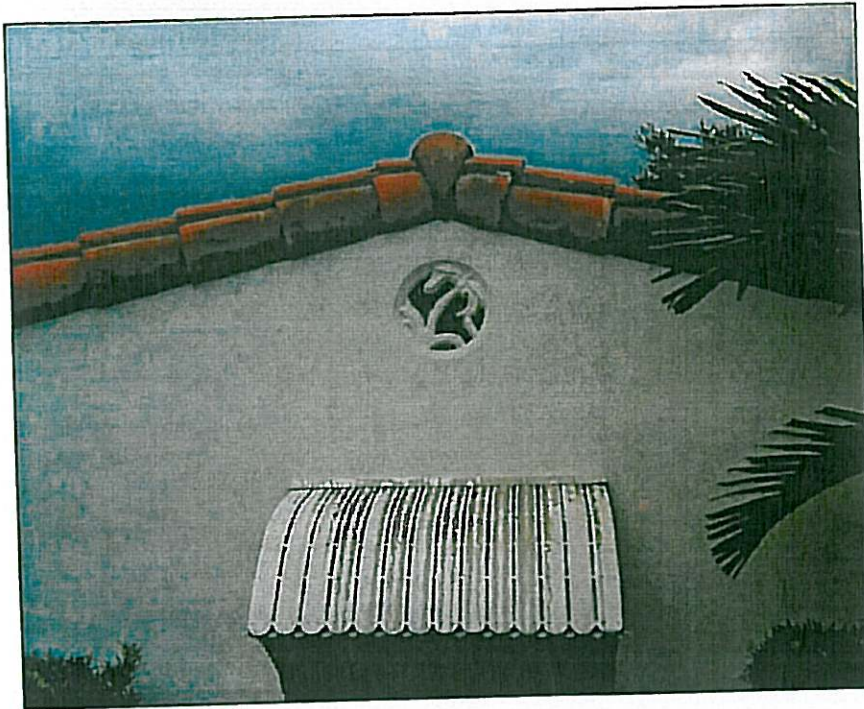
Photograph 17: Detail of Concrete Vent at 317 Malaga Avenue. Photograph Taken by Janus Research, 1999.
