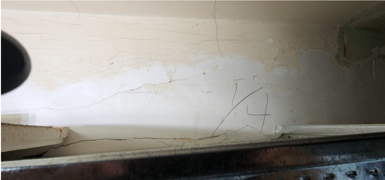
PHOTOGRAPH 40 - EXAMPLE OF CRACKING IN 3 RD FLOOR CITY ATTORNEY'S OFFICE
