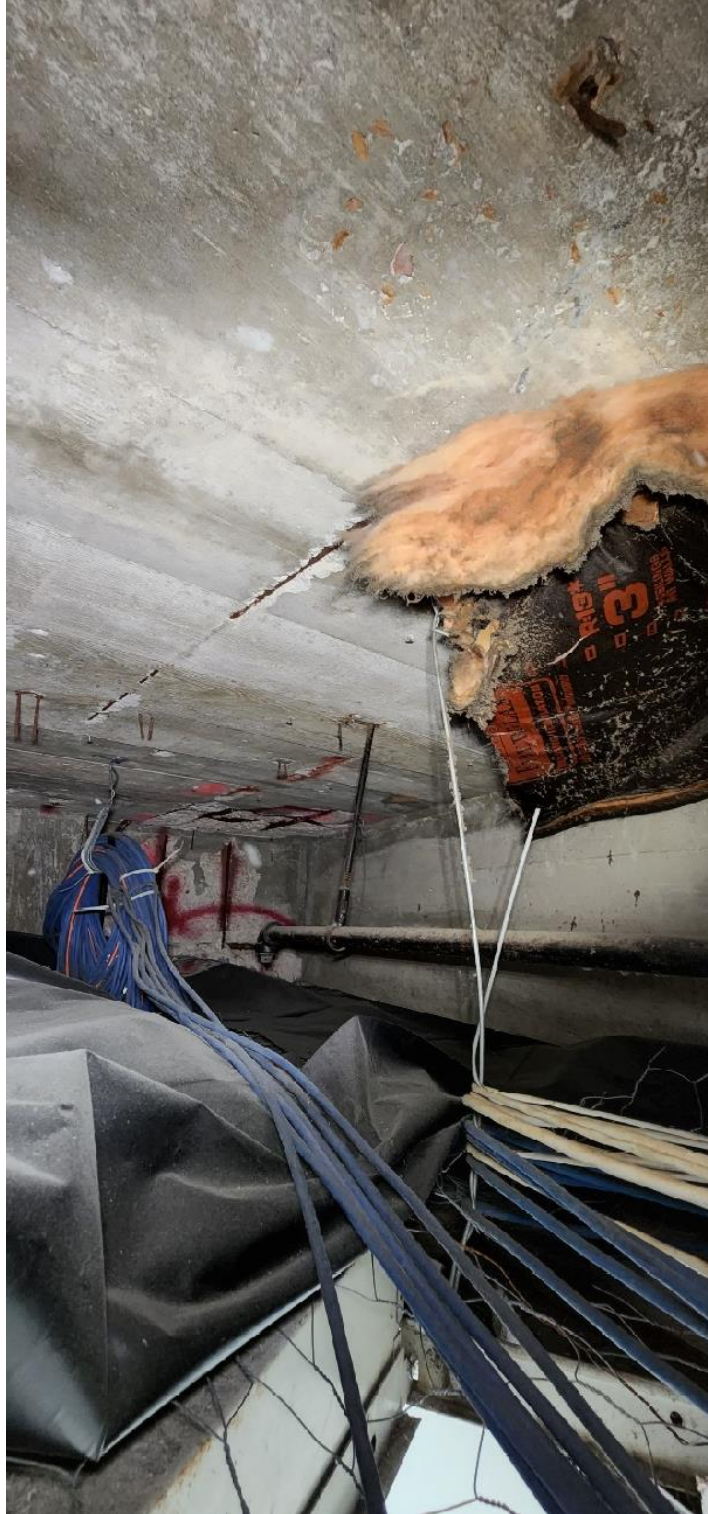
PHOTOGRAPH 7 - EXAMPLE OF SPALLING AT EXTERIOR TIE BEAM AND SLAB ABOVE FINANCE DEPARTMENT
