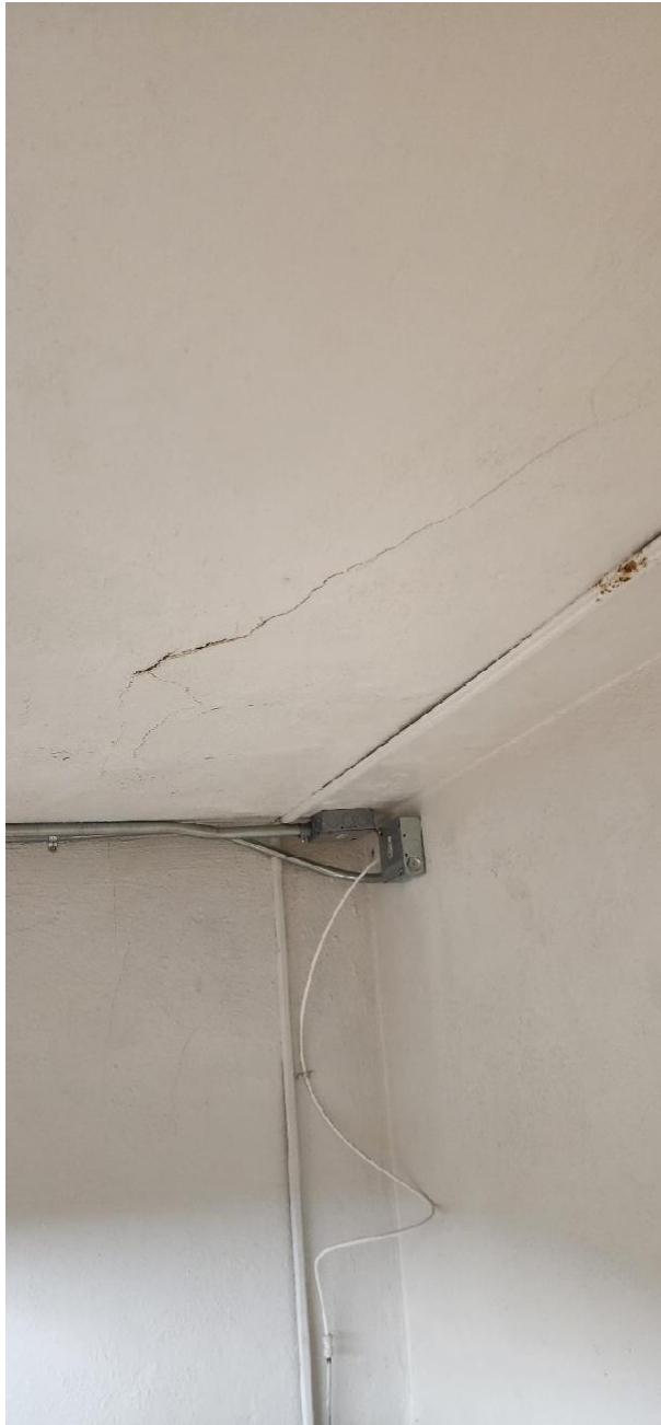
PHOTOGRAPH 16 – SPALLING IN CEILING AND WALL CRACKS AT HISTORICAL SAFE IN CITY MANAGER'S DEPARTMENT
