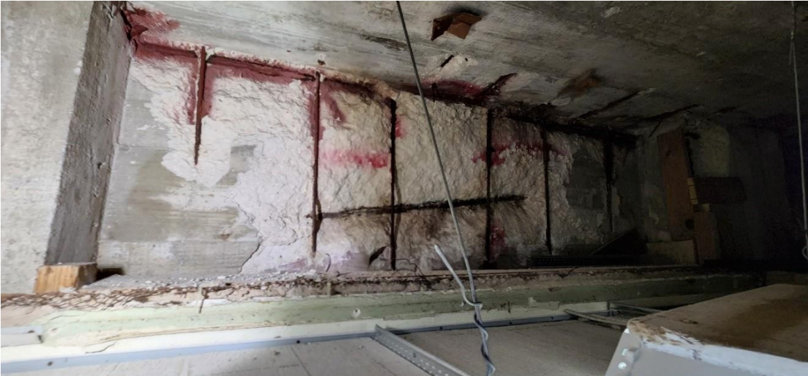
PHOTOGRAPH 13 - SPALLING AT EXTERIOR BEAM ABOVE CITY MANAGER'S CEILING
