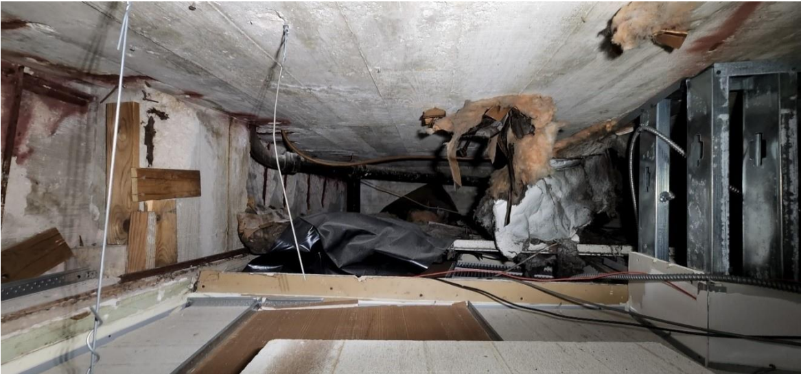
PHOTOGRAPH 14 - SPALLING AT EXTERIOR BEAM ABOVE CITY MANAGER'S CEILING
