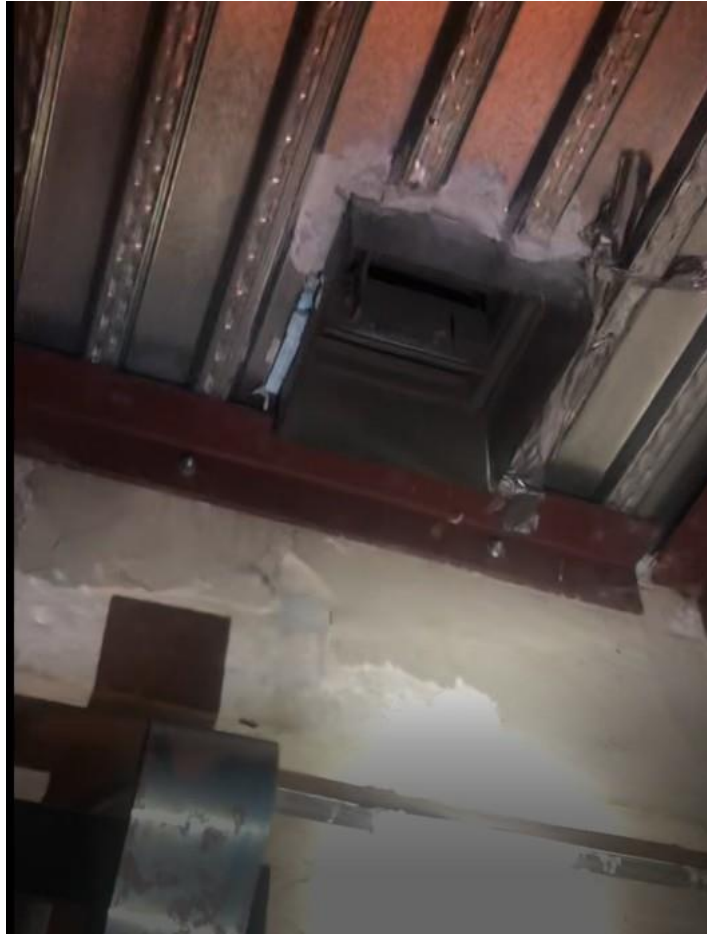
PHOTOGRAPH 45 - EXAMPLE OF SPALLING AT ELEVATOR CHASE WALLS
