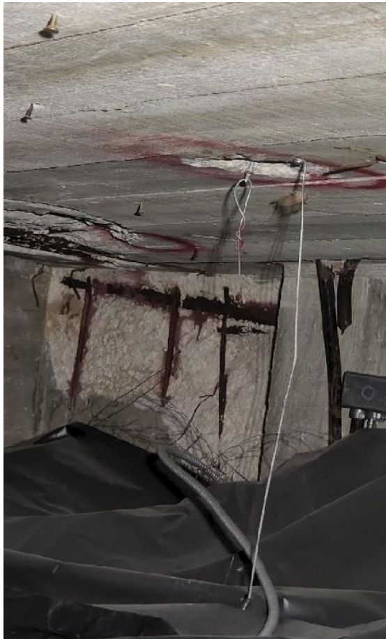
PHOTOGRAPH 6 - EXAMPLE OF SPALLING AT EXTERIOR TIE BEAM ABOVE FINANCE DEPARTMENT
