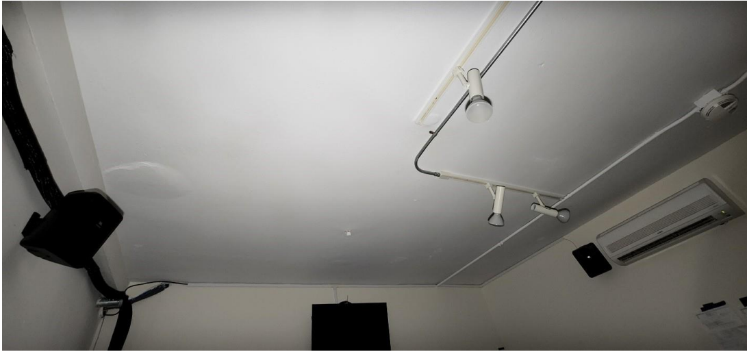
PHOTOGRAPH 38 - EXAMPLE OF CEILING SPALL AT MEDIA CONTROL ROOM
