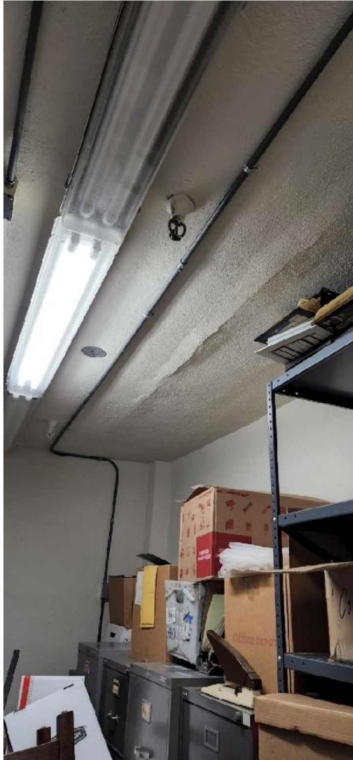
PHOTOGRAPH 48 - EXAMPLE OF SPALLING IN MICROFILM DEPARTMENT.
