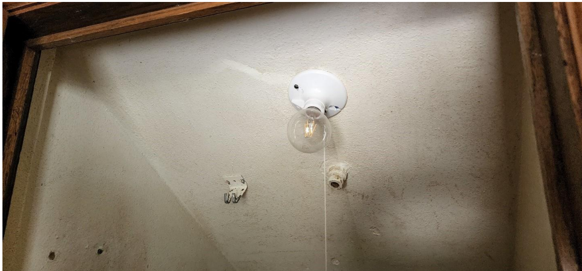
PHOTOGRAPH 25 - EXAMPLE OF SPALL UNDER AUXILIARY STAIRWAY
