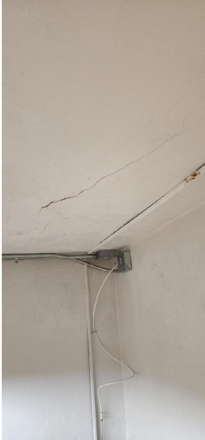
PHOTOGRAPH 16 - SPALLING CEILING AND WALL CRACKS OF HISTORICAL SAFE IN
