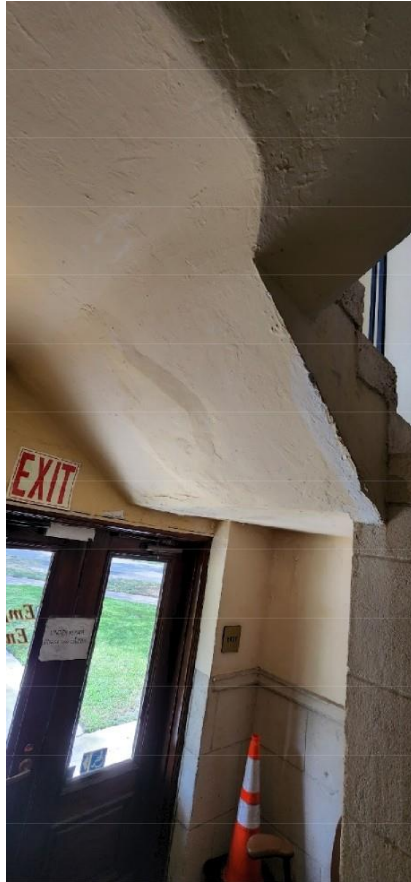
PHOTOGRAPH 1 - BULGING SPALL AT AUXILIARY STAIRCASE
