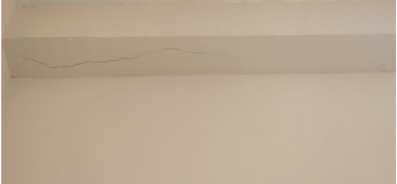
PHOTOGRAPH 17 - SPALLING AT BEAM IN CITY MANAGER'S OFFICE HISTORIC SAFE
