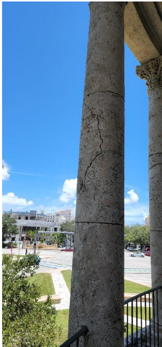
PHOTOGRAPH 32 - EXAMPLE OF SPALLING OF CLADDING AT EXTERIOR COLUMN
