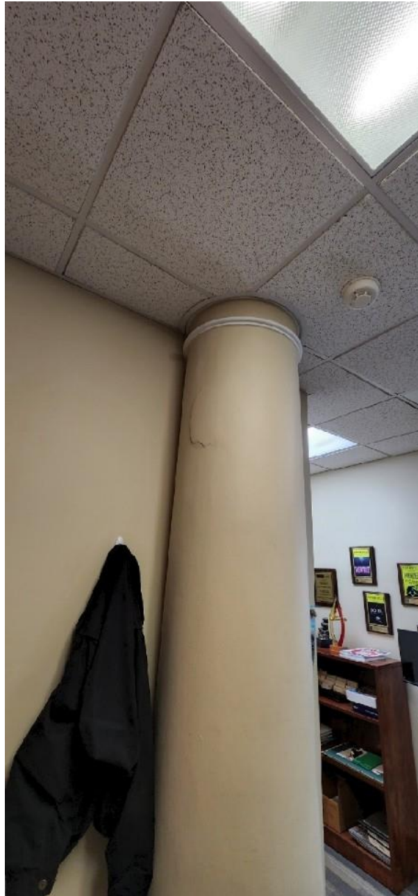
PHOTOGRAPH 11 - SPALLING AT CONCRETE COLUMN IN CITY MANAGER'S DEPARTMENT
