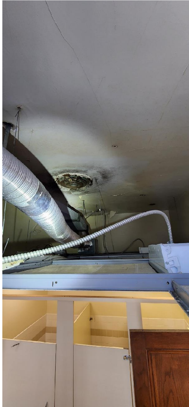
PHOTOGRAPH 47 - EXAMPLE OF EFFLORESCENCE AND CRACKING ABOVE CEILING IN WOMEN'S RESTROOM
