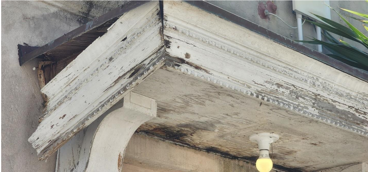
PHOTOGRAPH 66 - EXTERIOR CANOPY ROOF DETERIORATION ABOVE DOORWAYS AROUND ANNEX
