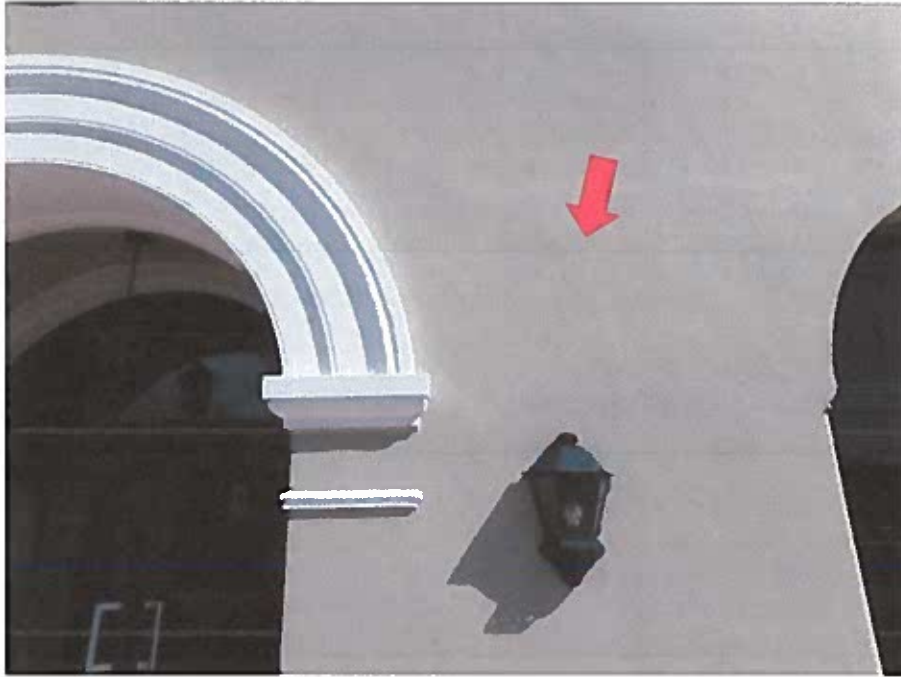
Patching observed at exterior wall
