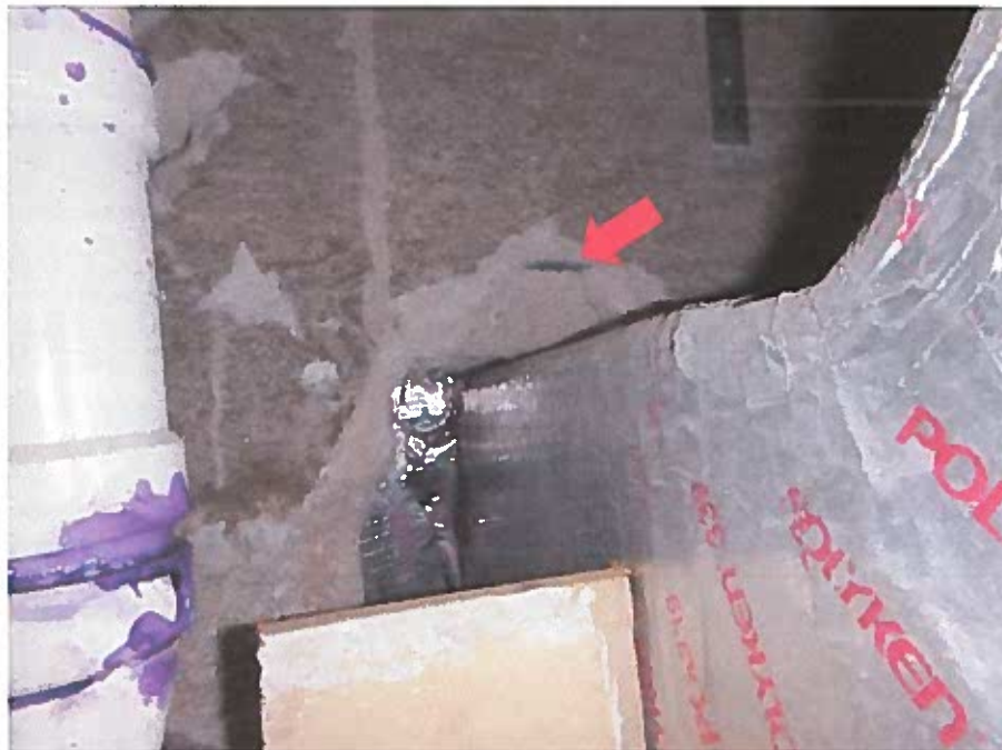
Overview of duct penetration with exposed reinforcement
