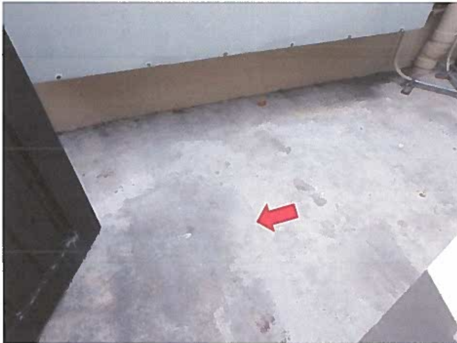
Hairline crack at A/C equipment slab
