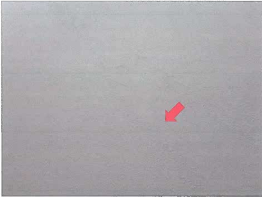
Close-up of patch with hairline crack
