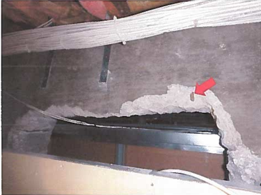
Overview of concrete beam with opening below and exposed reinforcement
