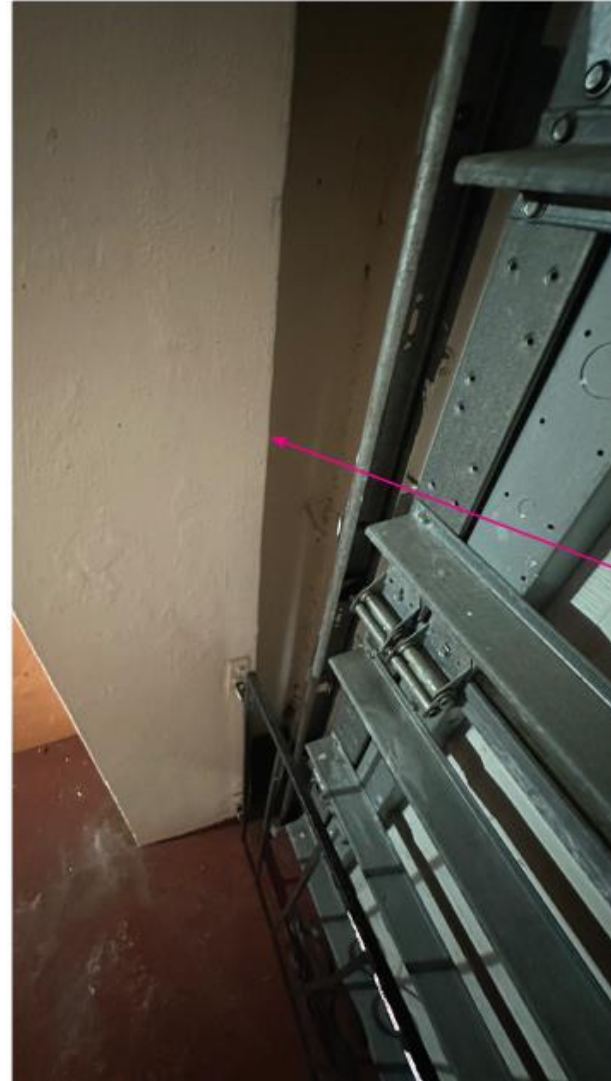
New column and wall tied into original column with rebar and cannot be separated without extensive cutting, reconstruction, and cost.
