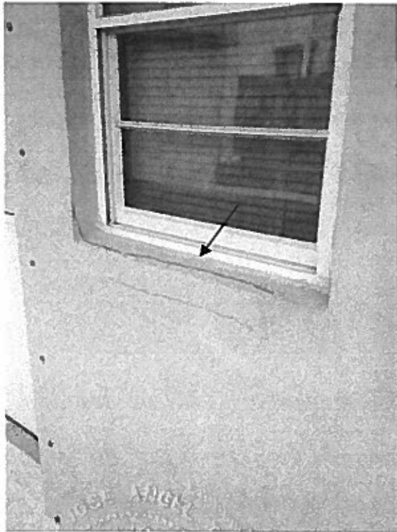
Photograph No. 4 (typical spalling at window sill)
