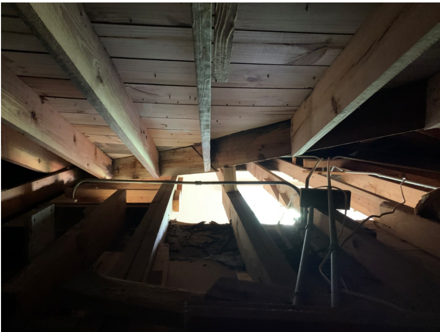
Picture #10 Ridge joist broken.
