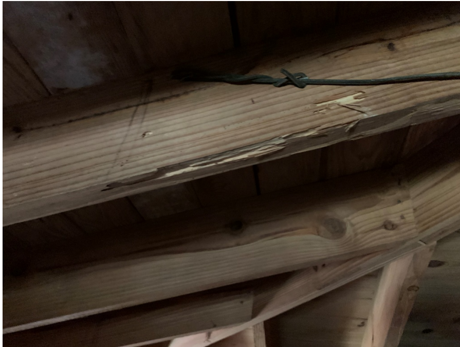
Picture 3 Roof joists damaged by termites.
