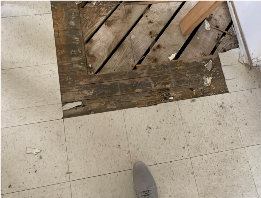
Picture #9 Wood floor damaged by termites.
