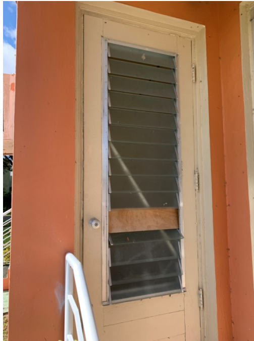
Picture #7 Exterior door very damaged
