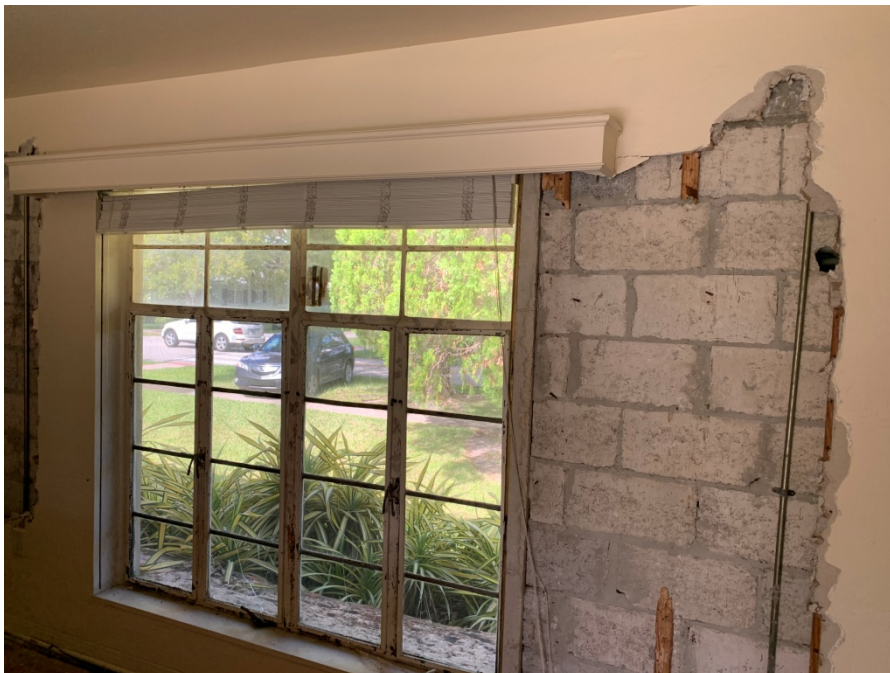
Picture #8 Front widow, very damaged
