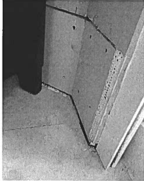
Unit 507 Master suite – Drywall that was affected for water intrusion was being replaced.
