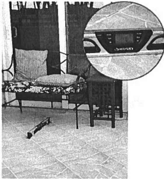
Unit 507 Master suite – No slope in the terrace pavers in front of the sliding door.
