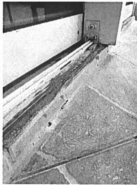
Unit 507 Master suite – Sealant between the pavers and the door threshold is de-bonded, has bubbles, is not covering the joint.
