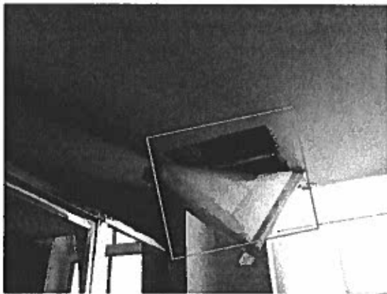
Unit 1105 Master Bathroom – removed ceiling where it was water stained.
