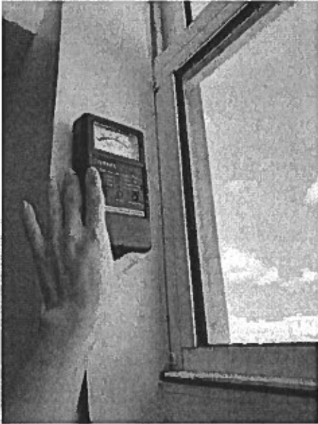
Unit 1105 Master Bathroom – window did not have any sign of moisture or water stain.
