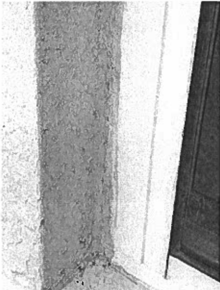
Unit 507 Master suite – Hairline cracks in the window perimeter sealant.
