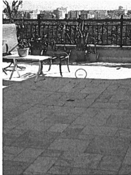
Above Unit 1505 Master Bedroom – farther drain (in the terrace of PH-2) located above the wall between the door and the walk-in closet.
