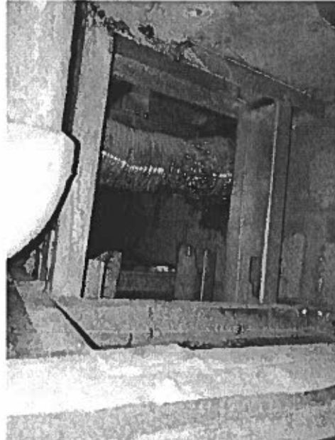
Unit 1105 Master Bathroom – vent duct and pipe above the removed ceiling. Corroded ceiling frame.
