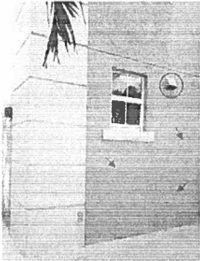
Unit 505 Master bathroom – vent exhaust close to the bathroom window and above the ceiling. Hairline cracks visible that were repaired in 2016.
