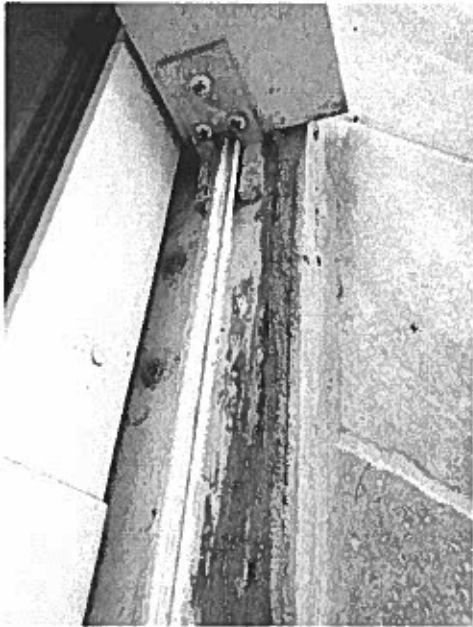
Unit 507 Master suite – Crack between sliding door threshold and flooring
