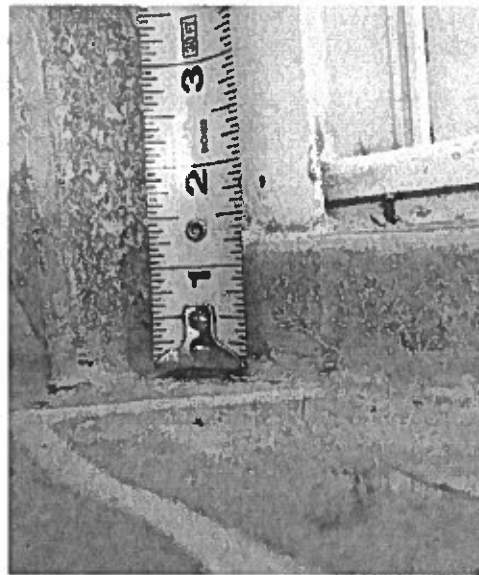
Unit 507 Master suite – Sealant between the pavers and the wall and door threshold is de-bonded and has bubbles.
