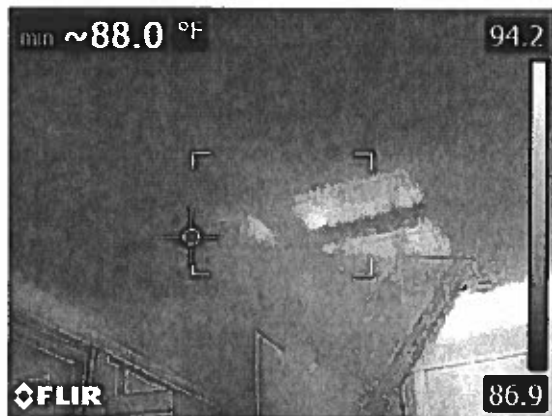
Unit 1105 Master Bathroom – thermo-camera photo where no water intrusion is shown.
