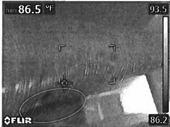
Unit 1105 Master Bathroom – thermo-camera photo where the vent duct located to the left and above the removed affected ceiling seem to have some moisture in the dark spot depicted above.
