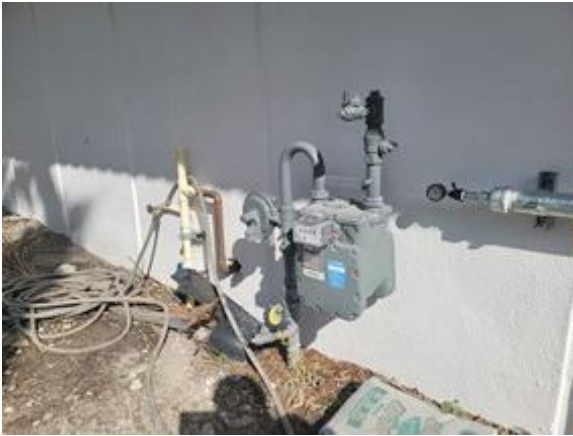
Subject gas meter
