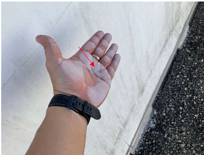
Photo # 19. Paint Chalking at exterior wall.
