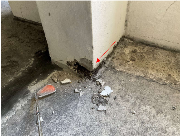
Photo # 13. Concrete spalling at column of parking garage.
