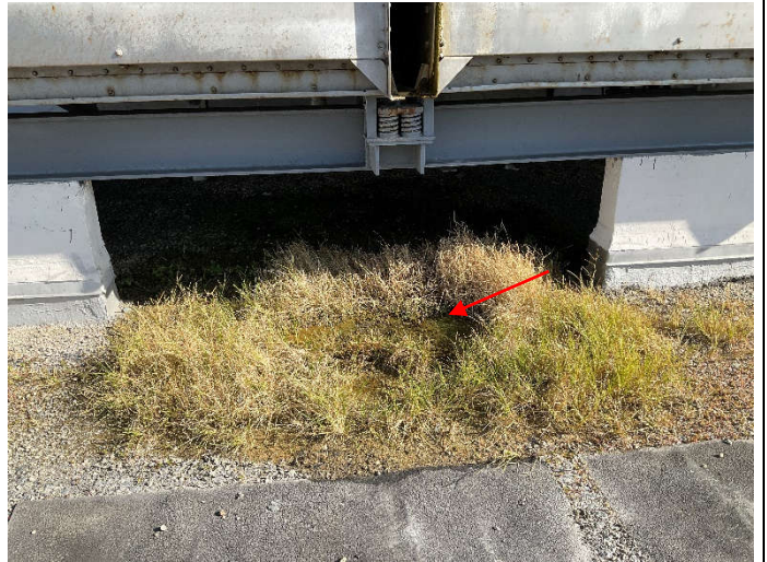
Photo # 38. Ponding water and biological growth at roof under cooling tower.
