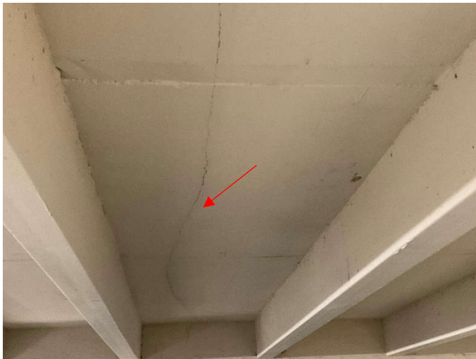
Photo # 27. Concrete crack at ceiling of parking garage.
