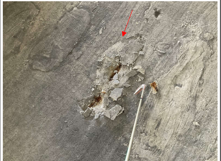
Photo # 8. Concrete spalling at parking garage.
