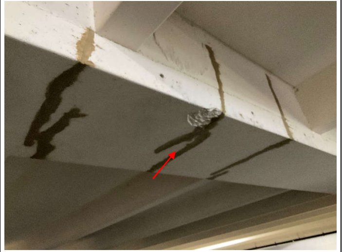
Photo # 30. Previously repaired areas at beam of parking garage.
