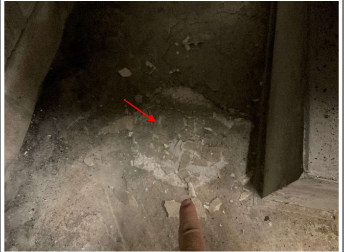
Photo # 6. Concrete spalling at roof (Generator Room).
