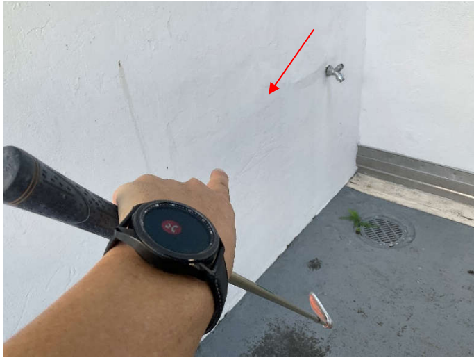
Photo # 21. Stucco delaminating at parking garage.
