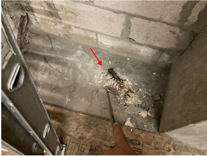
Photo # 5. Concrete spalling and exposed corroded rebar at roof (Generator Room).
