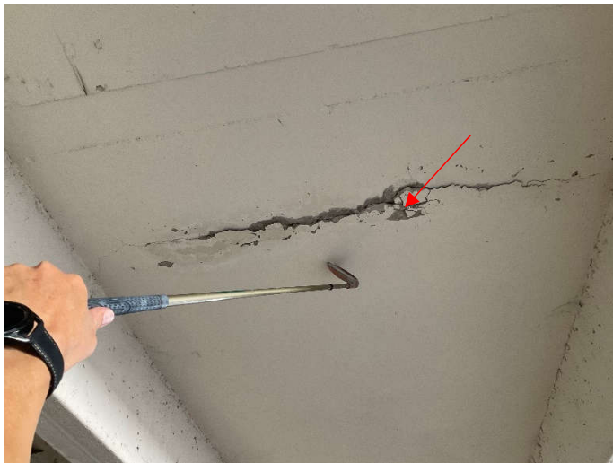
Photo # 11. Concrete spalling at ceiling of parking garage.
