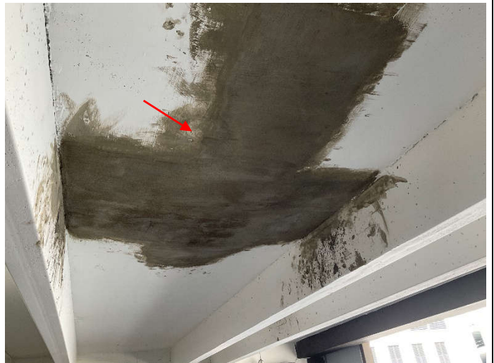
Photo # 28. Previously patched area at parking garage ceiling.
