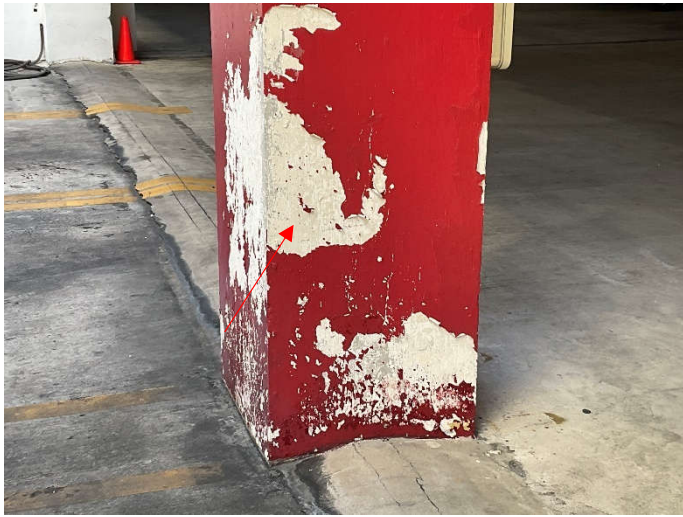
Photo # 17. Peeling paint at base of column.
