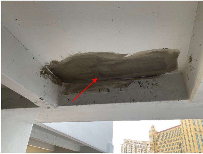
Photo # 29. Previously patched area at parking garage ceiling.
