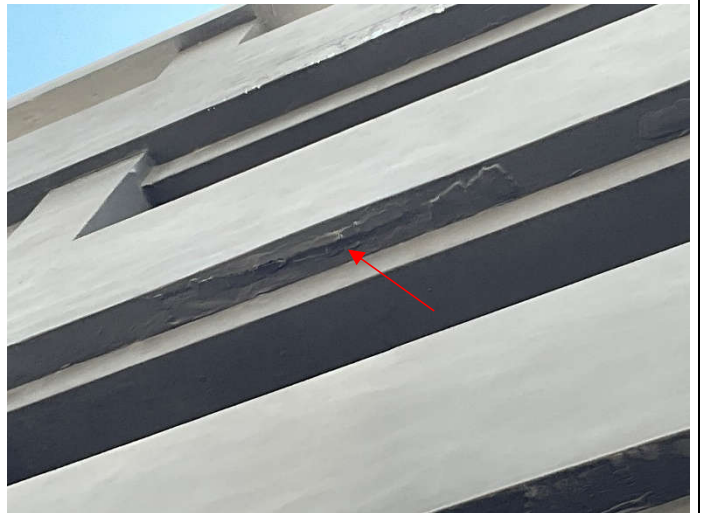
Photo # 16. Concrete spalling at slab edge of parking garage.
