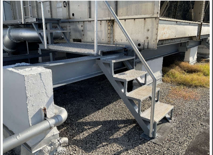
Photo # 36. Cooling tower supports.
