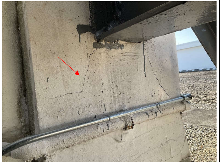
Photo # 24. Delaminated/de-bonded stucco at roof.
