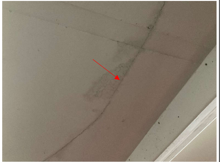
Photo # 26. Concrete crack at ceiling of parking garage.
