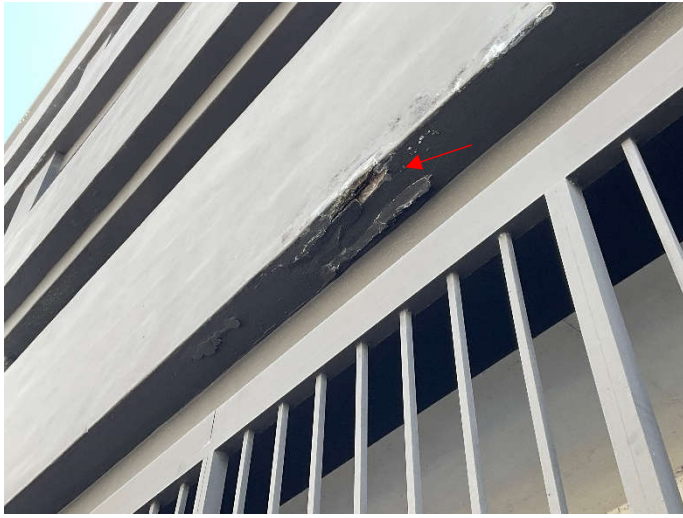
Photo # 25. Concrete spalling at slab edge of parking garage.
