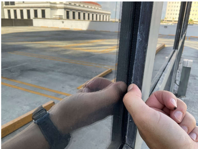
Photo # 51. Curtain wall sealant exhibiting typical dry condition.
