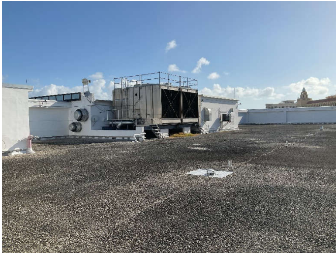
Photo # 33. Cooling tower located at roof.
