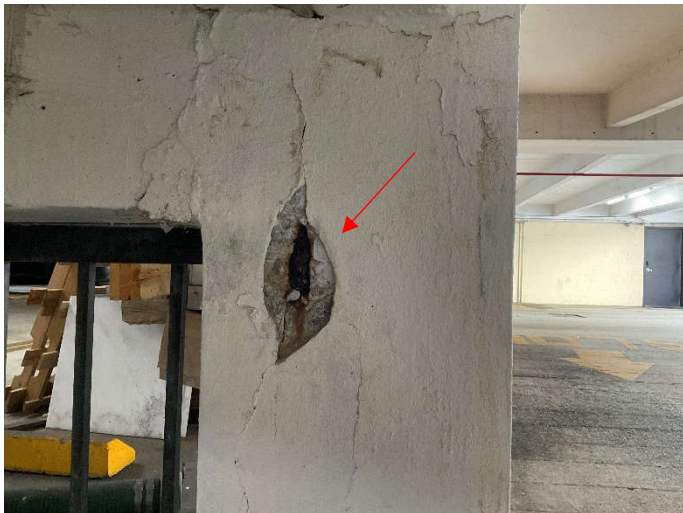
Photo # 15. Concrete spalling at column of parking garage.
