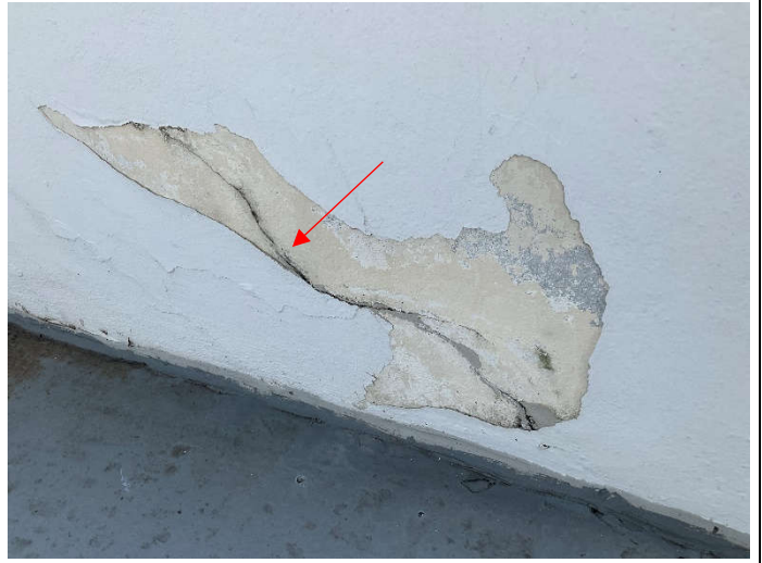
Photo # 22. Stucco crack at parking garage.
