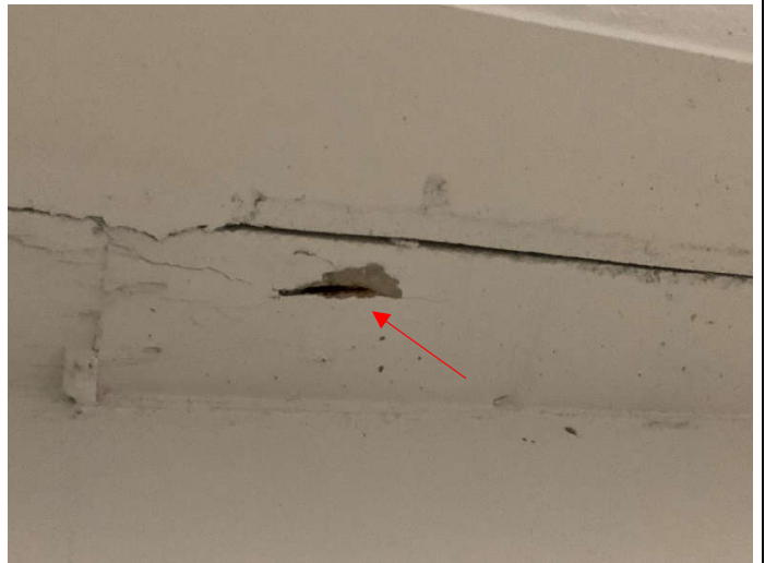
Photo # 12. Concrete spalling at ceiling of parking garage.
