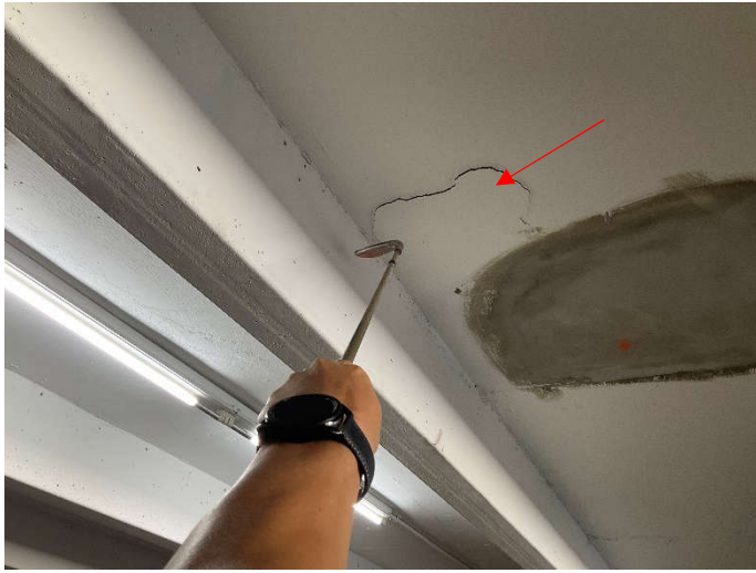
Photo # 9. Concrete spalling at ceiling of parking garage.
