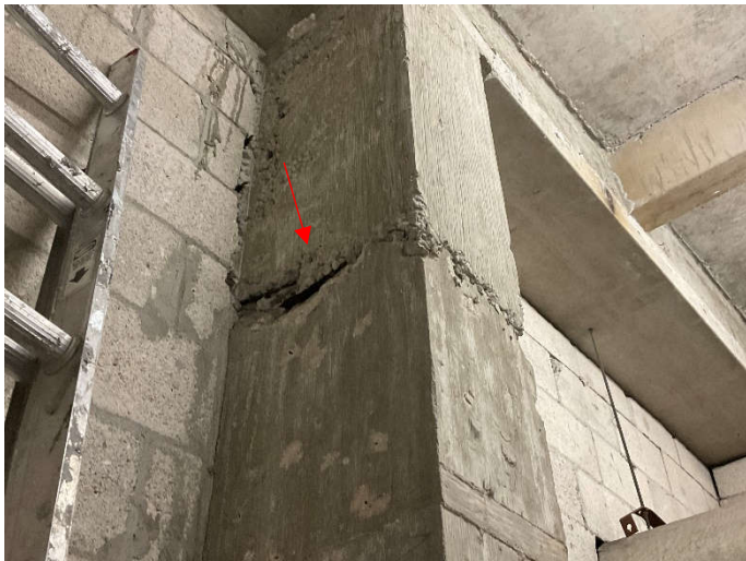
Photo # 7. Concrete damage at column of Generator Room.
