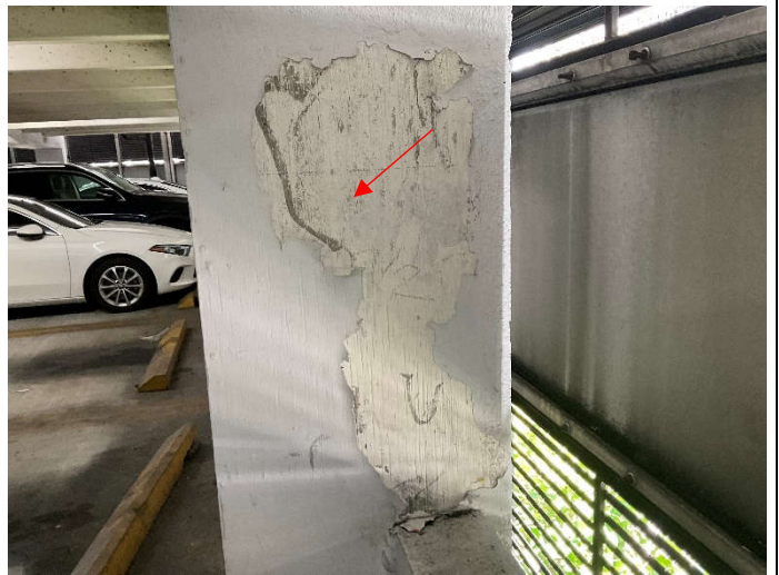
Photo # 20. Paint peeling at column.
