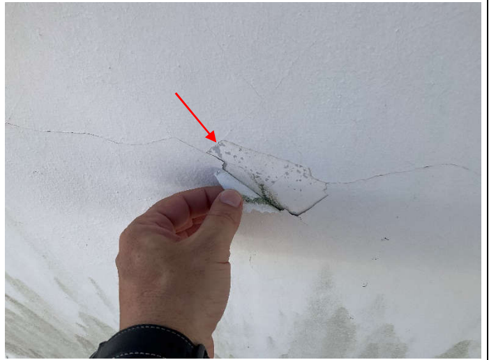
Photo # 18. Paint peeling at roof parapet wall.
