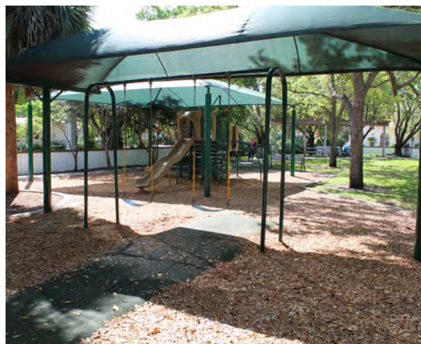
Need for playground surface improvements at Sunrise Harbor Park
