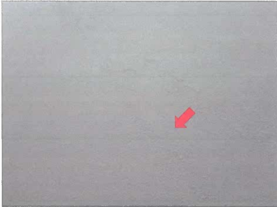
Close-up of patch with hairline crack
