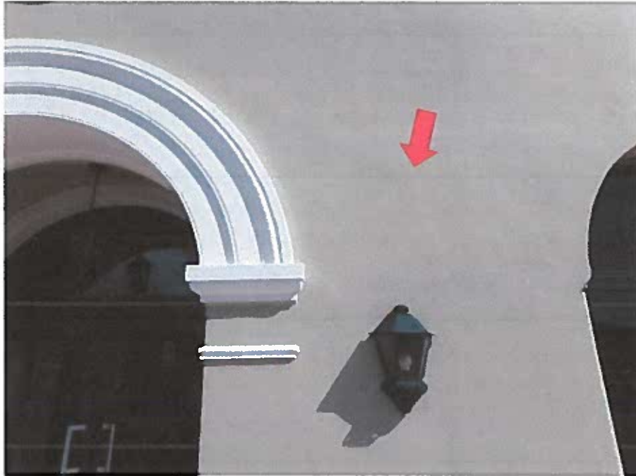
Patching observed at exterior wall
