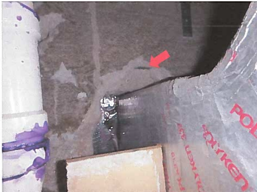
Overview of duct penetration with exposed reinforcement
