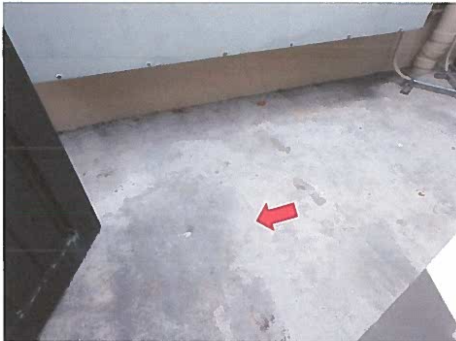
Hairline crack at A/C equipment slab
