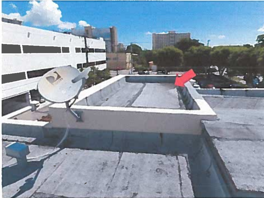
Overview of rooftop over stairwell with water accumulation beneath roofing
