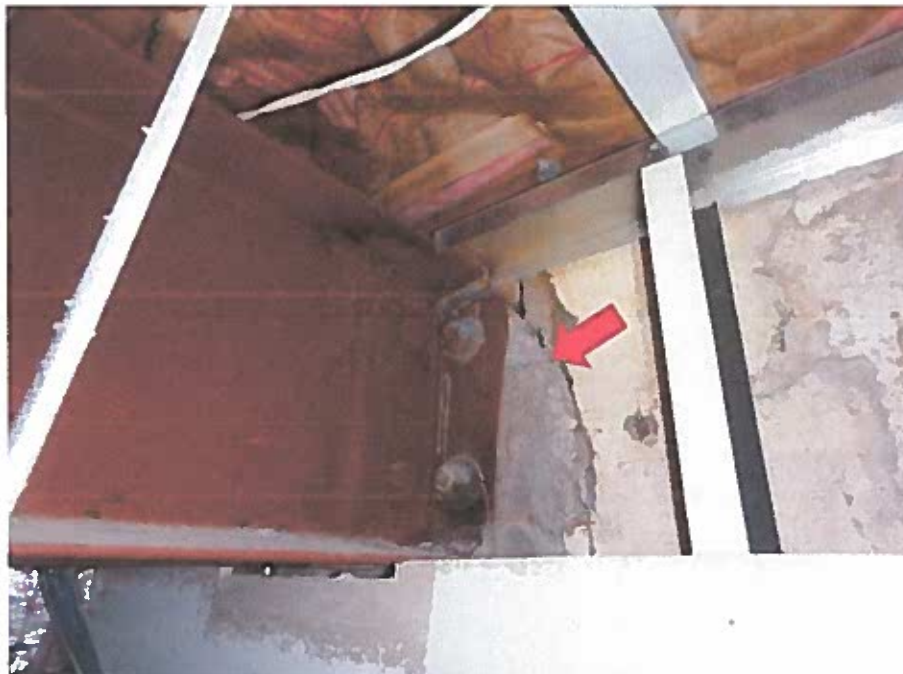
Concrete cracking near bolt location at steel beam clip angle connection
