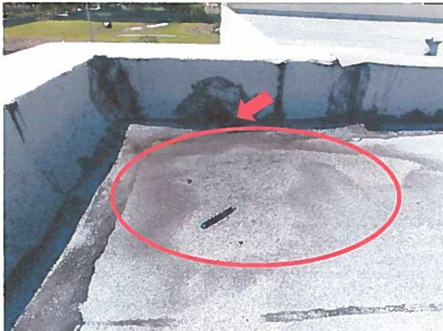
Water accumulating beneath roofing over stairwell and single scupper
