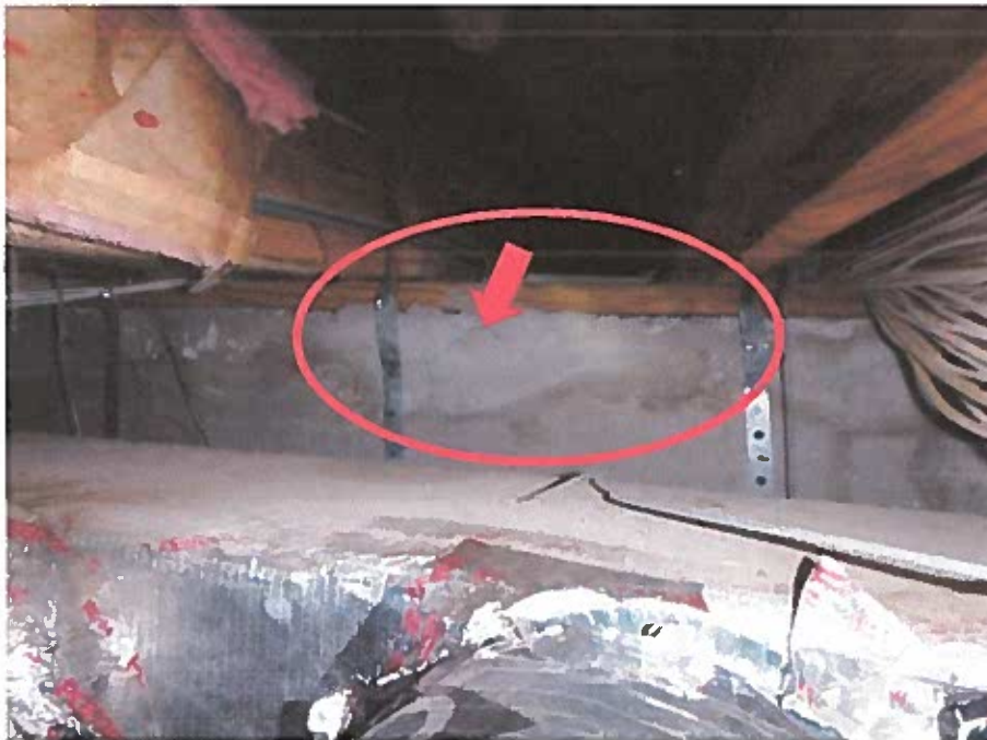
Cracking along concrete beam at previous repair location
