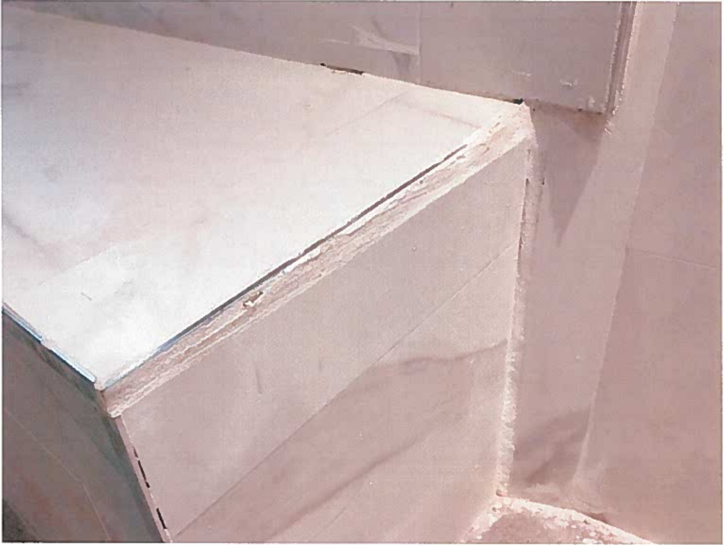
Master bathroom shower bench. Note poor workmanship of tiles and stainless steel insert.
