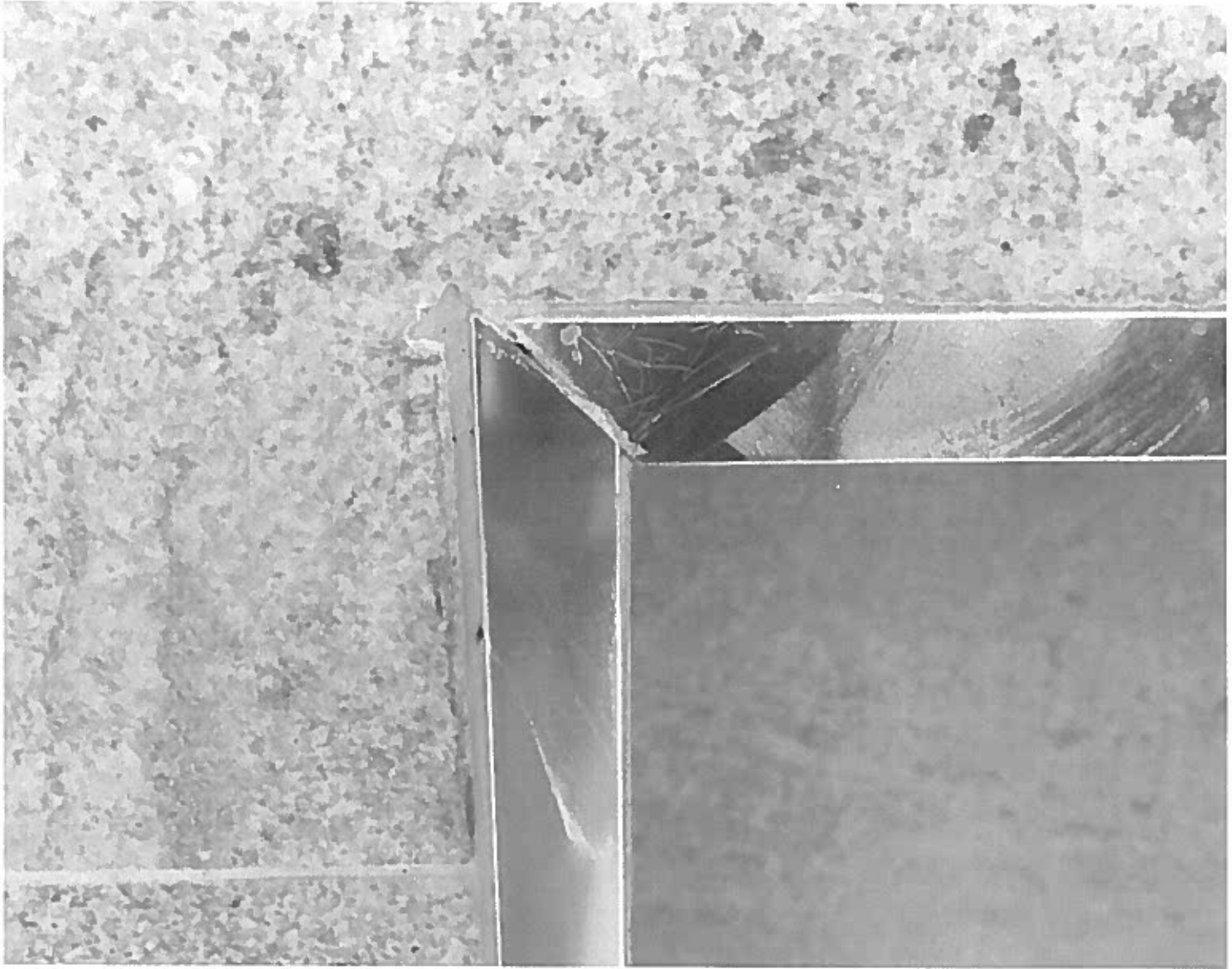
Poorly cut mitered joint of stainless steel insert. Most mitered joints are not flush and many have sharp edges.
