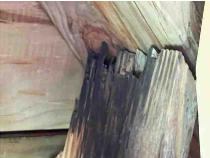
Wood Rot in Trusses
