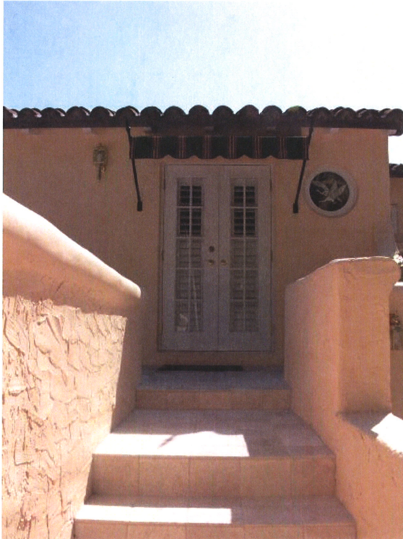
PHOTO #12—Northwest (Front Façade) Partial Elevation at Garage Roof Terrace Stairs and Doors
