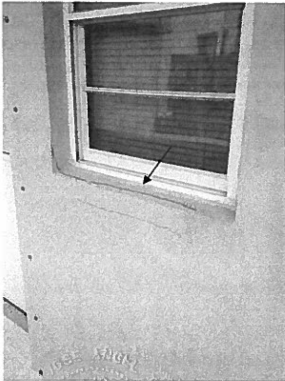
Photograph No. 4 (typical spalling at window sill)
