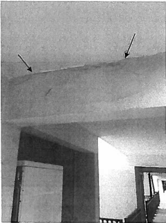
Photograph No. 5 (typical beam spalling)
