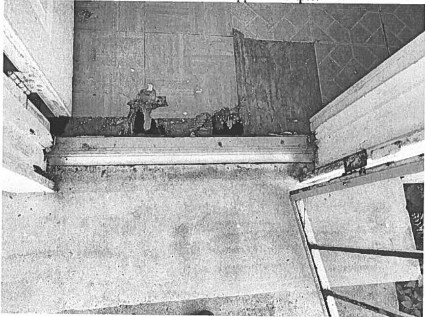
Picture #10 The wood floor is rotten in some areas.
