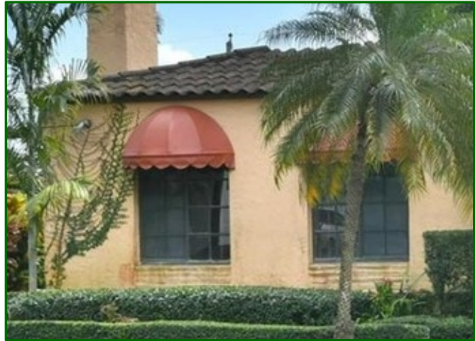
Figure 21: Slump Brick Below Windows, 2019
