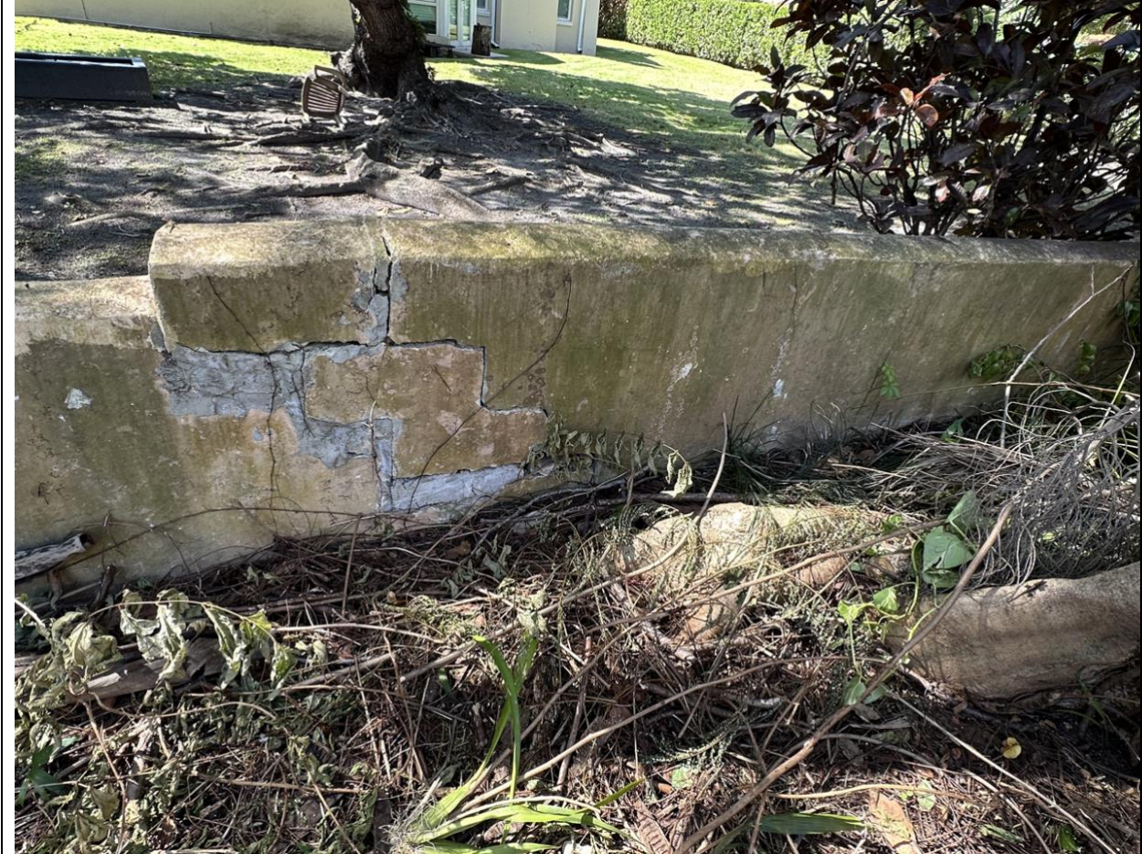
Large buttress root lifting and causing cracking in concrete wall.
