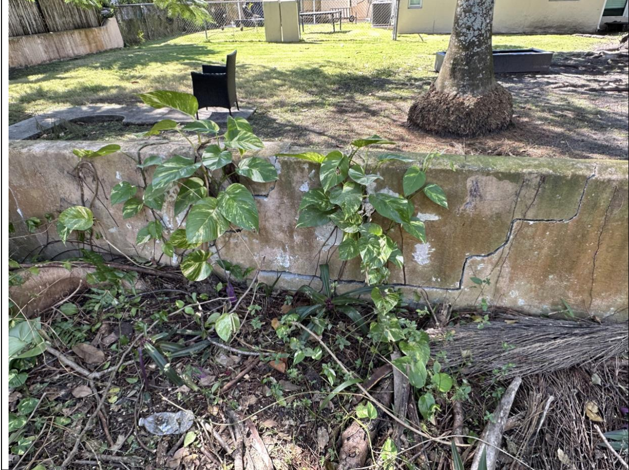
Tree #3, Roots of tree lifting and cracking concrete wall.
