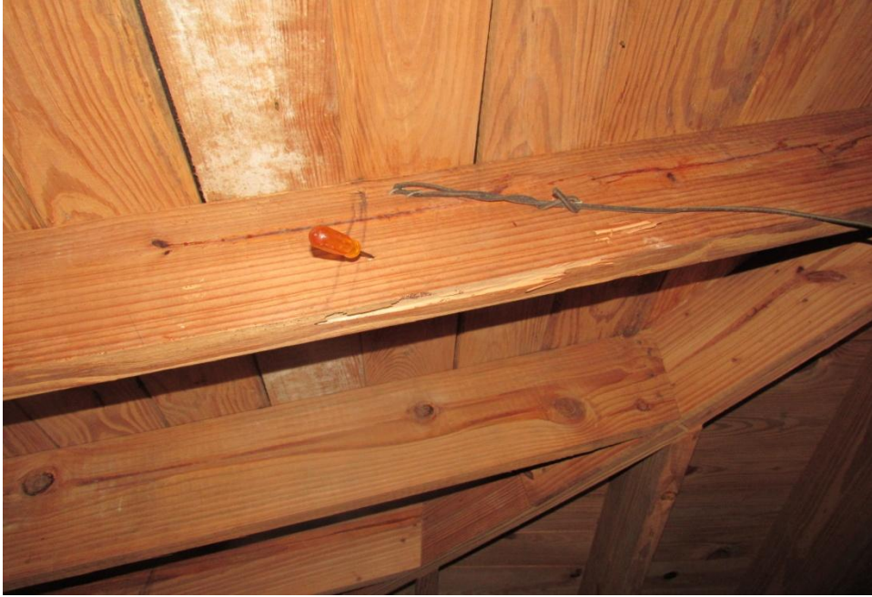
View of distressed roof joist due to termite infestation.
