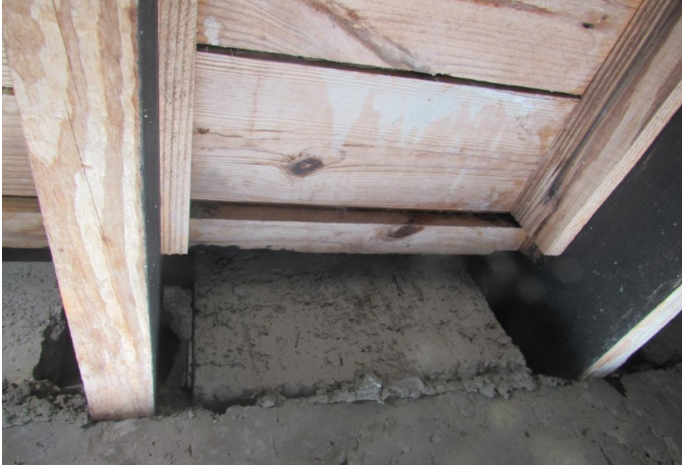
View of subfloor framing lacking structural connection to the foundation system.
