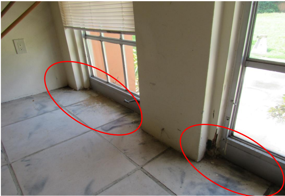
View of termite infestation evidence throughout the residence's interiors
