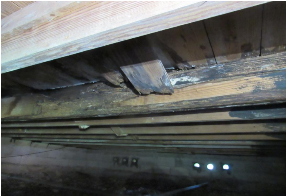
View of distressed (local failure) subfloor planks and joists due to water intrusion.
