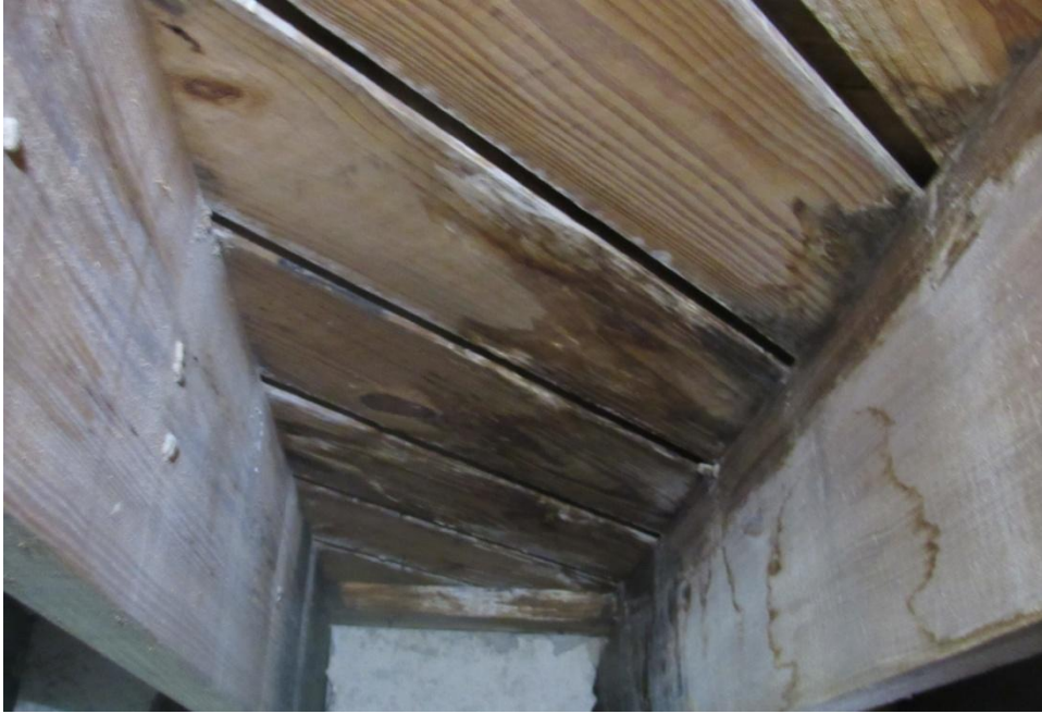
View of distressed subfloor planks and joists due to water intrusion.
