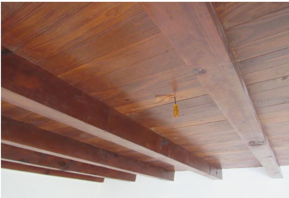
View of distressed roof plank due to termite infestation.
