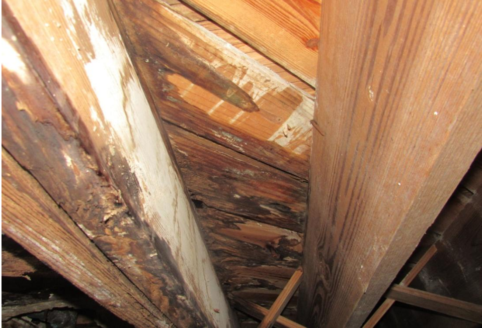
View of distressed (local failure) subfloor planks and joists due to water intrusion.
