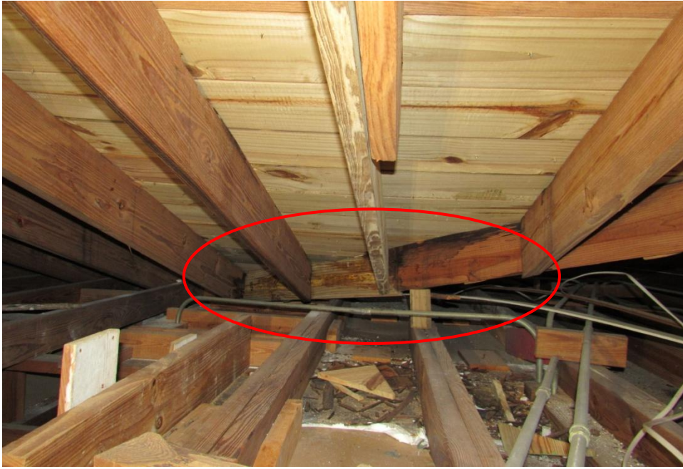
View of distressed rafter (local failure) due to water intrusion.
