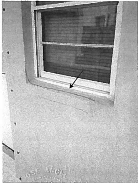
Photograph No. 4 (typical spalling at window sill)
