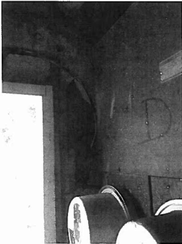
Photograph No. 8 (damage at meter roof door framing)
