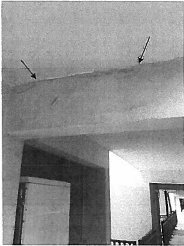
Photograph No. 5 (typical beam spalling)
