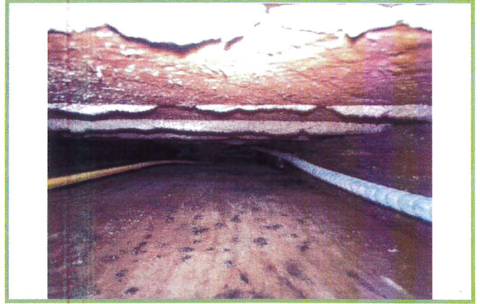
Photograph #8: Bathroom Wall Cavity – Photo depicts SVMG on backside of building material.
