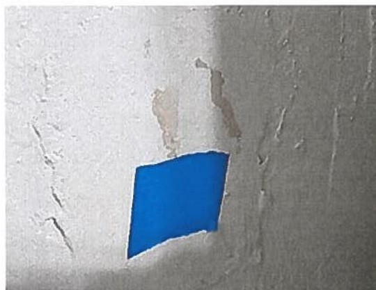
Visible Mold Growth
