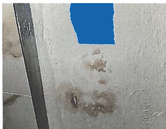
Visible Mold Growth
