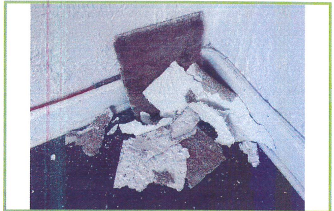
Photograph #2: Living Room West Perimeter Wall – Photo depicts debris (see bottom of Photograph 1) with SVMG on backside of building materials.
