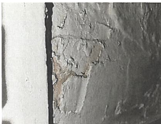
Visible Moisture Stains
