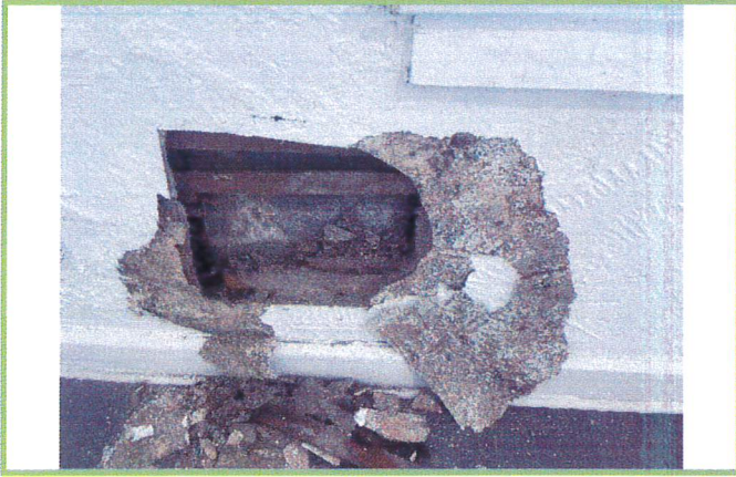
Photograph #7: Bedroom West Perimeter Wall – Photo depicts wall access location and SVMG on backside of building materials.
