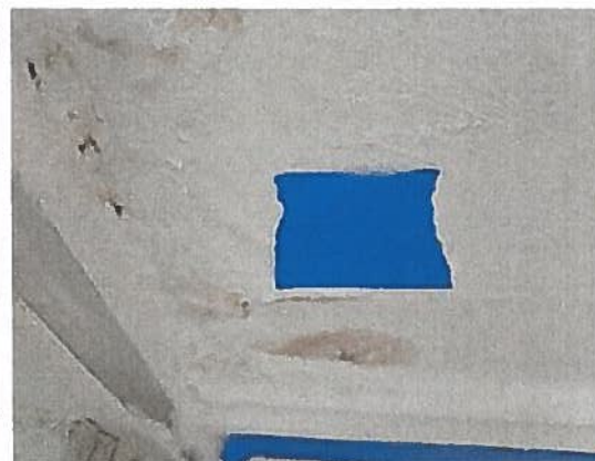
Damage And Mold Growth
