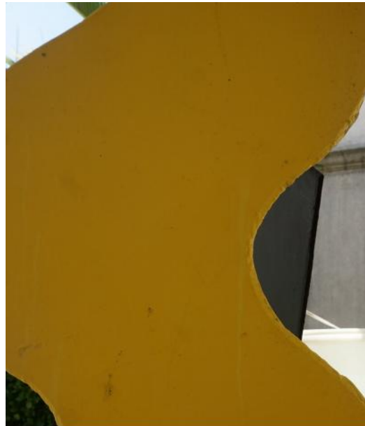
Figure 8. Soiling on yellow piece, typical both sides (photo by EverGreene, February 2021).
