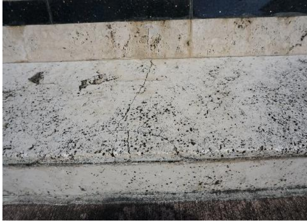
Figure 9. Large fracture in marble step (photo by EverGreene, February 2021).
