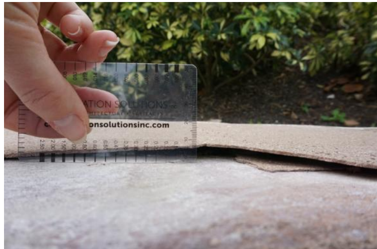
Figure 11. Delamination on platform, 1/2 cm gap (photo by EverGreene, February 2021).
