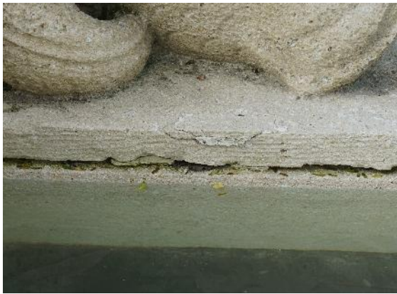
Figure 10. Previously repaired spall on north pegasus (photo by EverGreene, February 2021).
