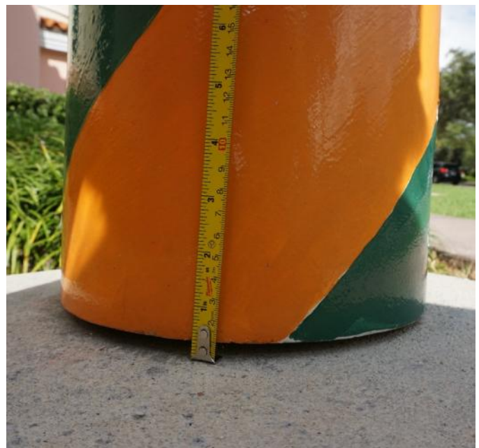
Figure 2. Displacement. (photo by EverGreene, February 2021).
