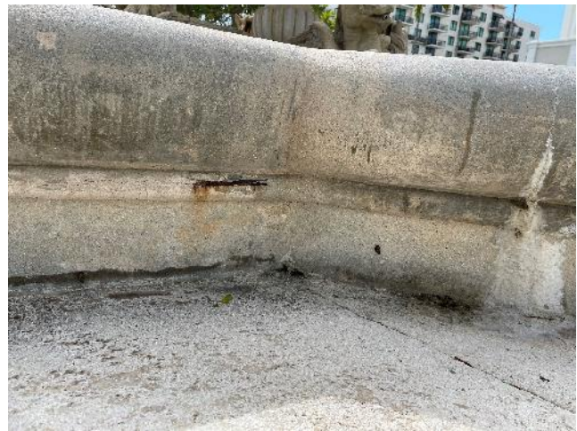
Figure 7. Corroded ferrous metal resulted in damage and loss in concrete (photo by EverGreene, February 2021).
