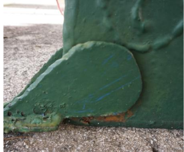
Figure 4. Deterioration on and around the green clamp, blue paint on the surface of the green clamp (photo by EverGreene, February 2021).
