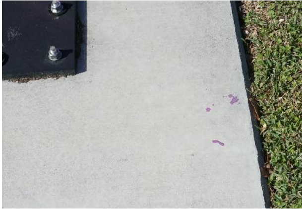
Figure 3. Magenta/purple coating drips on concrete pad (photo by EverGreene, February 2021).
