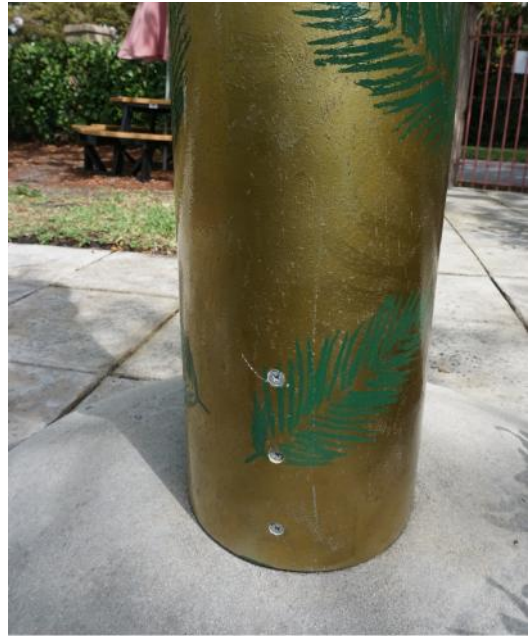
Figure 4. Vertical abrasion on shaft (photo by EverGreene, February 2021).
