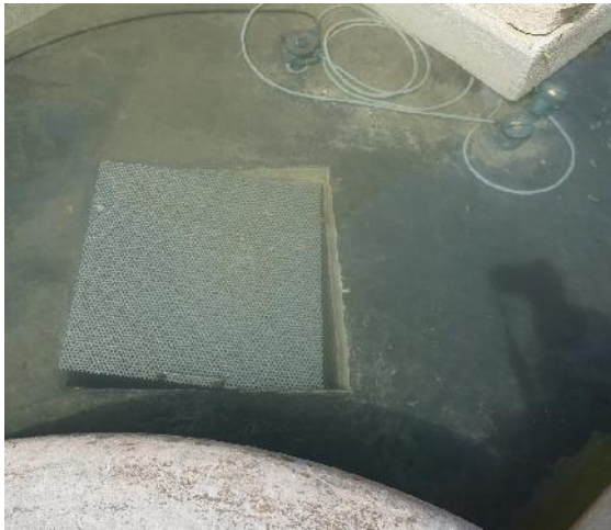
Figure 6. Displaced door (photo by EverGreene, February 2021).
