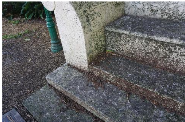
Figure 4. Accumulation of soiling and debris (photo by EverGreene, February 2021).
