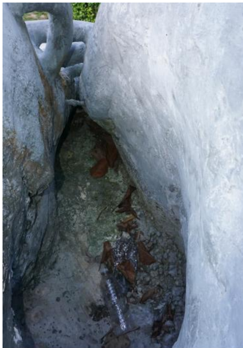
Figure 6. View of inside of south shoe, accumulation of soiling and debris (photo by EverGreene, February 2021).
