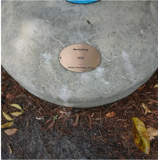
Figure 3. Plaque; network cracking of concrete base (photo by EverGreene, February 2021).
