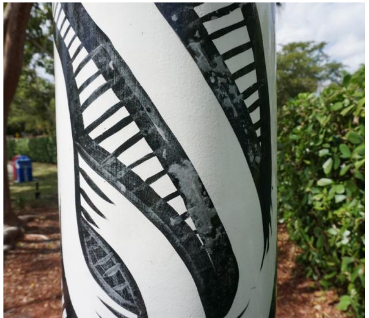
Figure 2. Coating failure (photo by EverGreene, February 2021).
