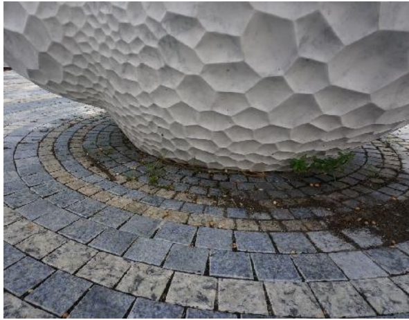
Figure 7. Plant growth in paver joints (photo by EverGreene, February 2021).
