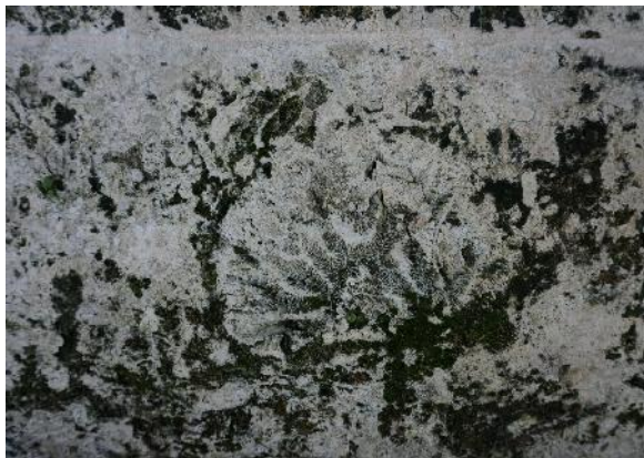
Figure 3. Detail of oolite stone, biological growth (photo by EverGreene, February 2021).
