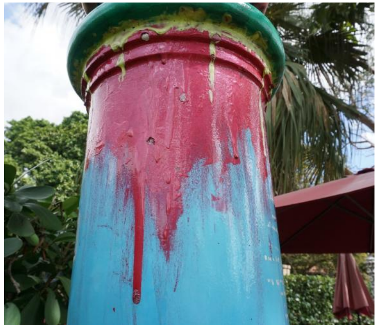
Figure 2. Impasto paint has chipped (photo by EverGreene, February 2021).
