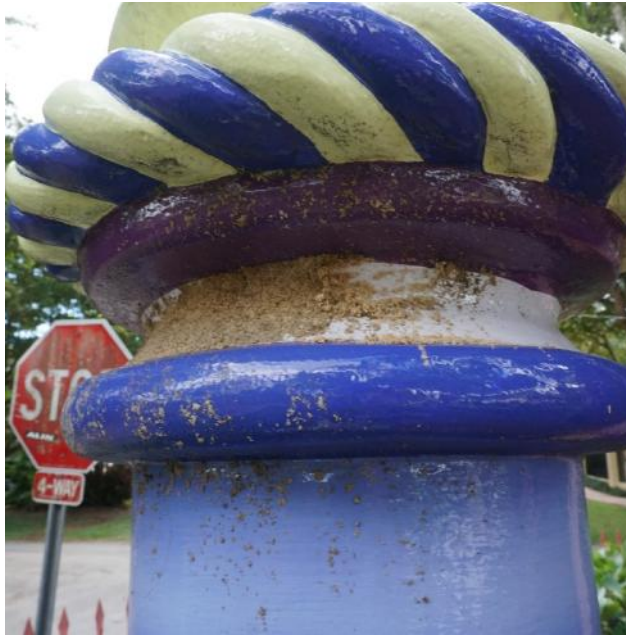
Figure 3. Soiling build-up on capital of Passionflower , possibly from insect activity (photo by EverGreene, February 2021).
