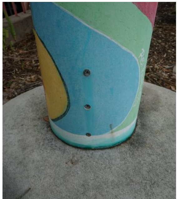
Figure 2. Accumulation of minerals from pool water spray (photo by EverGreene, February 2021).
