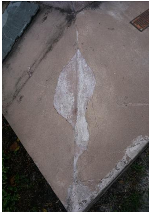
Figure 10. Typical loss of surface of platform (photo by EverGreene, February 2021).
