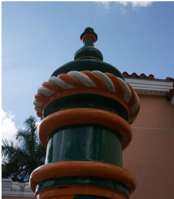
Figure 1. Soiling on underside of capital details (photo by EverGreene, February 2021).
