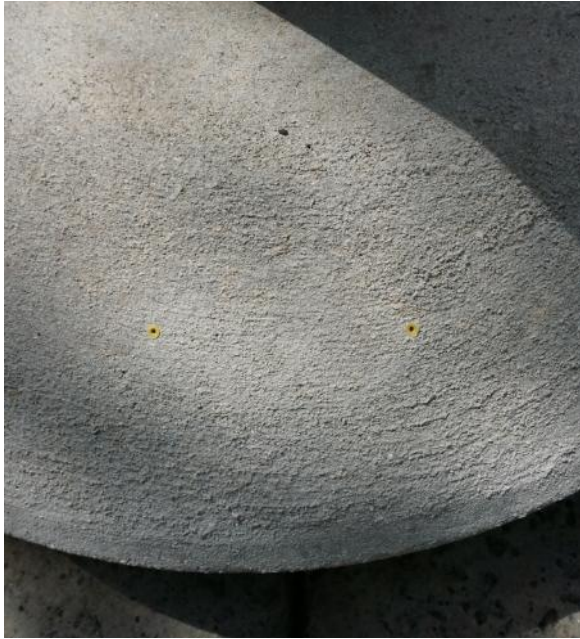
Figure 3. Missing plaque and screws (photo by EverGreene, February 2021).
