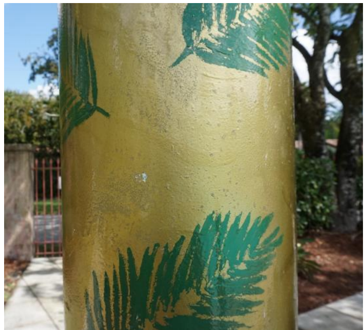
Figure 2. Paint failure/bubbling on shaft (photo by EverGreene, February 2021).
