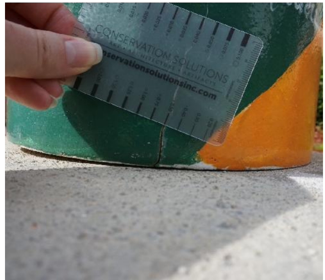
Figure 6. Crack (photo by EverGreene, February 2021).
