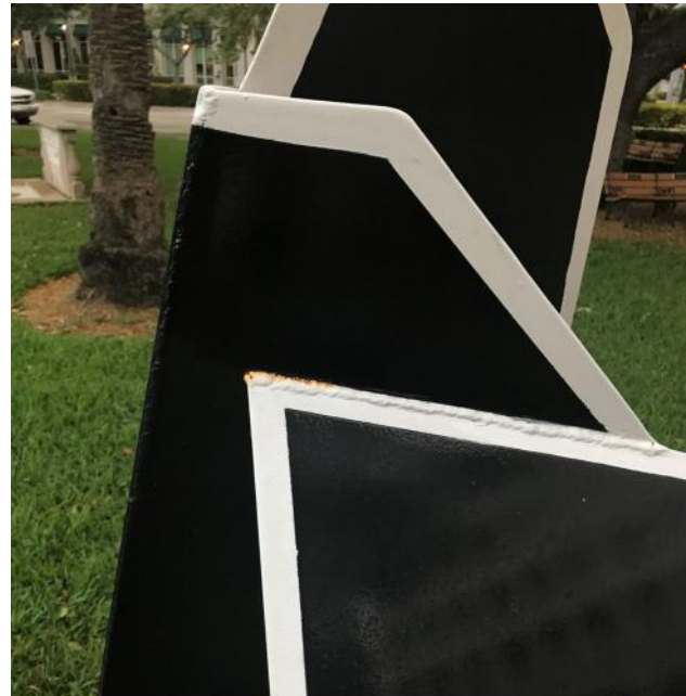
Figure 2. Corrosion on weld (photo by EverGreene, February 2021).
