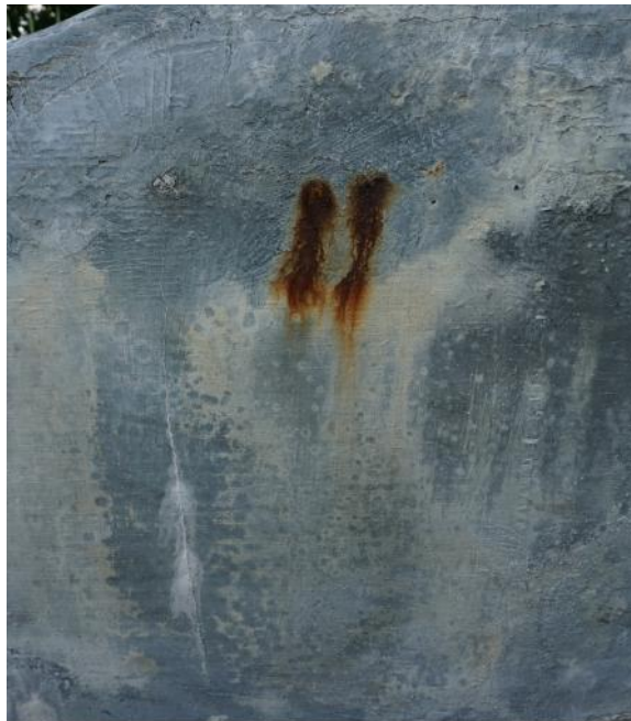
Figure 2. Ferrous corrosion deposits and staining on the bottom of the north shoe (photo by EverGreene,
