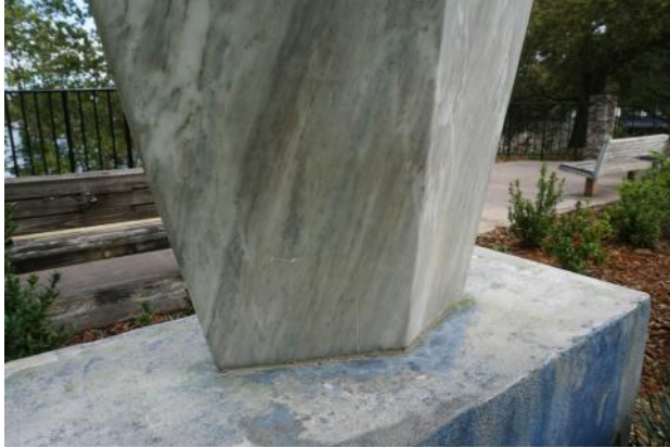
Figure 3. Joint is in good condition, concrete staining has deteriorated (photo by EverGreene, February 2021).
