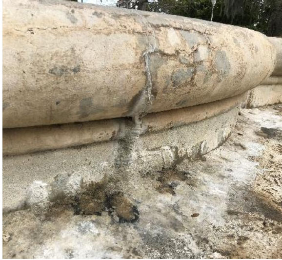
Figure 4. Detail of the typical mineral accretions on the outside of the concrete basin (photo by EverGreene, February 2021).
