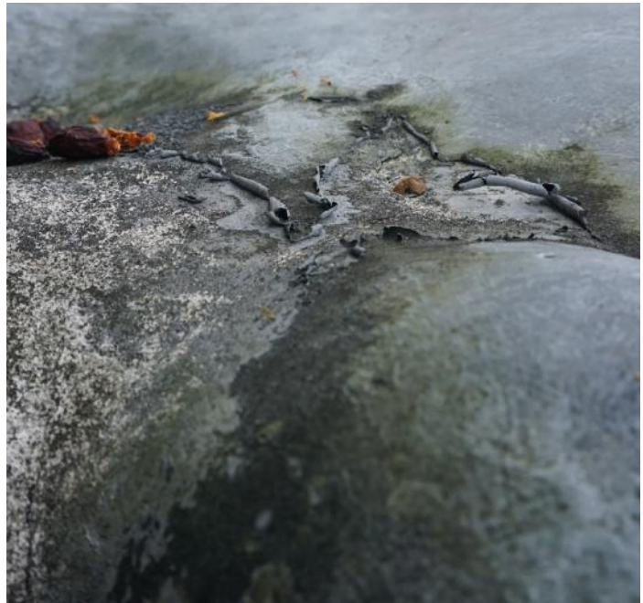
Figure 9. Coating failure and loss (photo by EverGreene, February 2021).
