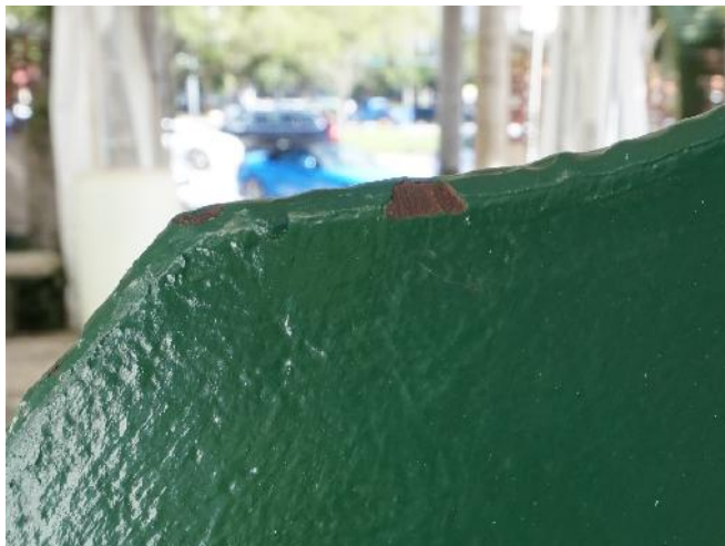
Figure 7. Small chip in metal and paint (photo by EverGreene, February 2021).
