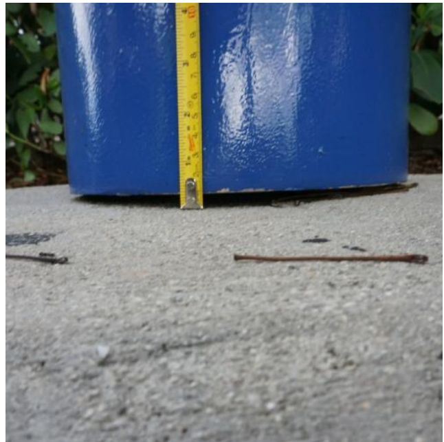
Figure 2. 3/8" gap at the base of the shaft (photo by EverGreene, February 2021).
