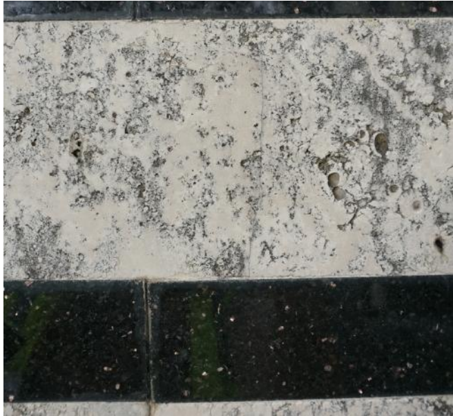
Figure 5. Mortar loss in granite joint, crack in marble (photo by EverGreene, February 2021).
