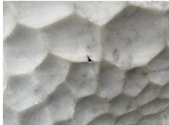
Figure 2. Loss in stone (photo by EverGreene, February 2021).
