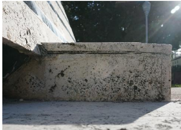
Figure 8. Cracked and displaced marble on step on south side (photo by EverGreene, February 2021).
