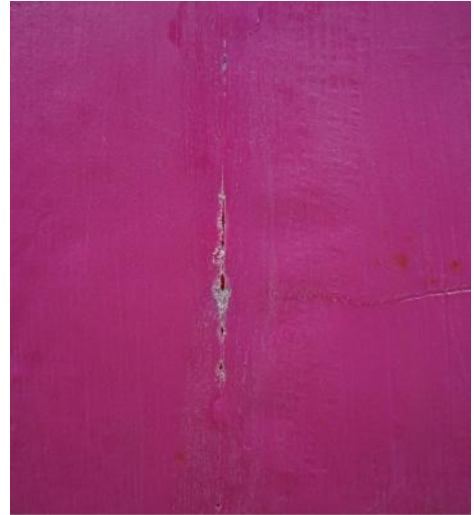
Figure 4. Opening at seam due to deterioration (photo by EverGreene, February 2021).
