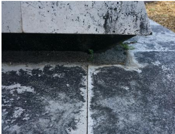
Figure 7. Soiling accumulation under pyramid with plant growth; soiling on marble pavers (photo by EverGreene, February 2021).
