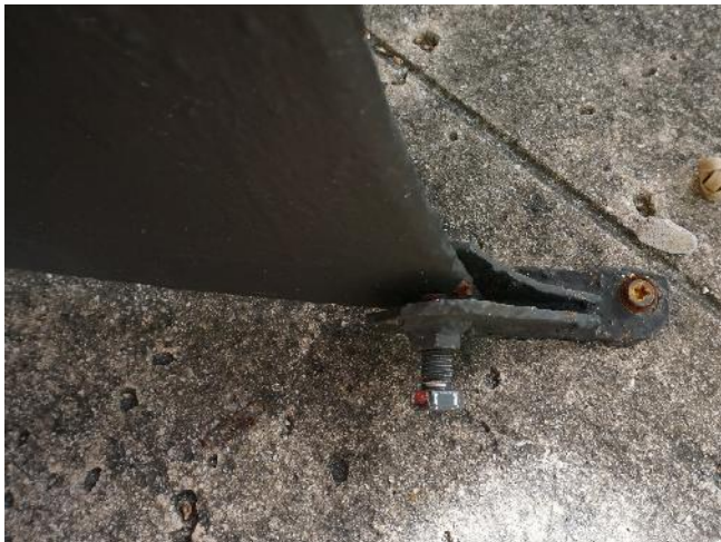
Figure 3. Deteriorated black clamp and Tapcon screw (photo by EverGreene, February 2021).
