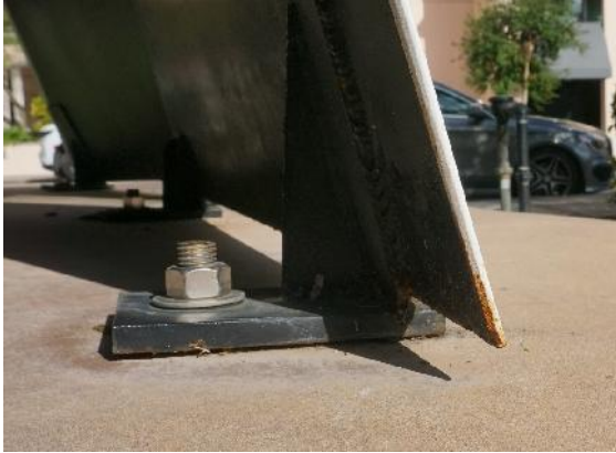
Figure 3. Corrosion on edge (photo by EverGreene, February 2021).
