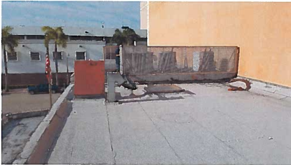
Another view of the rusty steel beam, both beams needs to be replace
