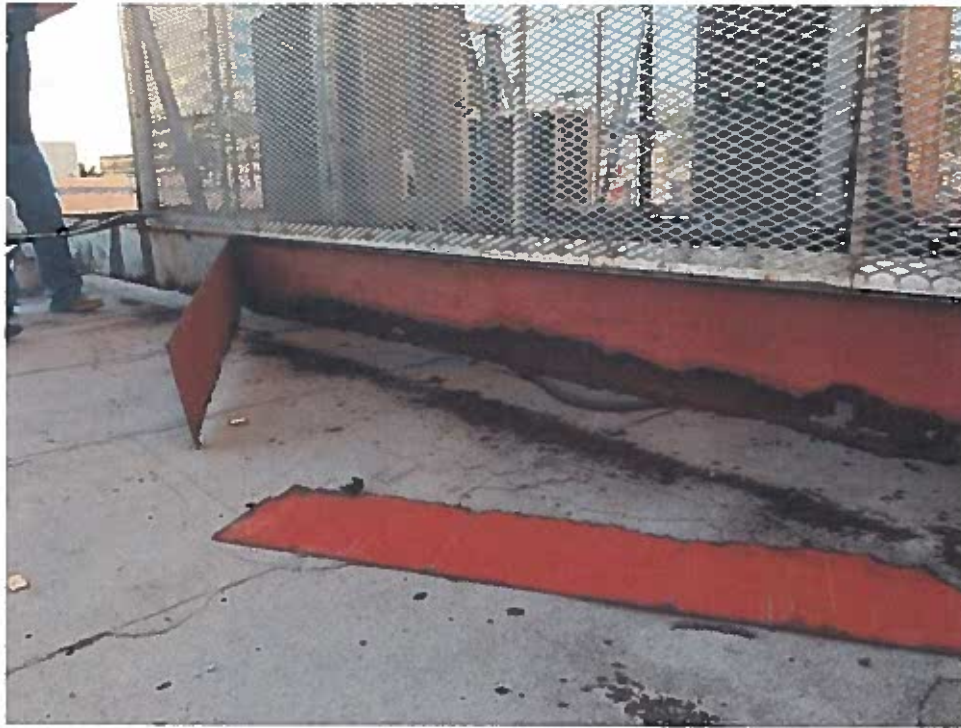
Bottom flange of Steel beam totally corroded
