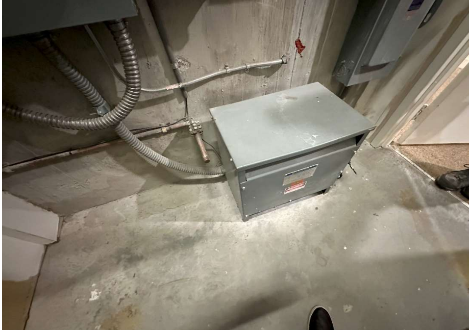
Transformer T82 – 30KVA
