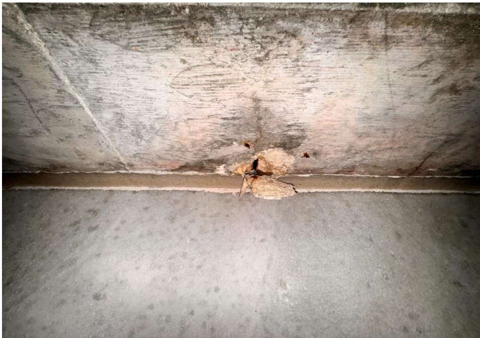
Typical spalling and exposed rebar at garage 2 nd level
