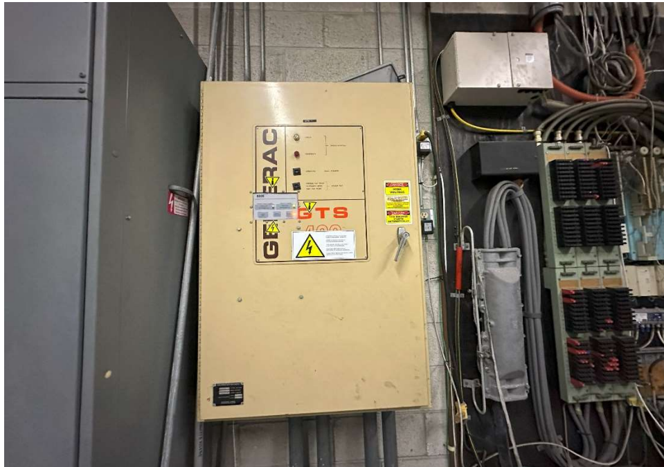
Automatic Transfer Switch (ATS) -
