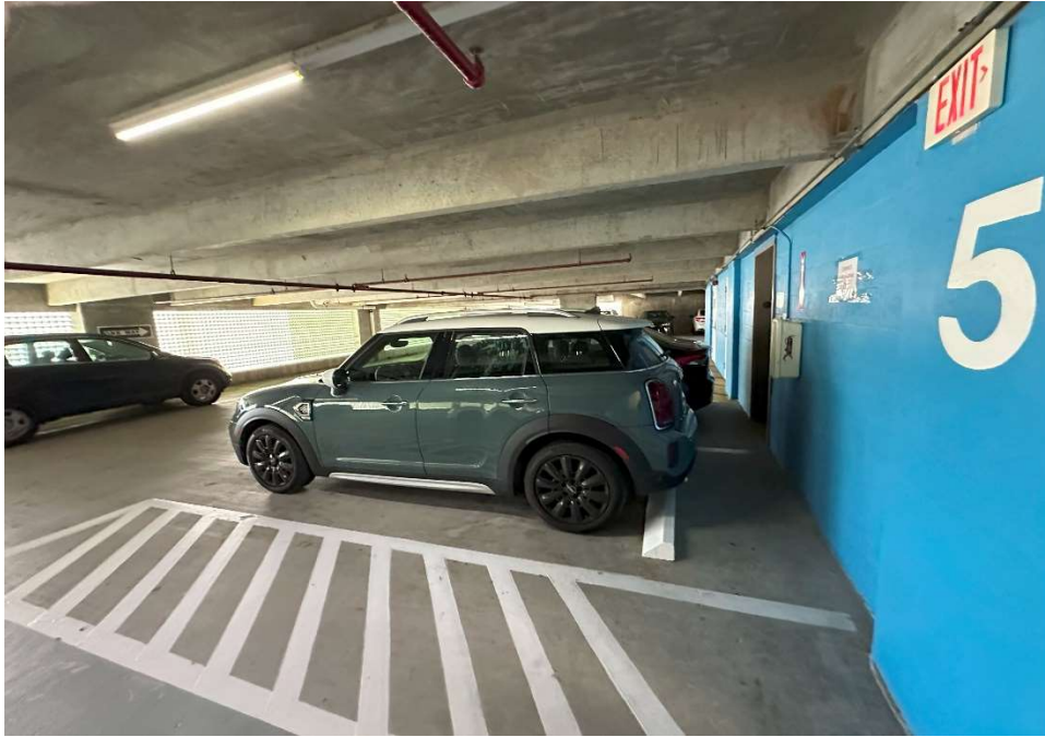
Emergency/Exit Lighting, Typical of garage Floors
