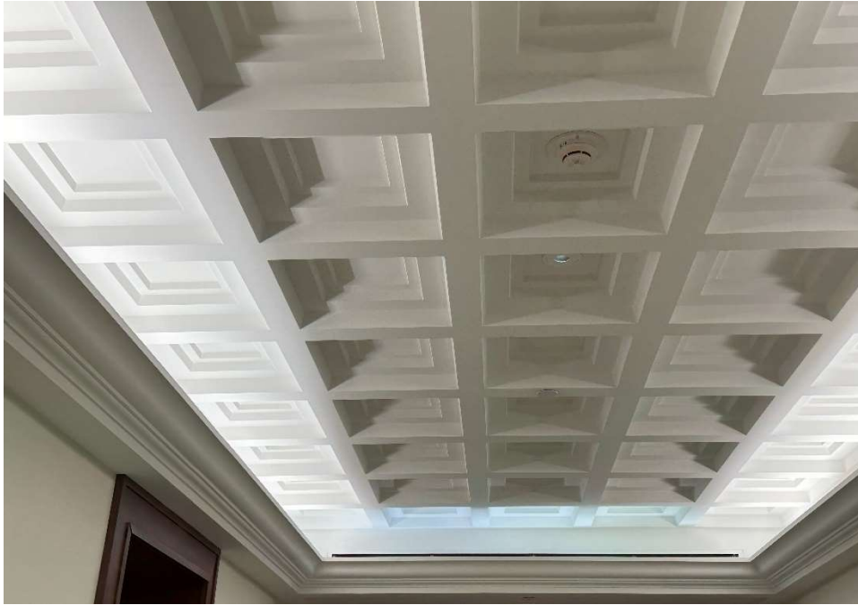
Smoke Detector at Elevator Lobby –
