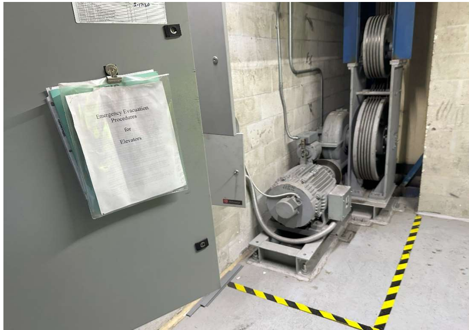
Elevator Machine Room 4 -
