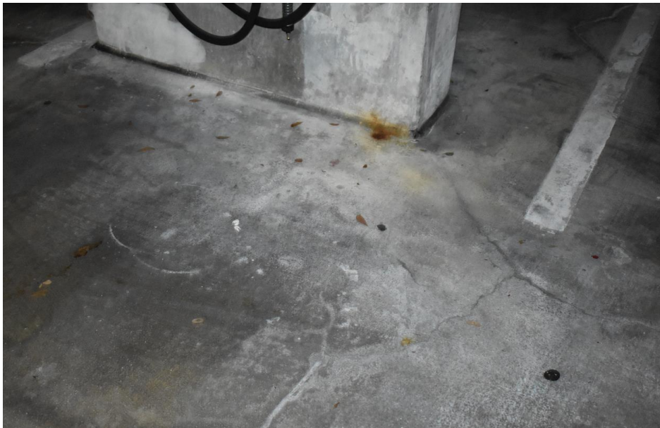
Typical cracks along the top of the spread and combined footings in the basement
