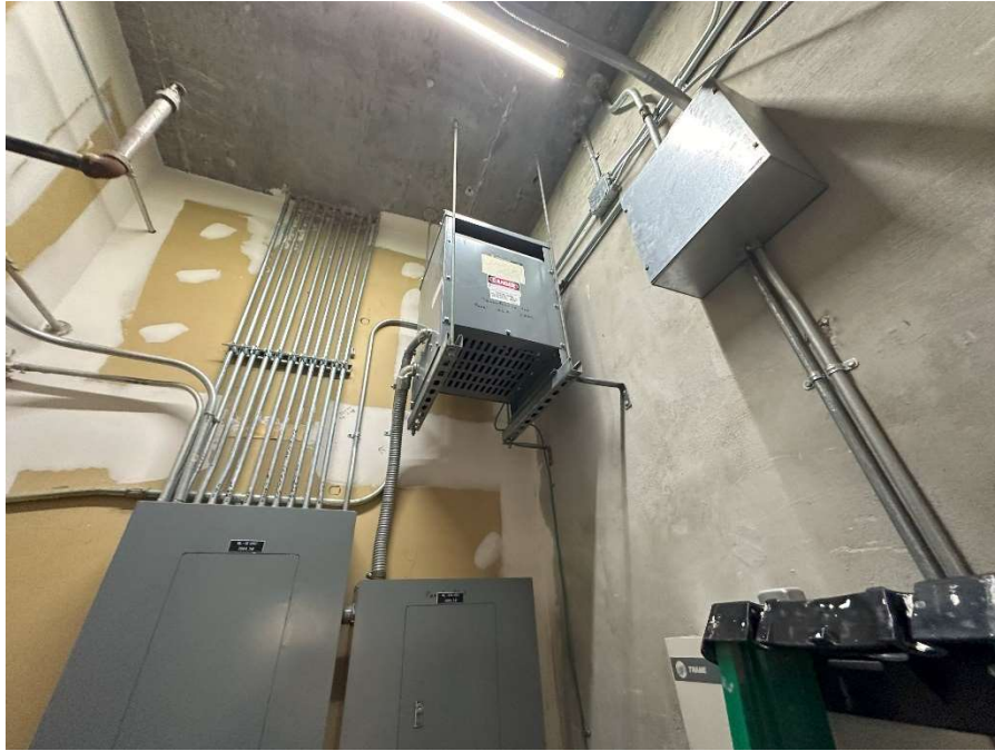
Transformer T102 – 30KVA
