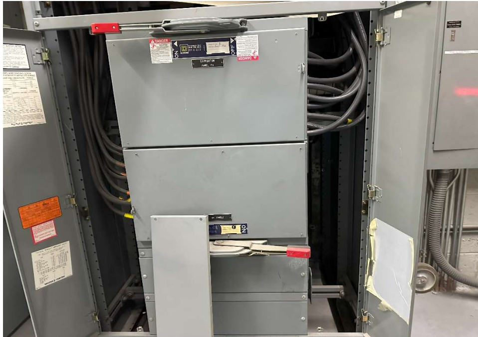
Main 4 of 5 Opened – 400 Amps – Panel NH
