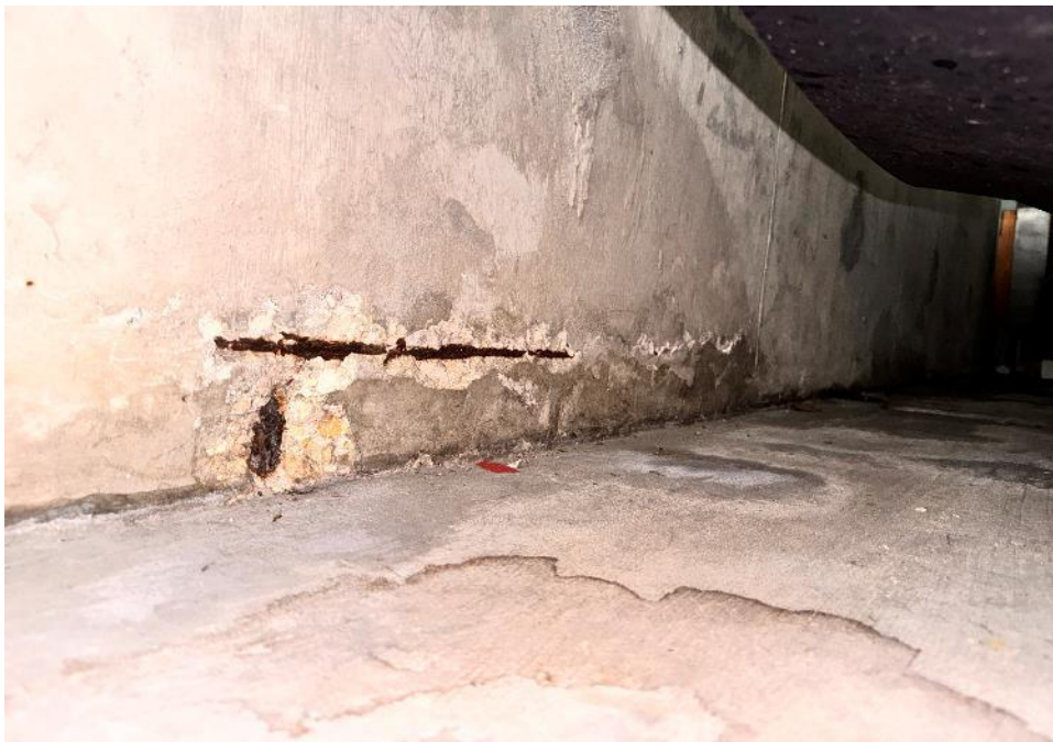
Typical spalling and exposed rebar at the garage levels
