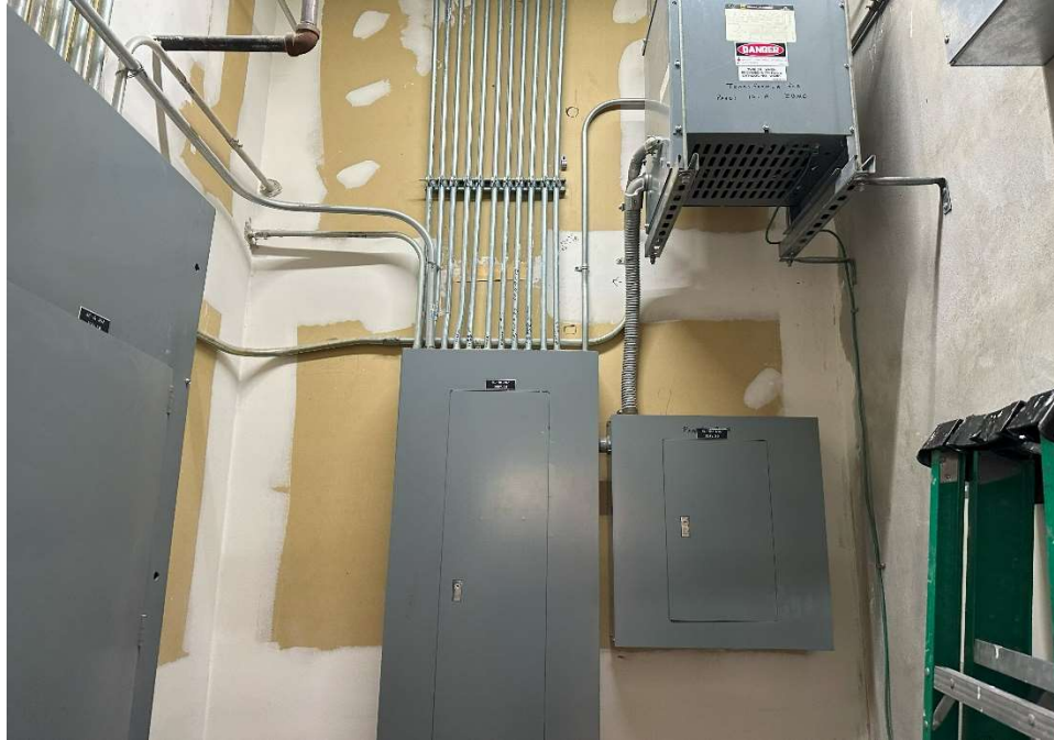
10 th Floor Electrical Room
