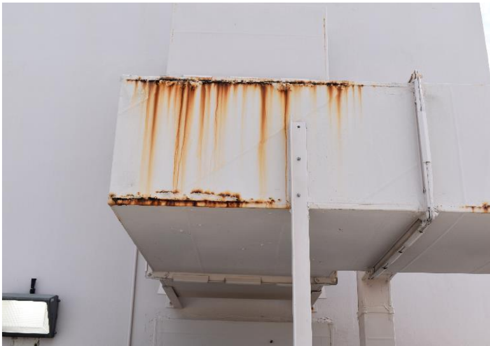
Corroded metals of the roof top ducts
