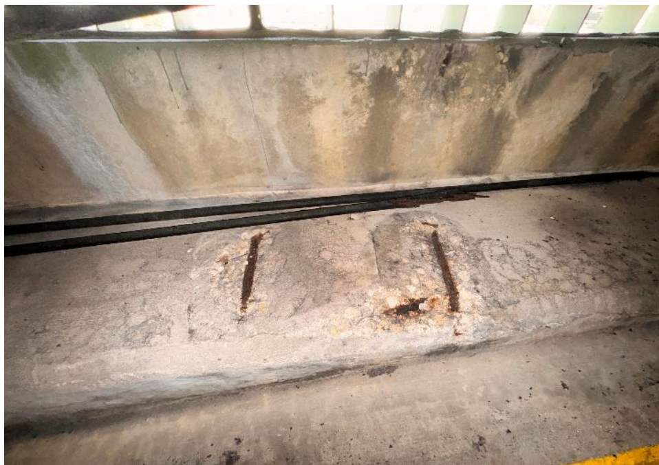
Typical spalling and exposed rebar at the garage 5 th level
