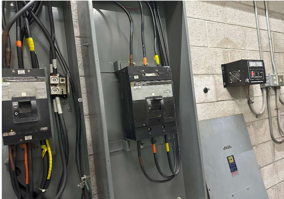
Fire Pump Disconnect -
