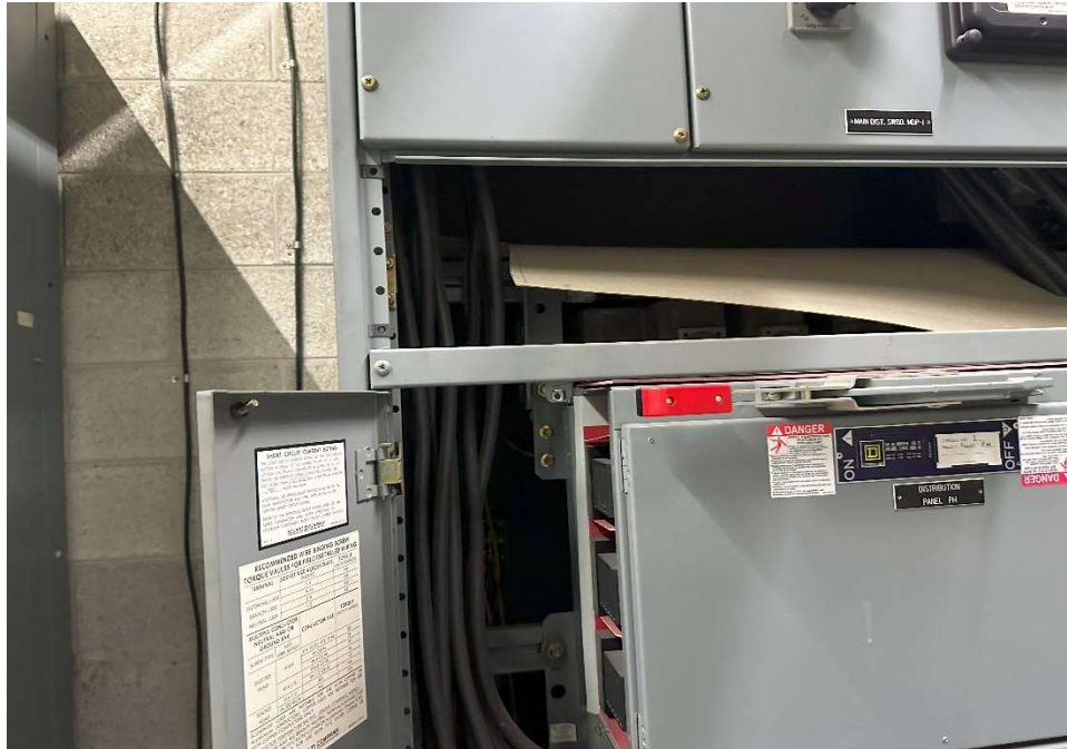
Main 3 of 5 Opened – 400 Amps – Panel PH
