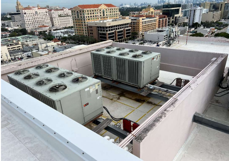
RTU Package Units on Roof
