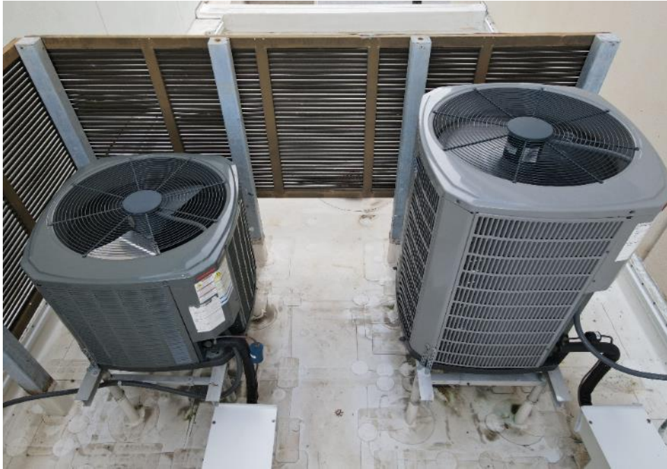
RTUs on the small low-slope roof of the east elevation
