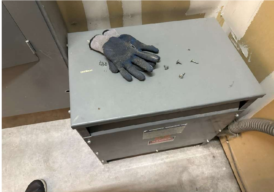
Transformer T92 – 30KVA
