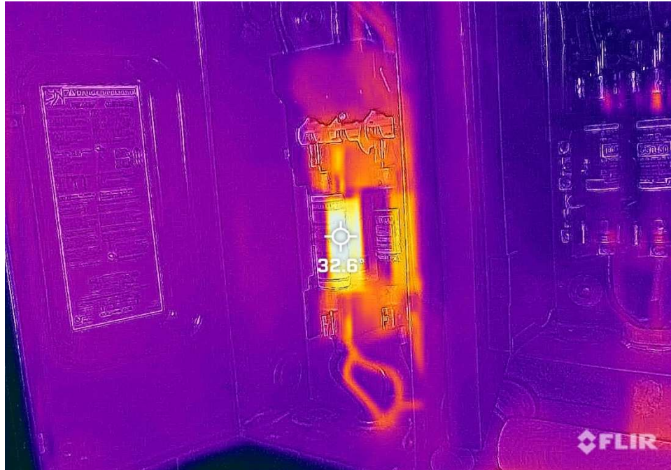
Item 30: Mech Disconnect at 32.6 Degrees Celsius (delta 7.6C)
