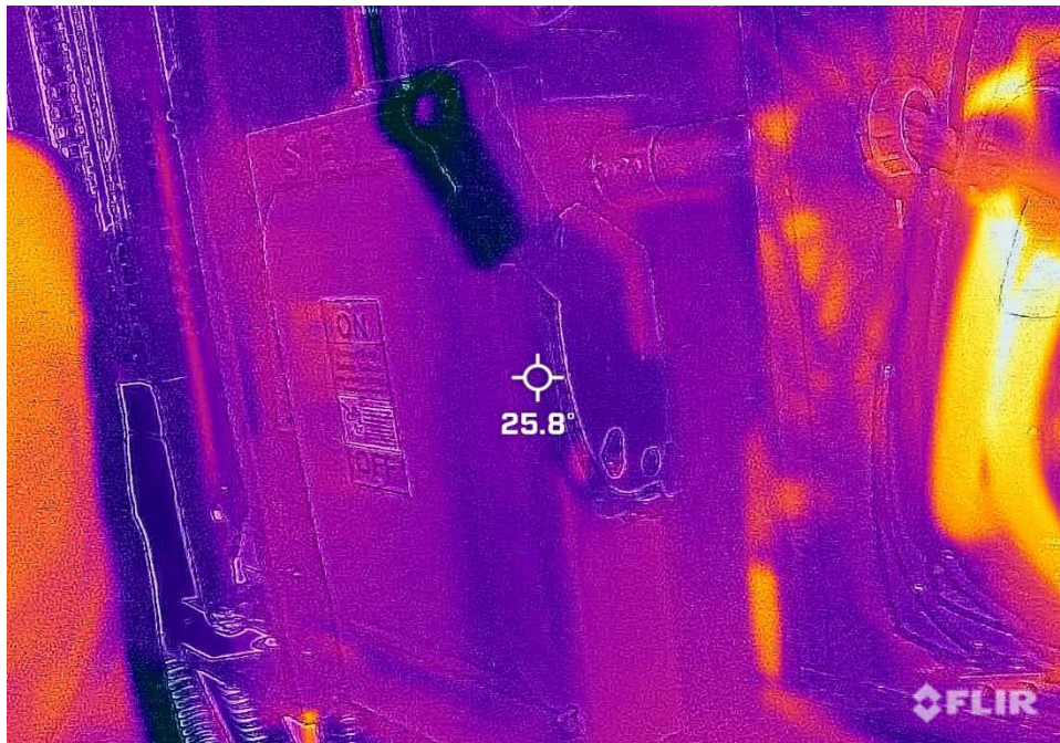
Item 42: Disconnect at 25.8 Degrees Celsius (delta 2.8C)
