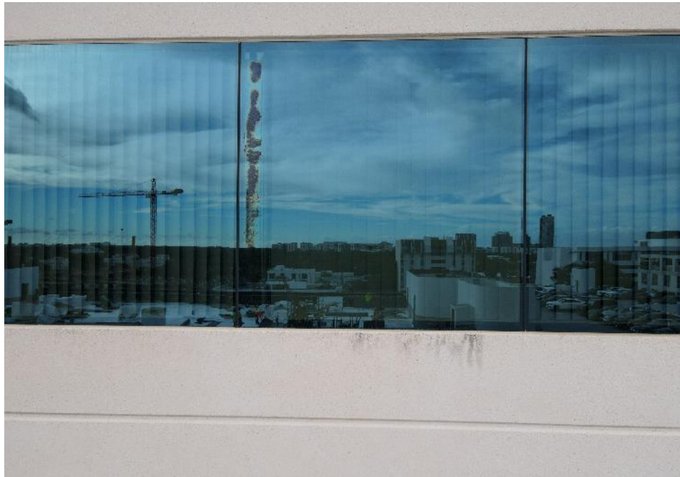
Corrosion staining at the windows at random locations
