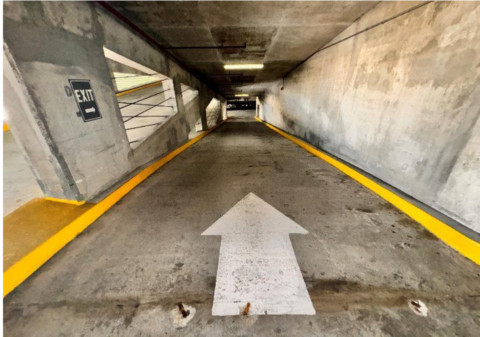
Ramp at garage levels with spalling
