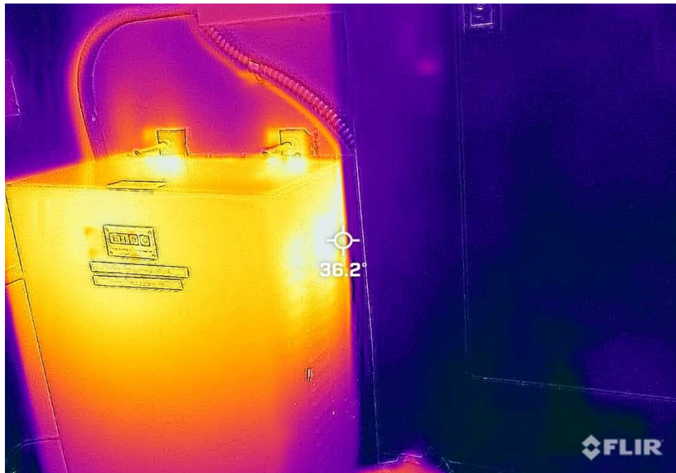
Item 38: Transformer at 36.2 Degrees Celsius
