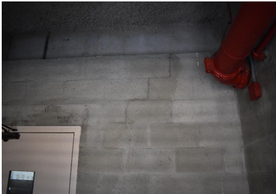
Stairstep cracking at CMU walls
