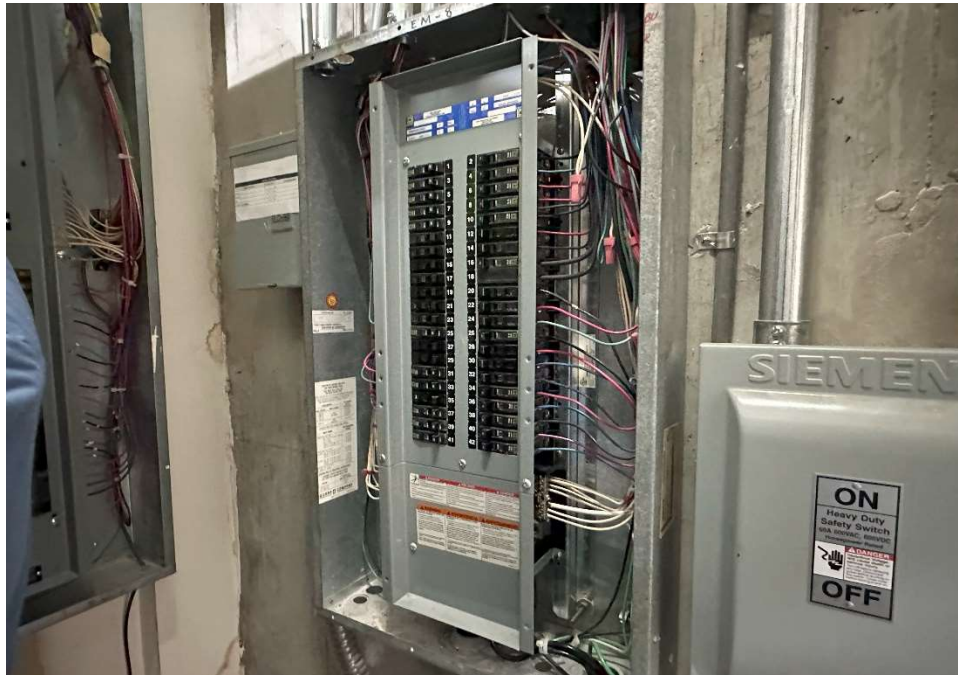
Panel EM8 Opened –
