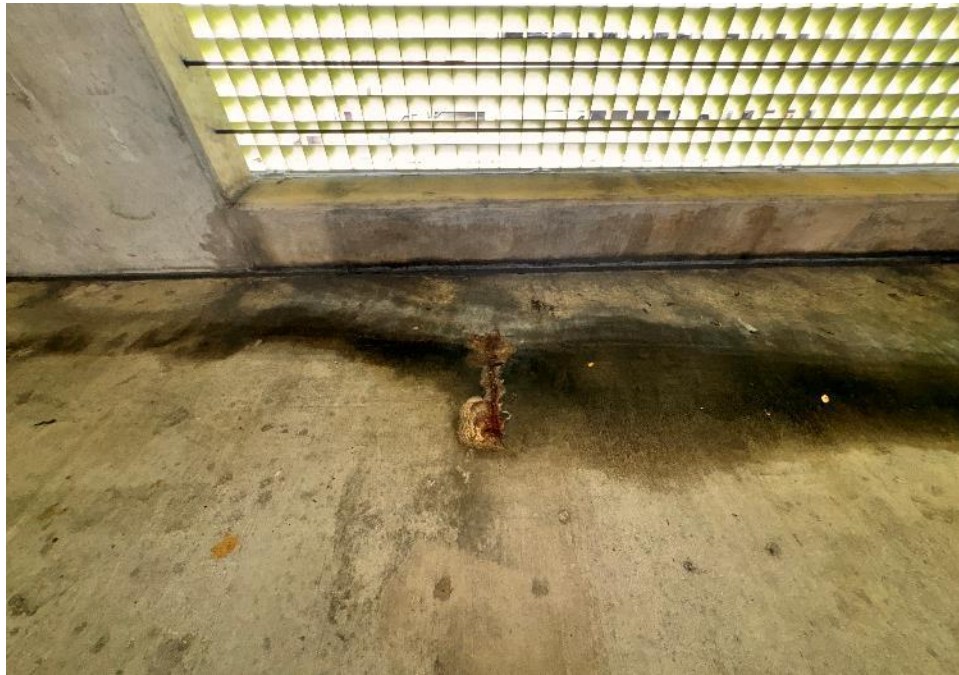
Typical spalling and exposed rebar at the garage 4 th level
