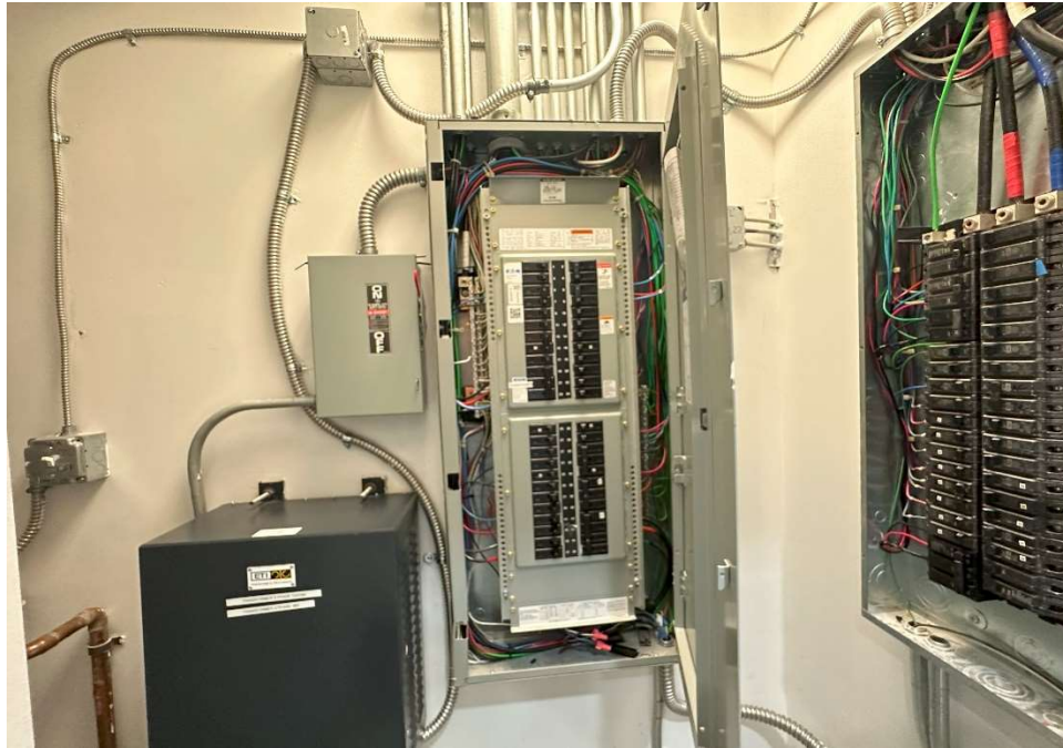
Panels A, DMFL & 75KA Transformer Opened -
