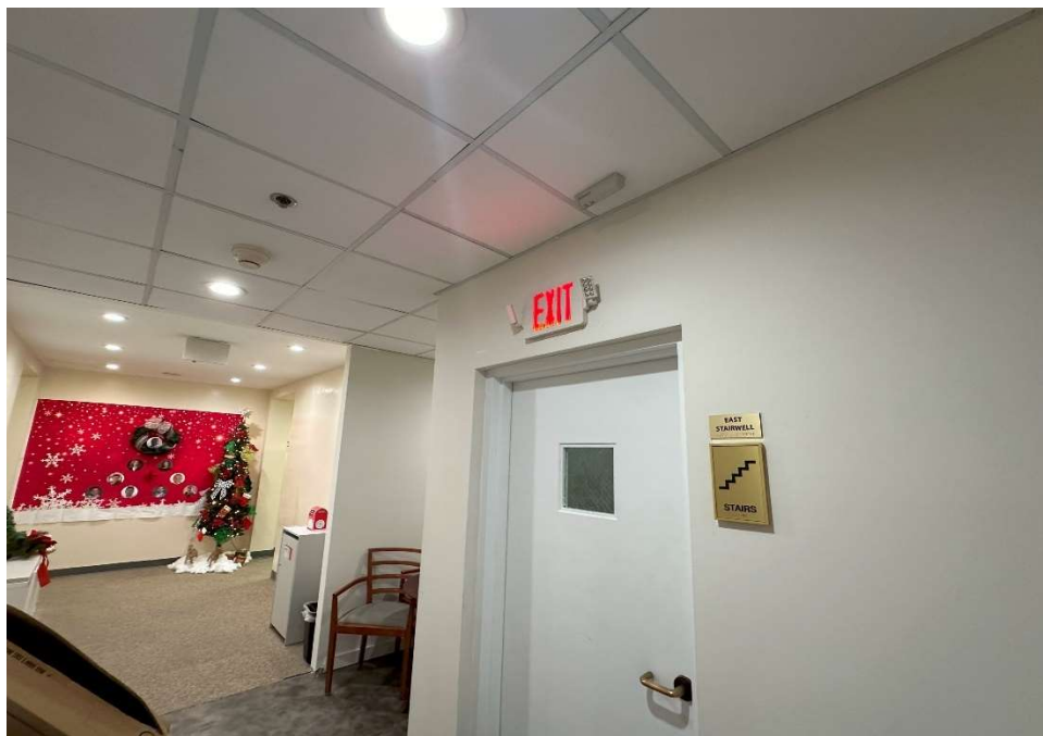
Means of Egress Lighting – Exit Lighting -
