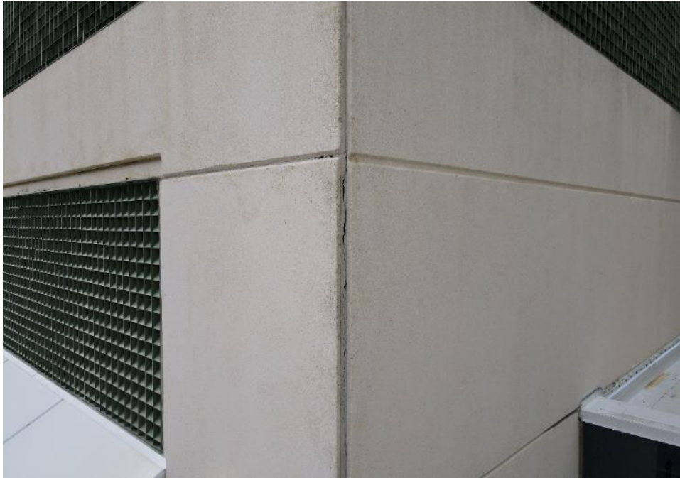
Random deteriorated joints along the exterior panel joints
