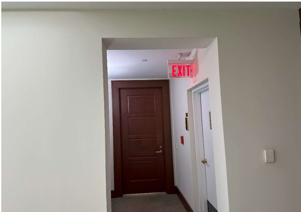
Means of Egress Lighting – Exit Lighting -
