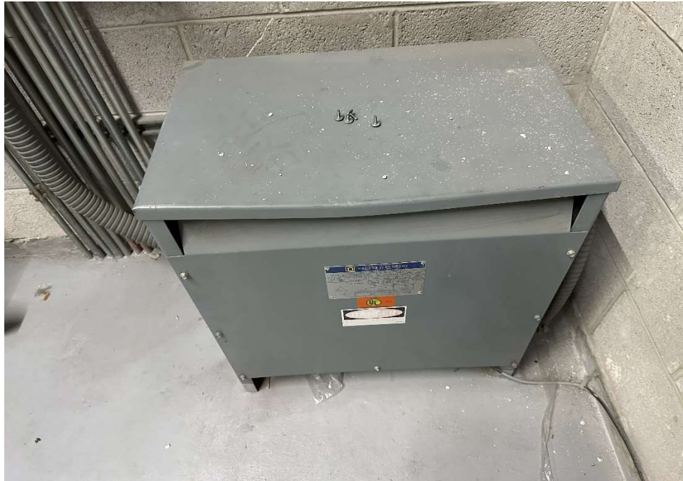
Transformer T1 – 45KVA – 480-208Y/120V
