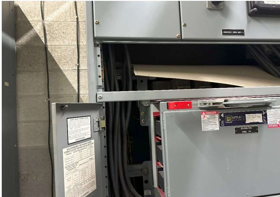
Main 3 of 5 Opened – 400 Amps – Panel PH
