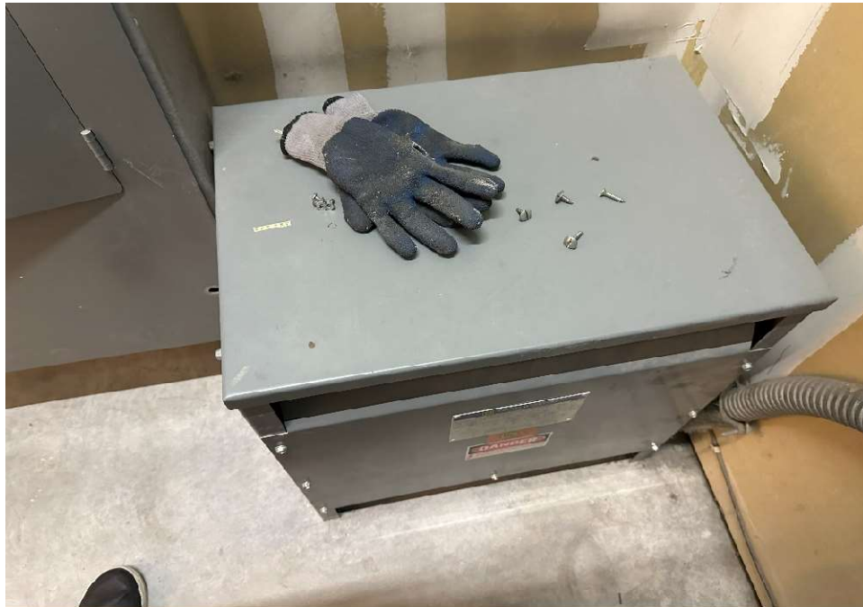
Transformer T92 – 30KVA
