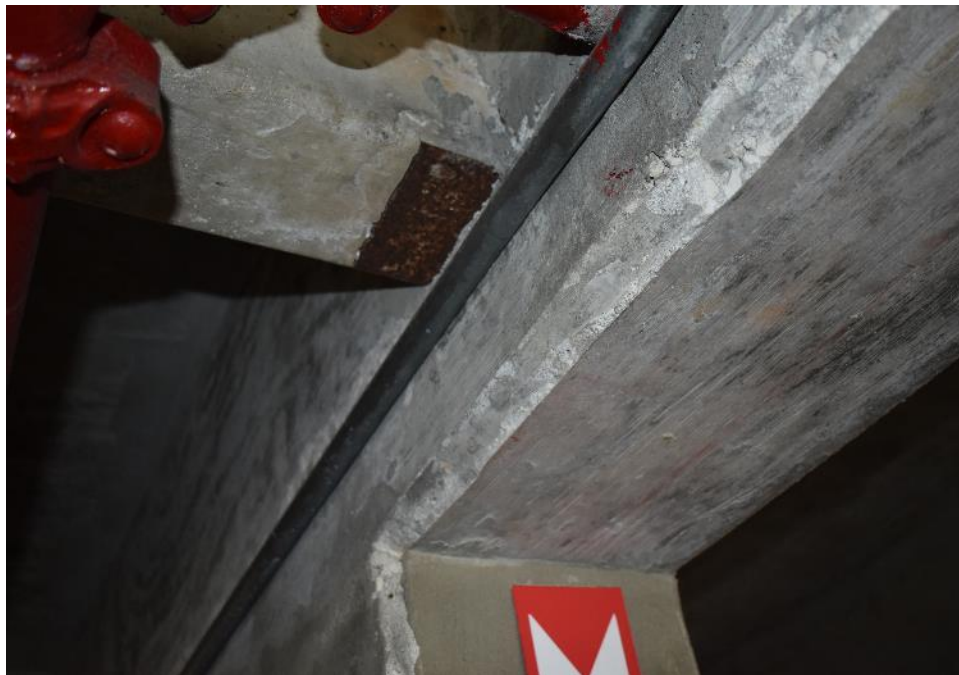
Typical corroded angles at the PCJ to wall/beam connections
