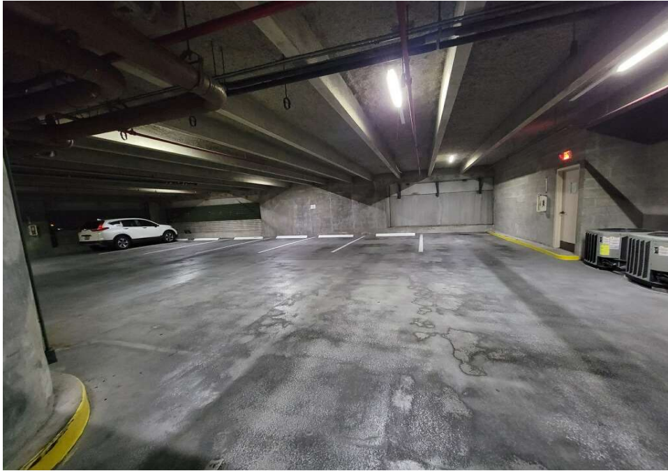
Parking Lot lighting, Typical for Floors Ground Through 7 –
