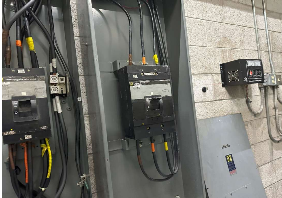
Fire Pump Disconnect –
