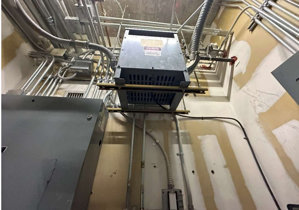
Transformer T122 – 75KVA
