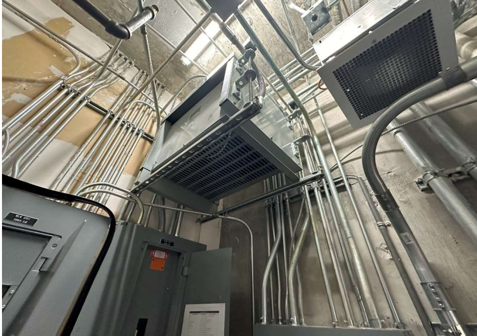
Transformer T83 – 30KVA
