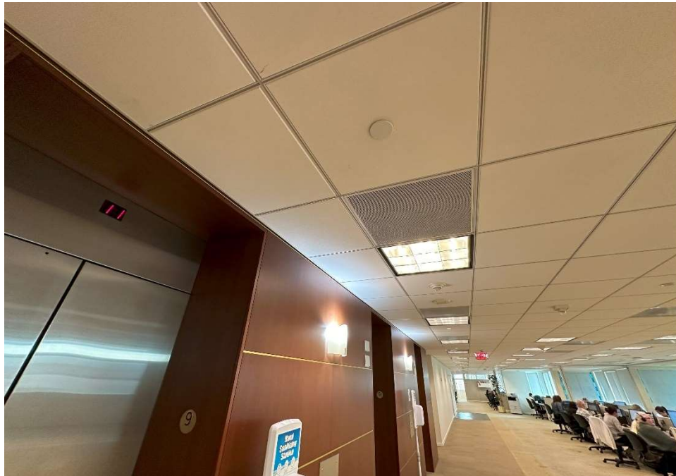
Smoke Detector at Elevator Lobby –
