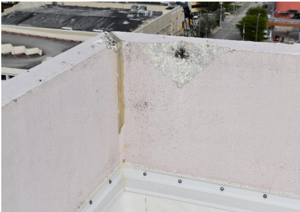
Spalling at the parapet walls
