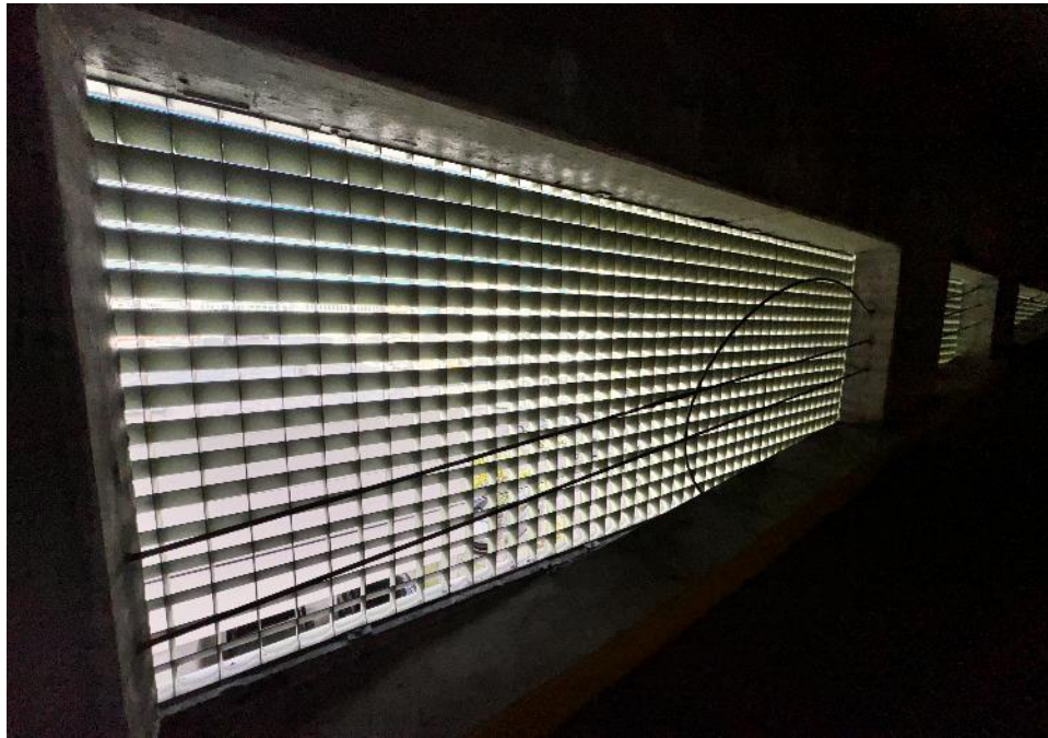
Detached barrier cable at garage level
