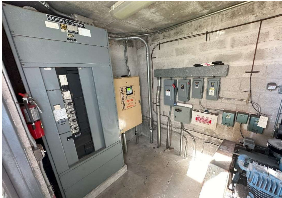
Elevator Machine Room Layout – Tied to Generator - Roof
