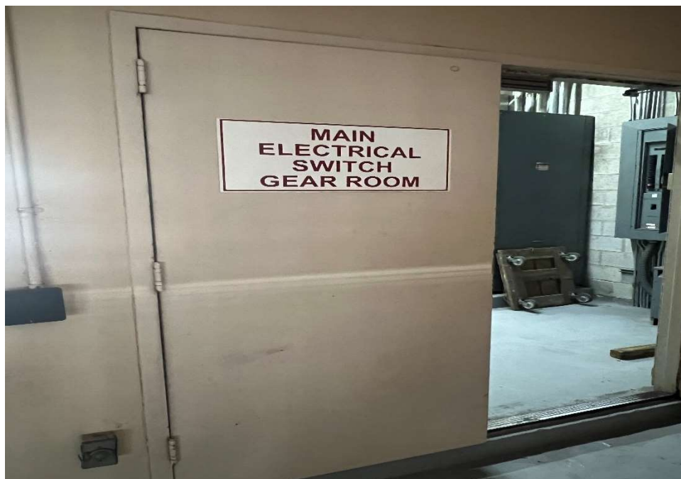
Service Entrance – Main Electrical Switchgear Room -
