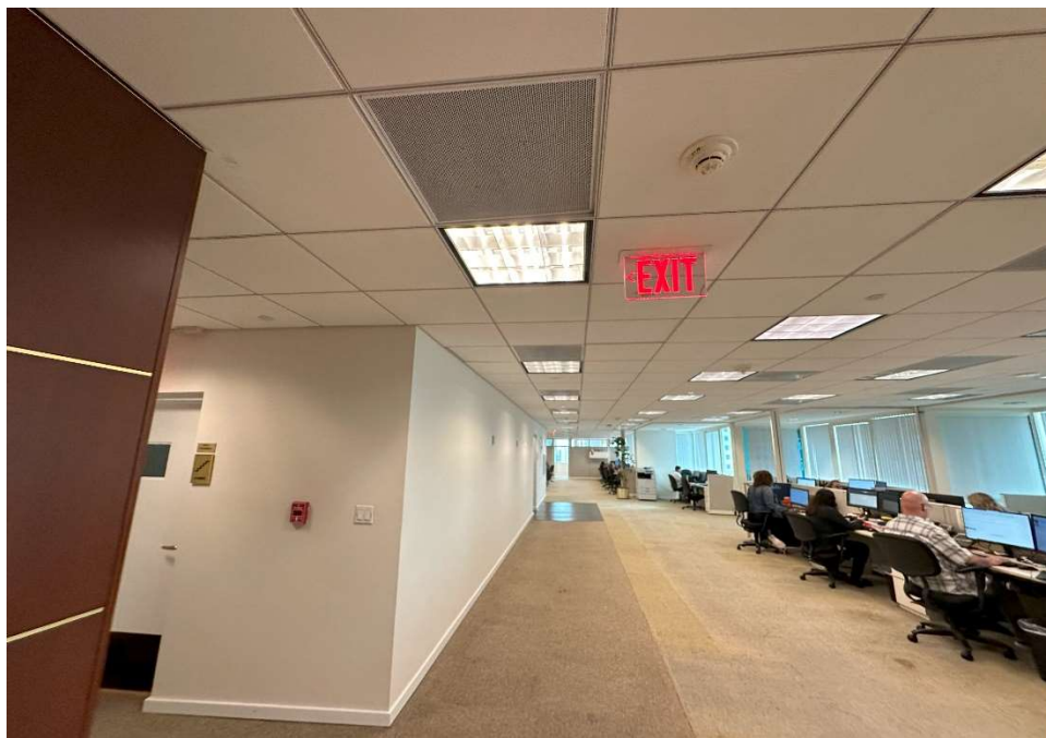
Means of Egress Lighting – Exit Lighting -
