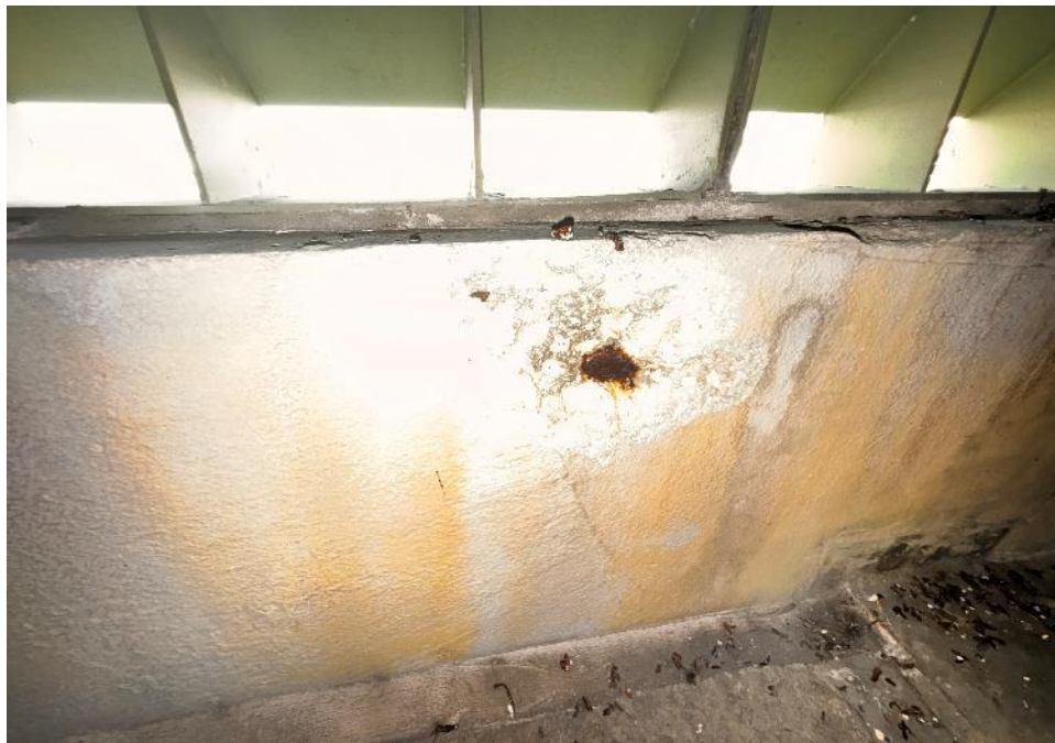
Typical spalling and exposed rebar near louvers at the garage 4 th level
