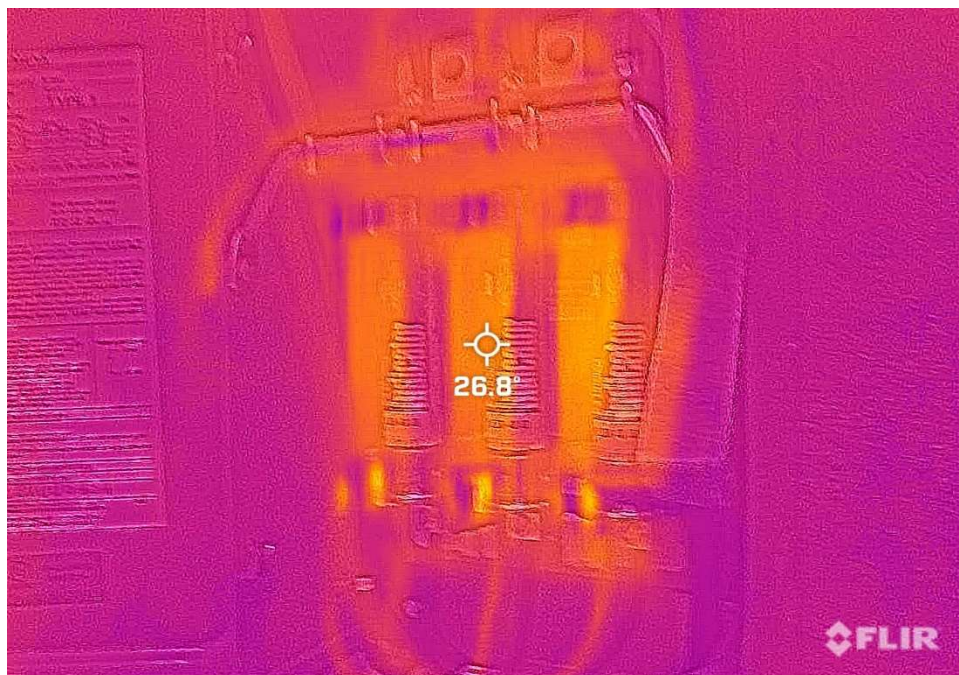
Item 52: Disconnect at 26.8 Degrees Celsius (delta 4.8C)
