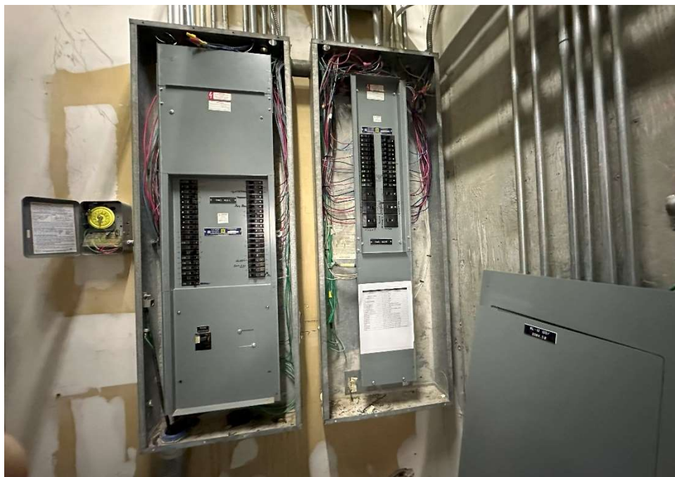
Panels NL12L and NL12R Opened -
