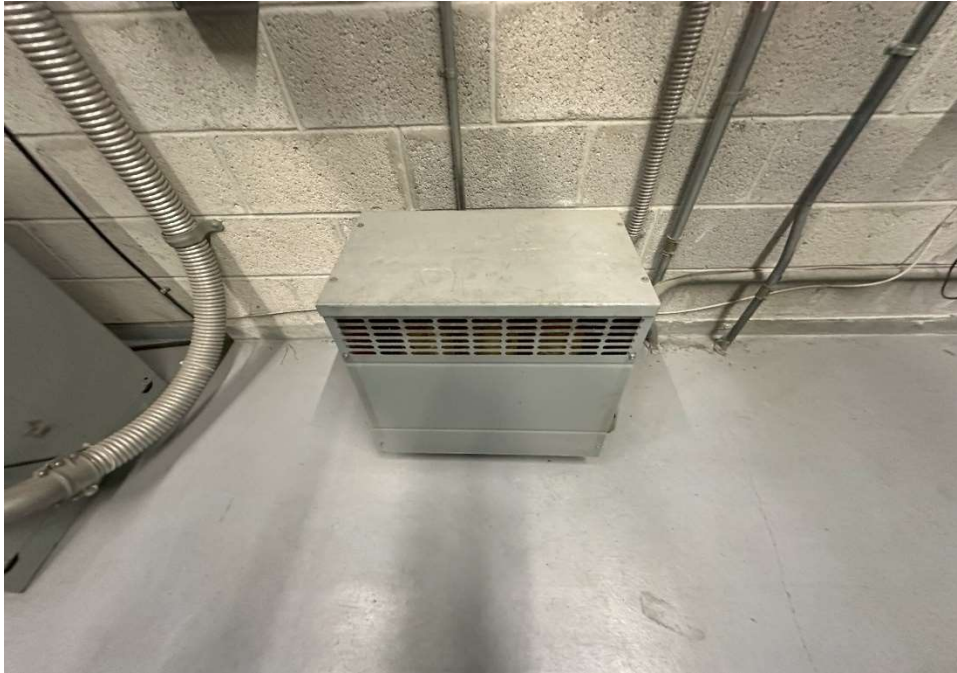
Transformer T3 – 30KVA – 480-208Y/120V
