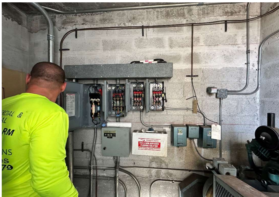
Elevator Disconnects Opened -
