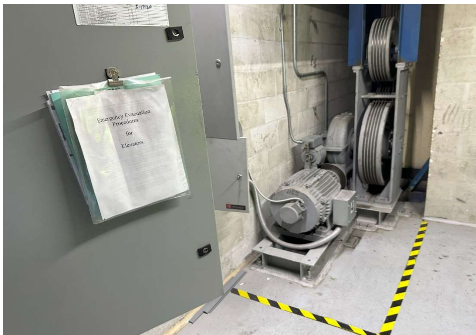
Elevator Machine Room 4 - Page 25 of 71
