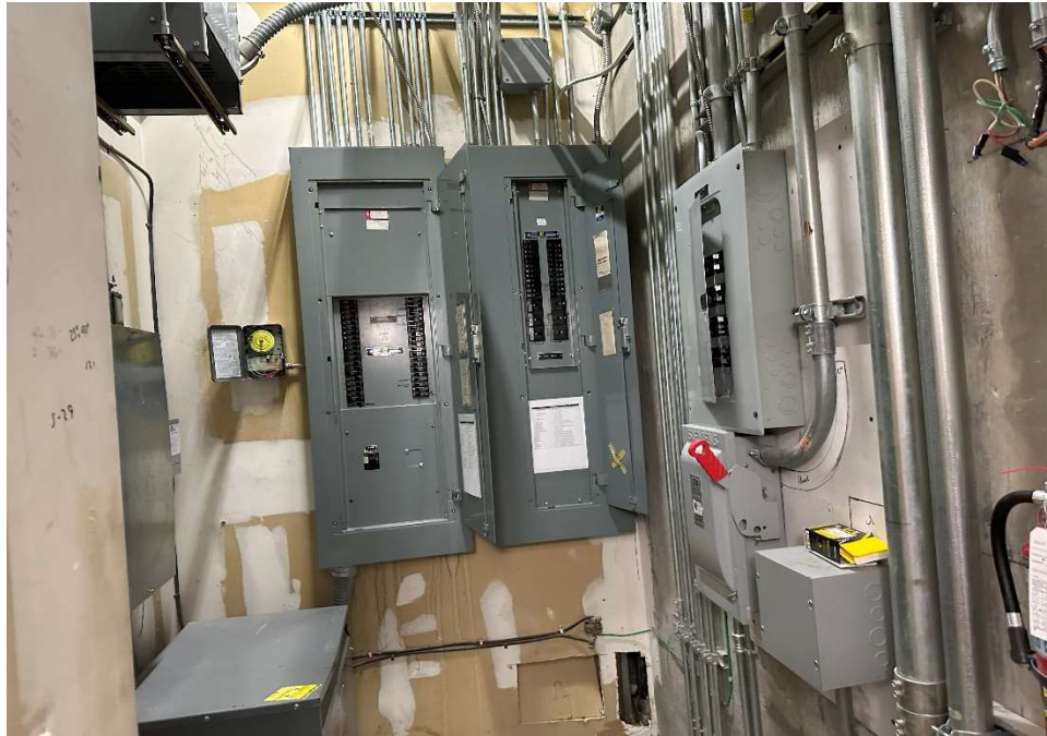
PH Electrical Room -
