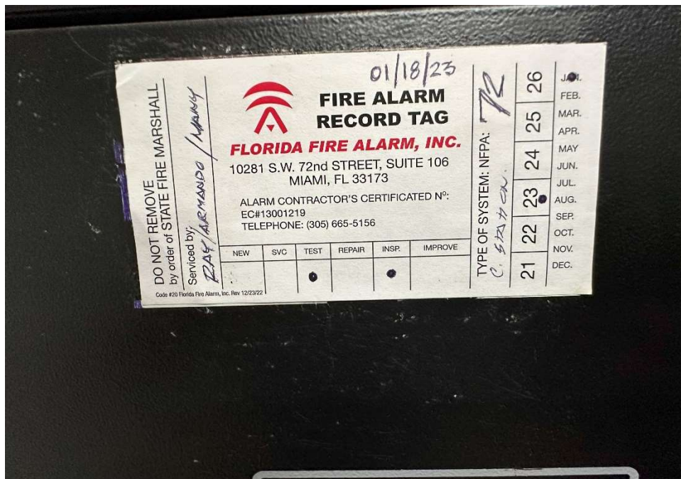
Fire Alarm System Certified 2023 – Renew Certification January 2024 -
