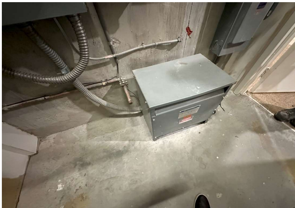
Transformer T82 – 30KVA
