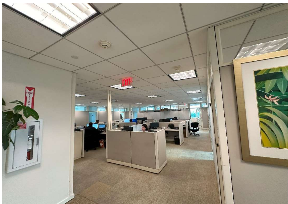
Means of Egress Lighting – Exit Lighting -
