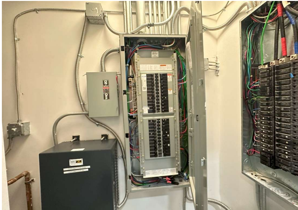
Panels A, DMFL & 75KA Transformer Opened –
