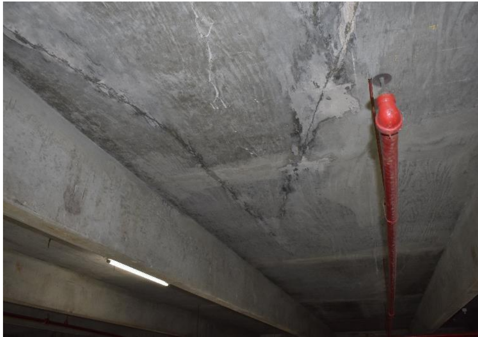
Typical cracks along the concrete deck at the garage level
