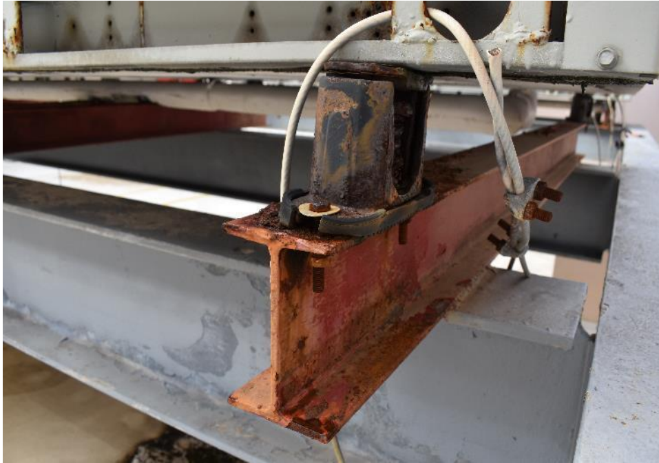
Corroded steel supports for the roof top equipment
