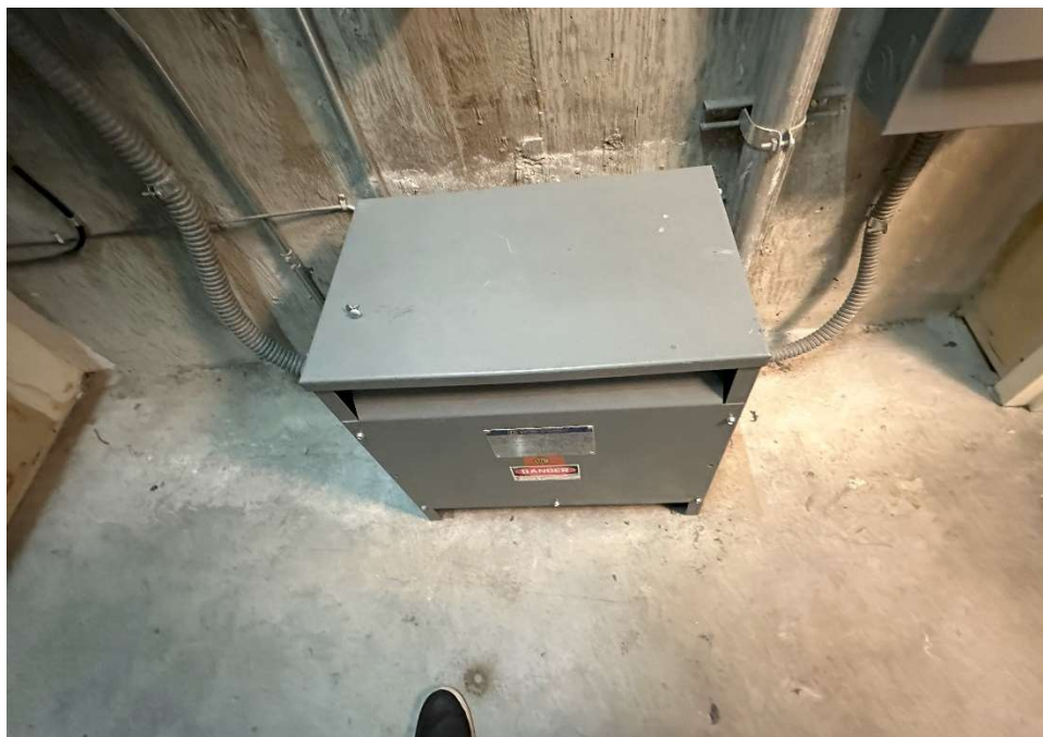
Transformer T121 – 75KVA
