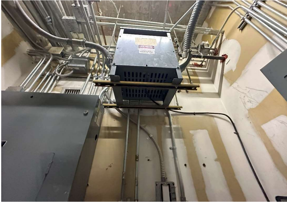
Transformer T122 – 75KVA
