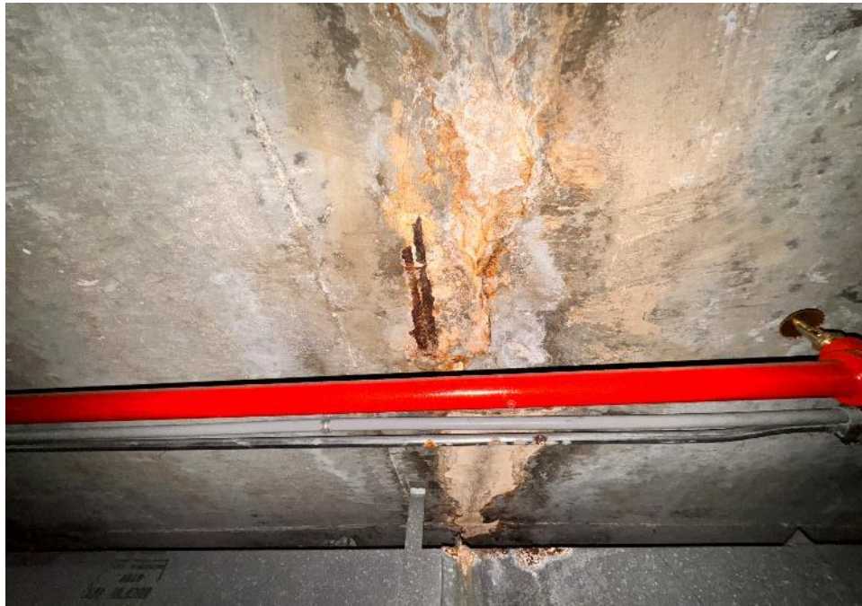
Typical cracks with efflorescence/moisture at the garage 2 nd level
