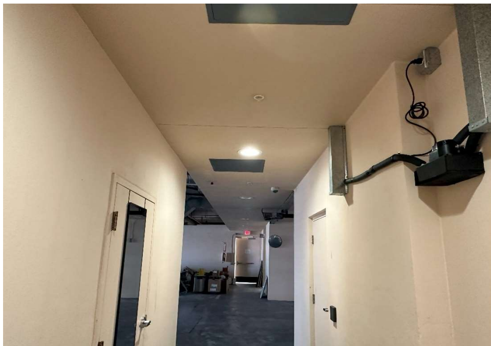
Exit Lighting Ground Floor
