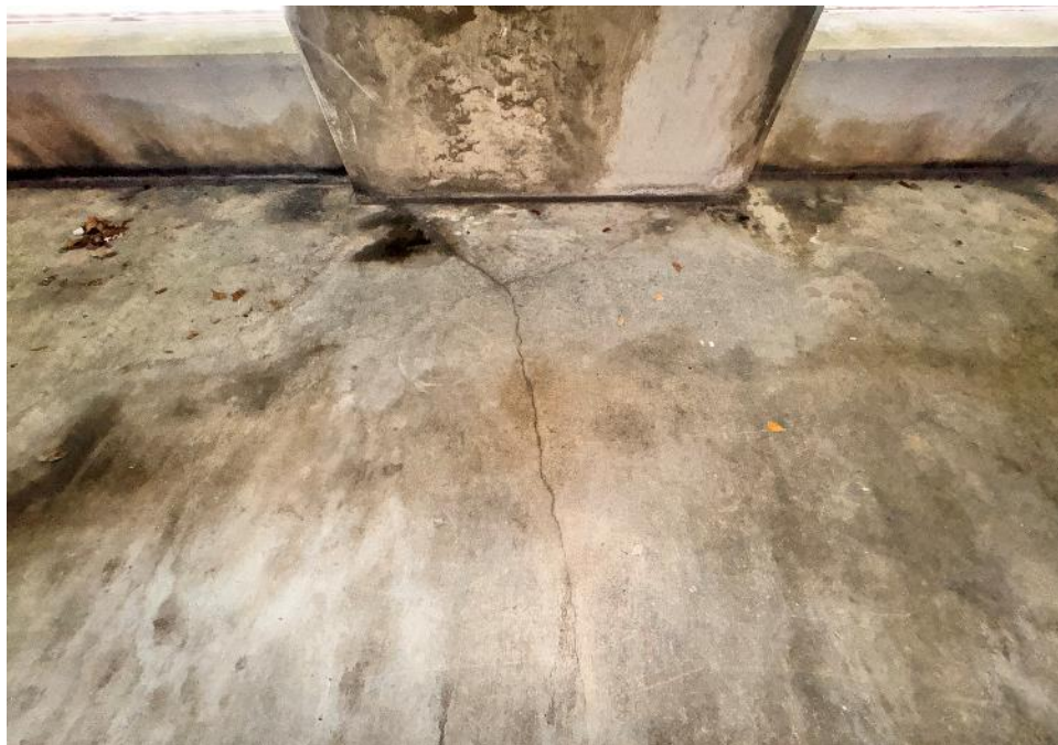
Cracking at the concrete decking-column connection on the garage 6 th level
