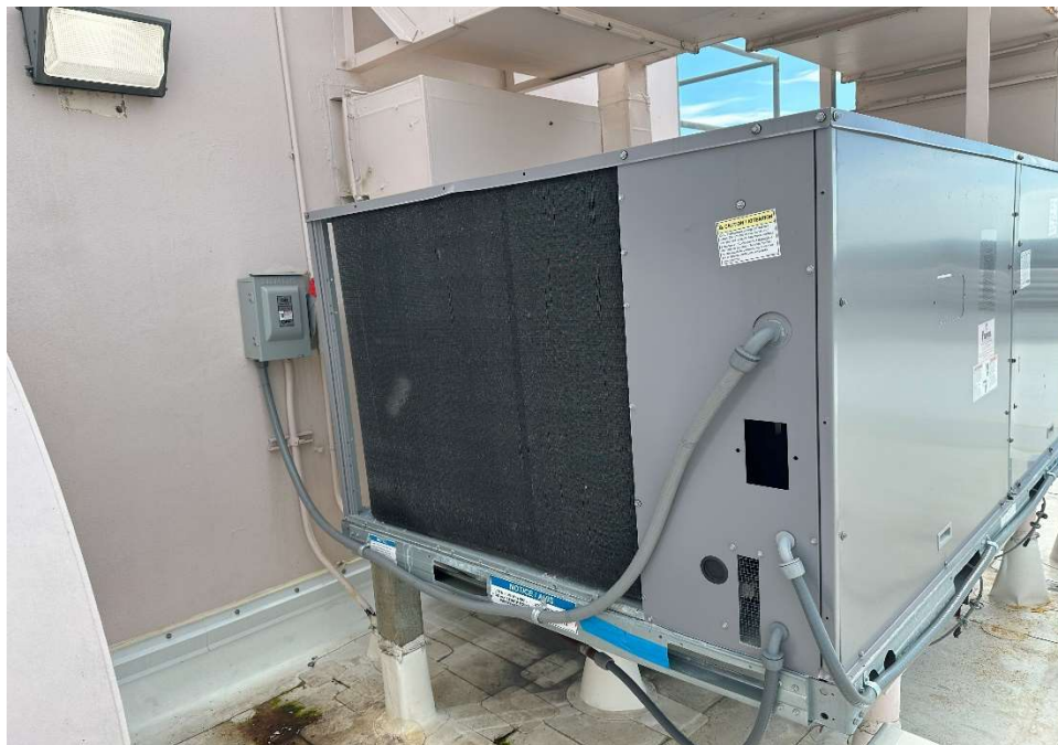
RTU Package Unit on Roof -
