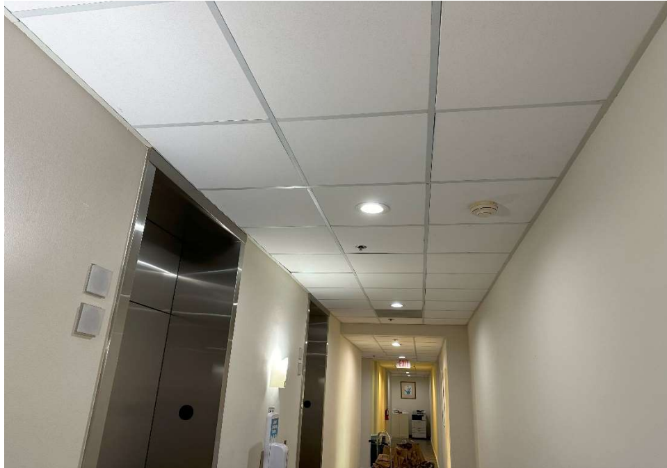
Smoke Detector at Elevator Lobby -
