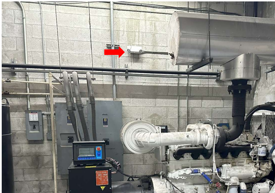
Emergency Light in Generator Room – Typical of All Elec/Mech Rooms -
