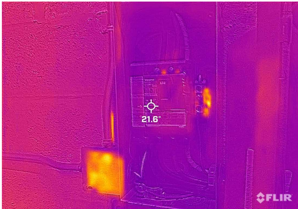
Item 27: Service Disconnect at 21.6 Degrees Celsius (zero delta)
