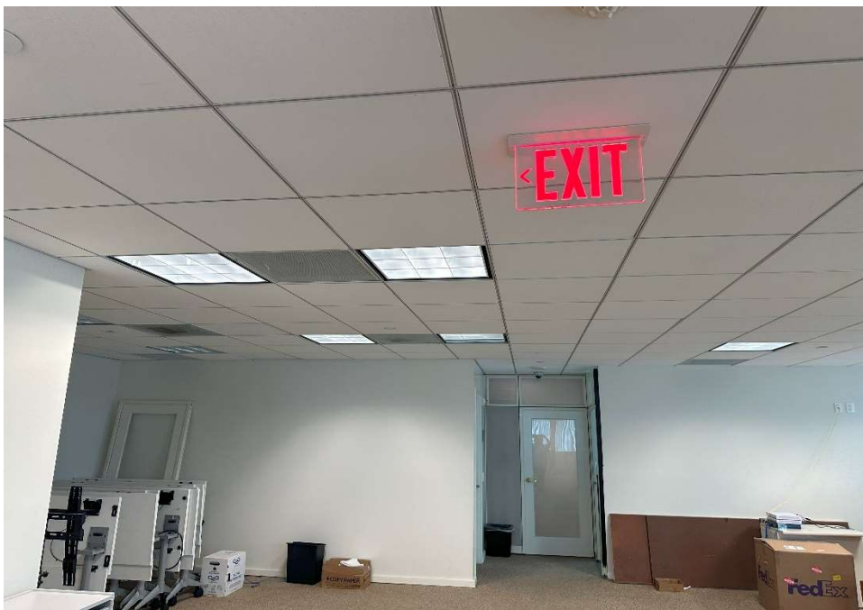
Means of Egress Lighting – Exit Lighting -
