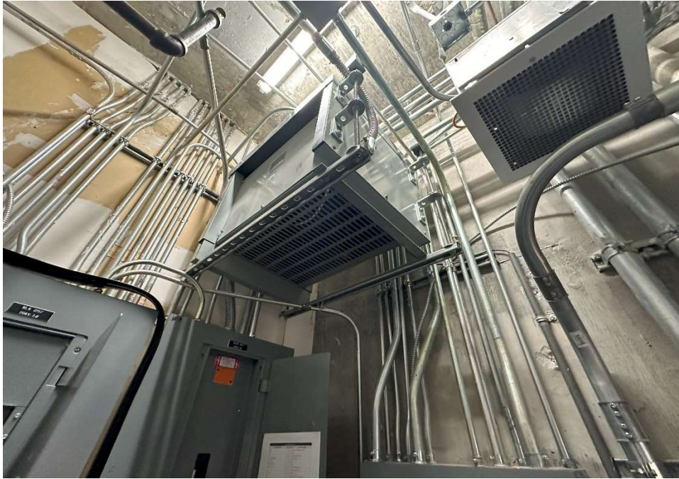
Transformer T83 – 30KVA
