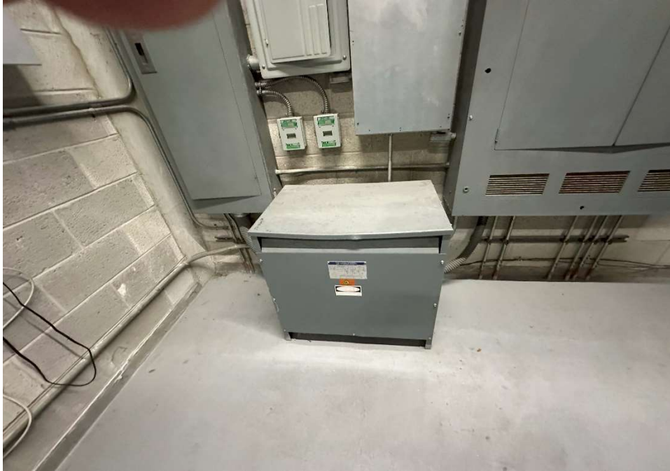
Transformer T2 – 75KVA – 480-208Y/120V
