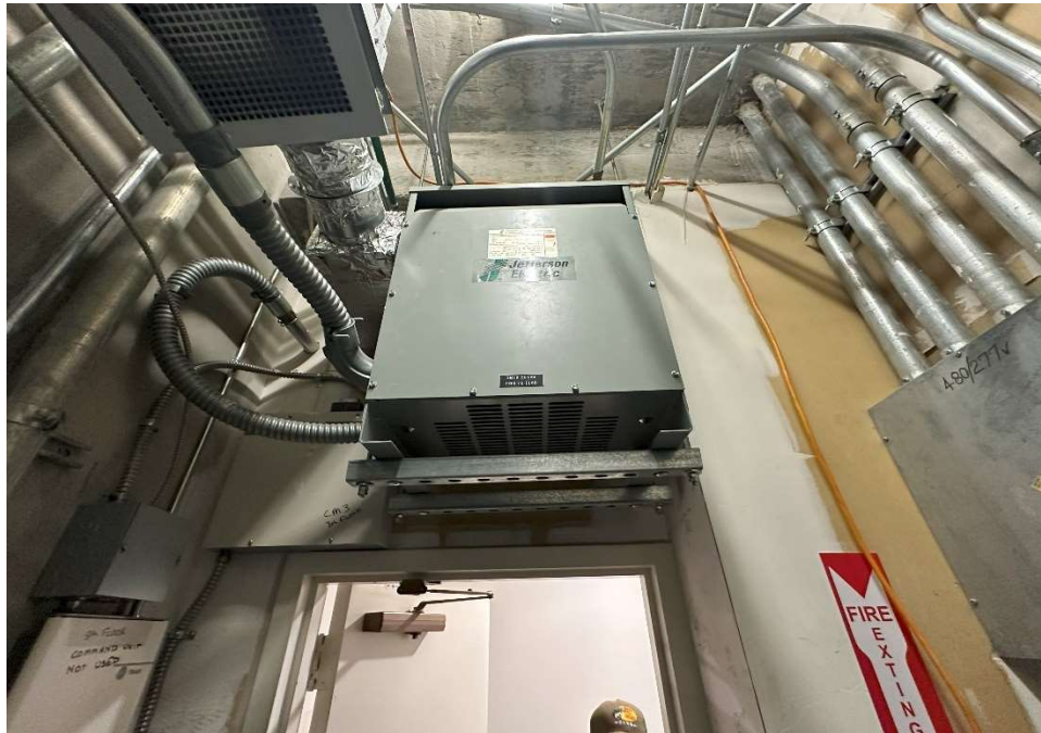
Transformer T81 – 30KVA
