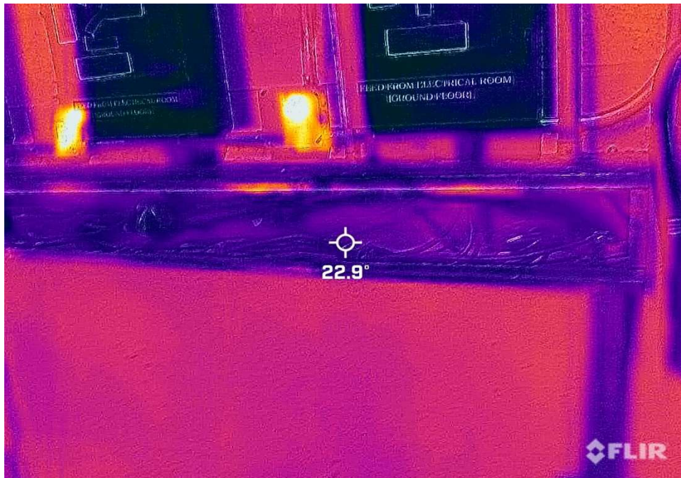
Item 26: Gutter at 30.0 Degrees Celsius (delta 9.0C)
