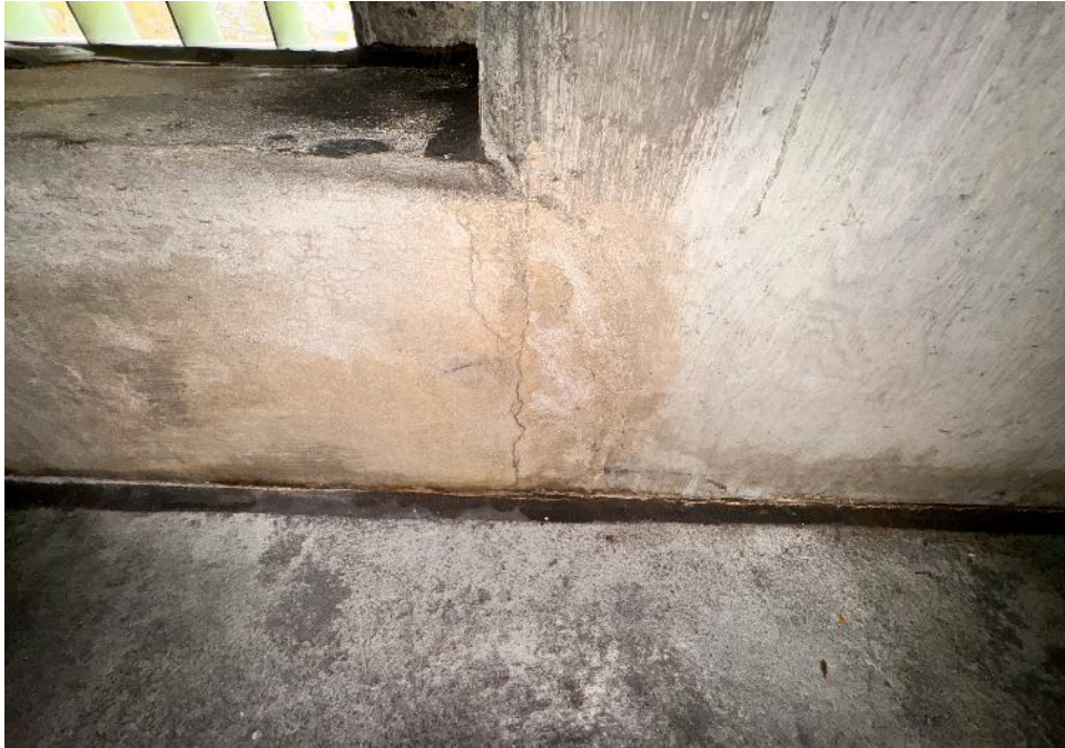
Typical cracks at the garage 2 nd level
