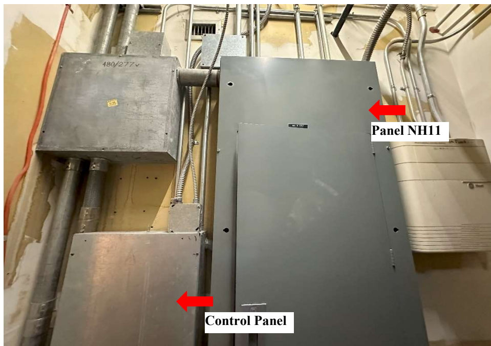
Panel NH11 and Relay Control Panel
