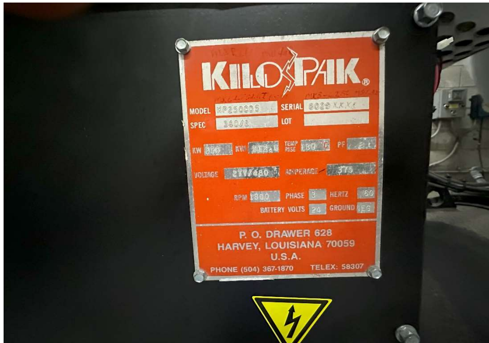
Generator Room Layout Nameplate -
