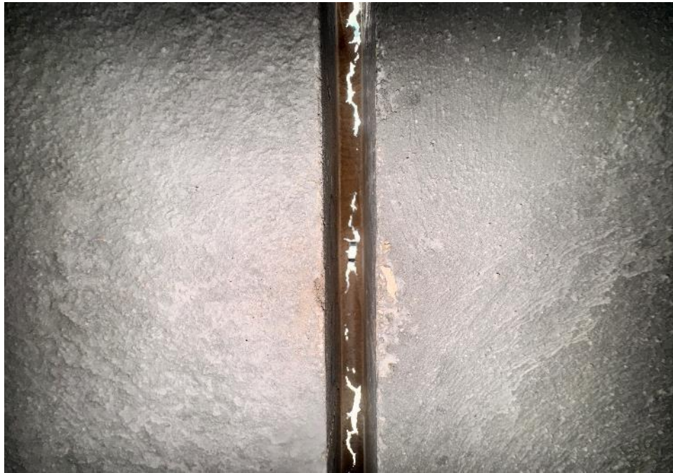
Close-up typical view of deteriorated sealant from the interior
