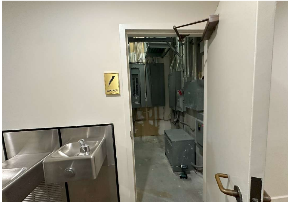
8 TH Floor Electrical Room
