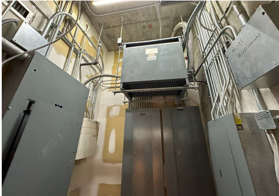
Transformer T112 – 75KVA
