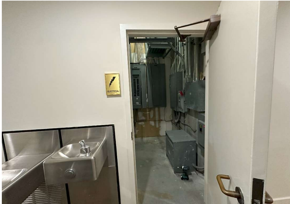
8 TH Floor Electrical Room
