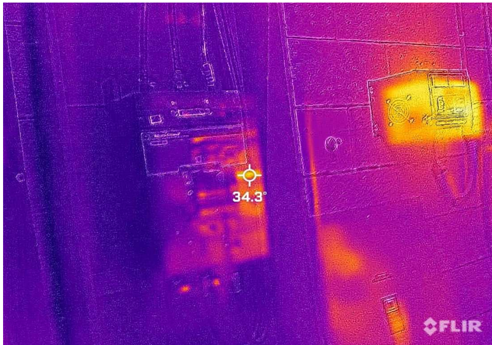
Item 20: Fire Pump Disconnect at 34.3 Degrees Celsius (delta 9.3C)
