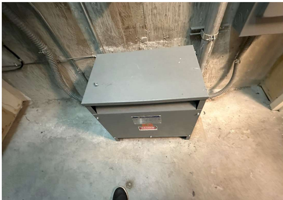
Transformer T111 – 30KVA
