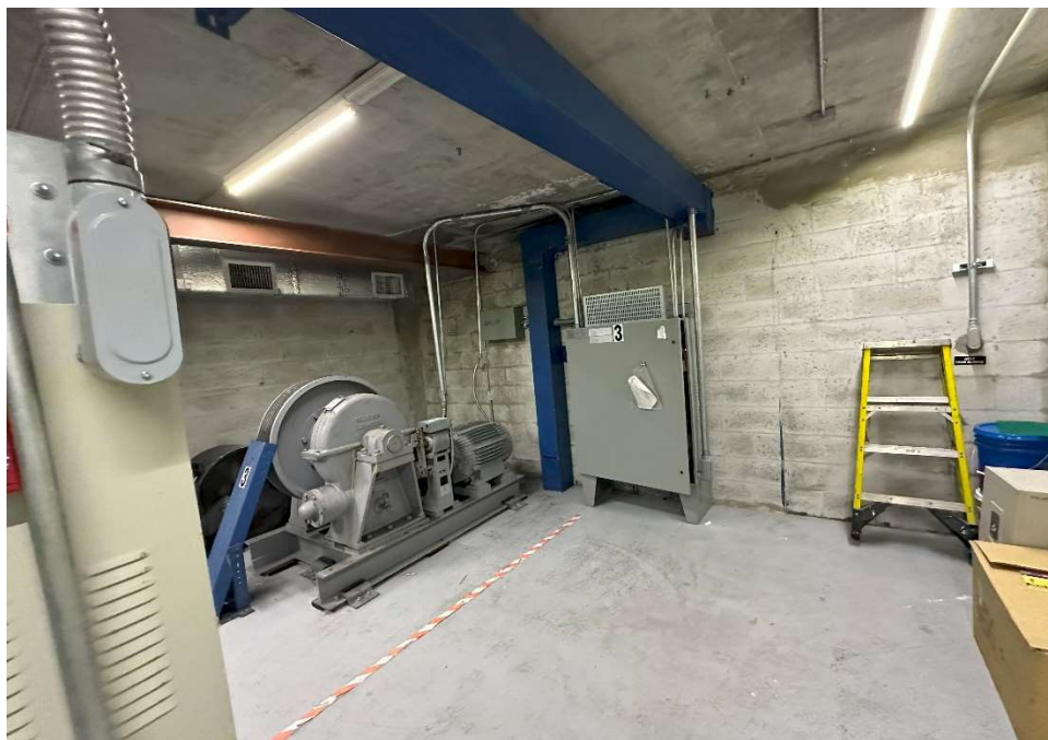
Elevator Machine Room – Elevators 1,2 & 3
