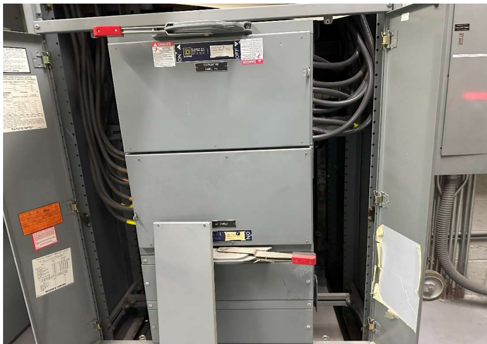
Main 4 of 5 Opened – 400 Amps – Panel NH
