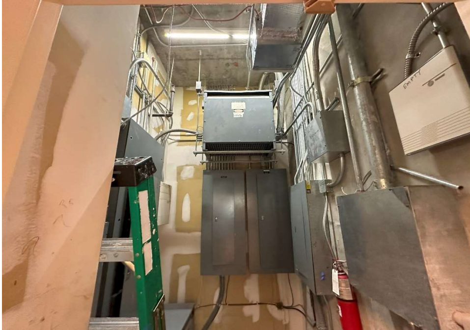
11 th Floor Electrical Room -
