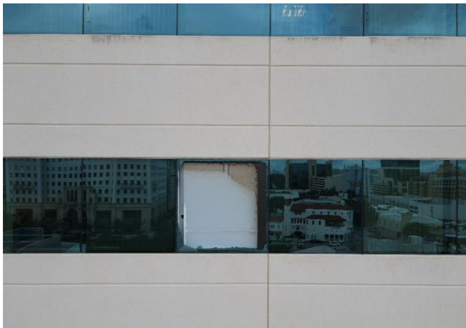
Broken window at the east elevation
