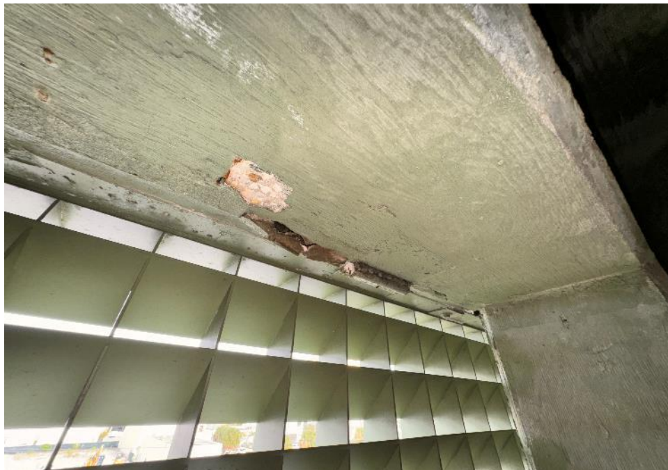
Deteriorated sealant at the top of louvers
