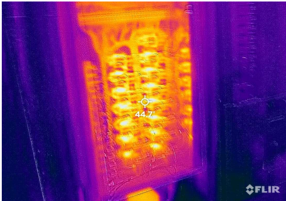
Item 60: Control Panel at 44.7 Degrees Celsius
