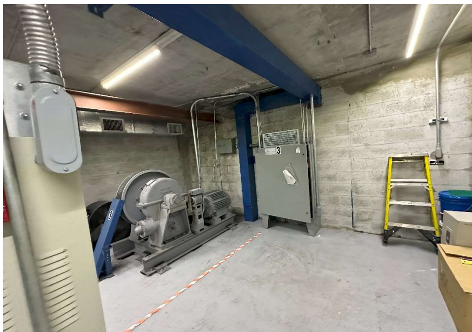
Elevator Machine Room – Elevators 1,2 & 3
