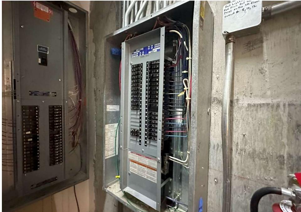
Panel EM3 Opened -
