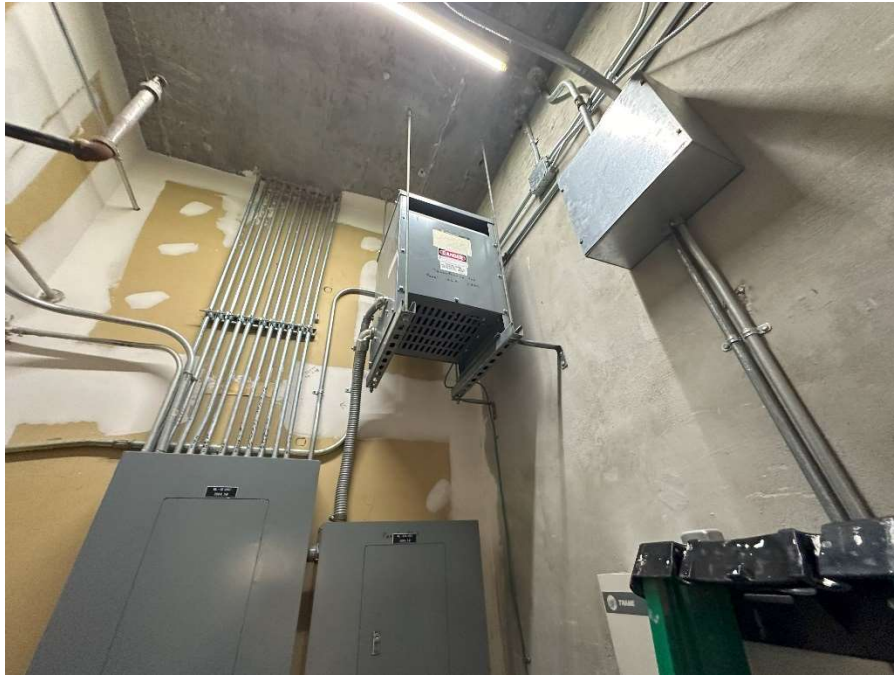
Transformer T102 – 30KVA
