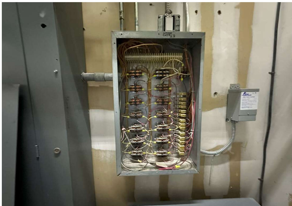
Relay Control Panel Opened -
