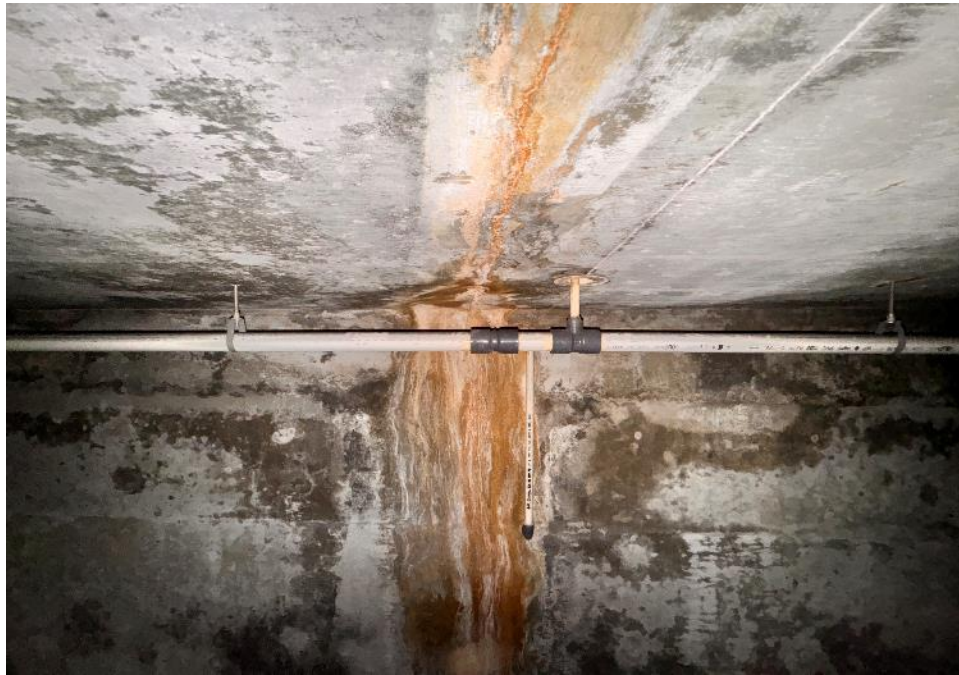
Typical cracks with efflorescence/moisture at the garage basement
