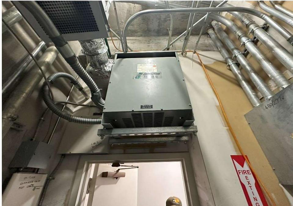
Transformer T81 – 30KVA
