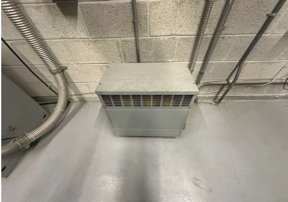
Transformer T3 – 30KVA – 480-208Y/120V
