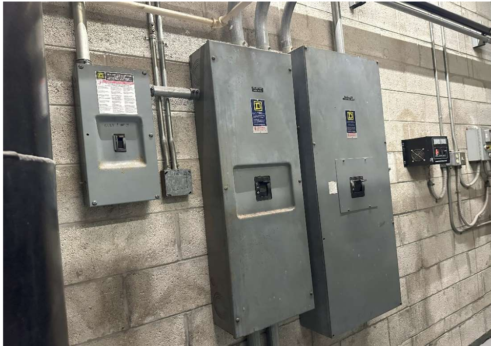
Generator Main Disconnects: Elev 1 of 3, ATS Main, Fire Pump Main
