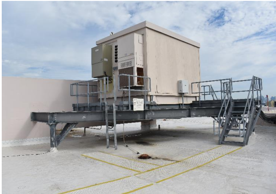
Additional roof top equipment
