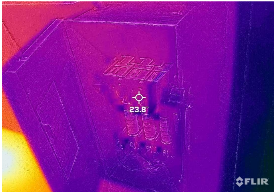
Item 43: Disconnect at 23.8 Degrees Celsius (delta 0.8C)
