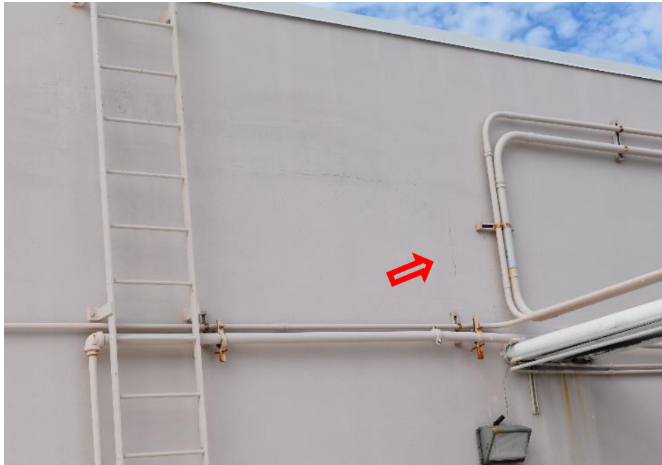
Typical stucco cracks at the exterior of the roof equipment room
