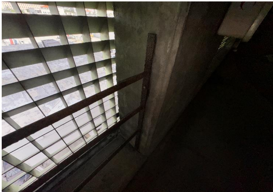
Typical corroded parking barrier cable
