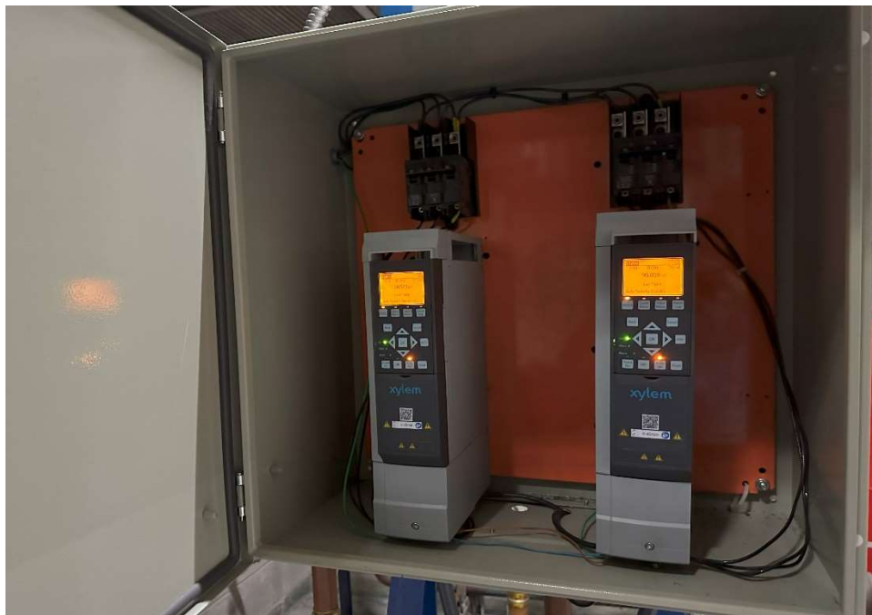
Fire Pump VFD's
