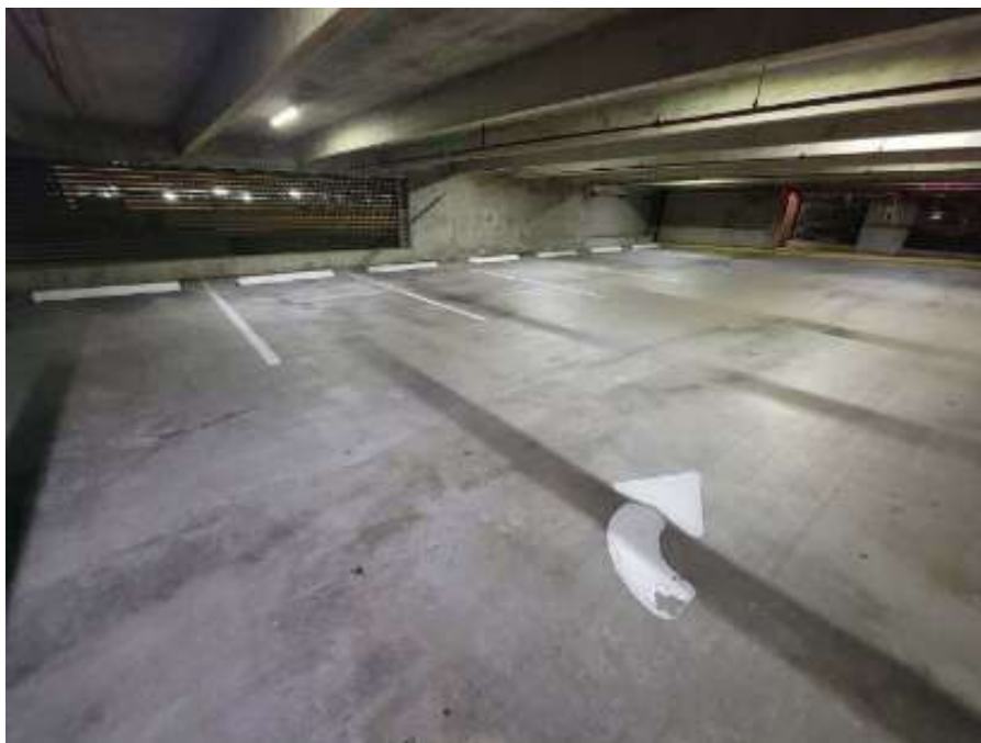
Parking Lot lighting, Typical for Floors Ground Through 7 –
