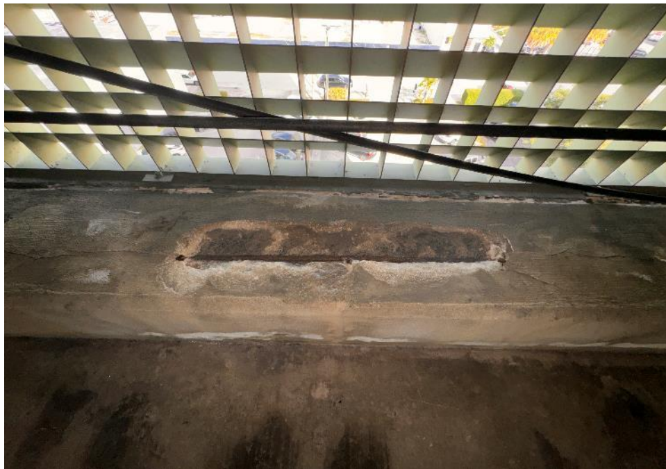
Spalling and exposed rebar at the garage level
