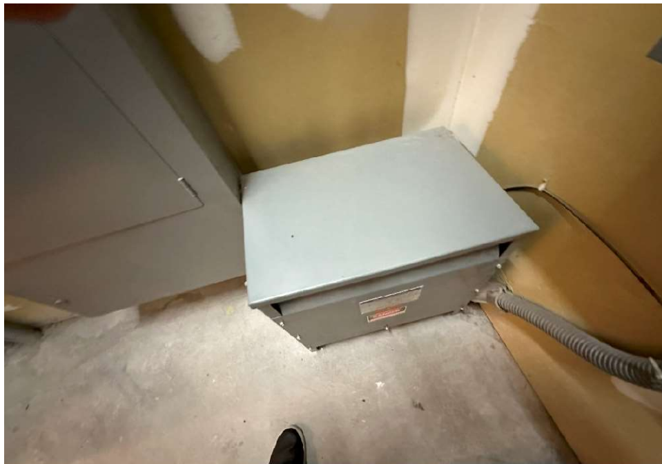
Transformer T101 – 30 KVA
