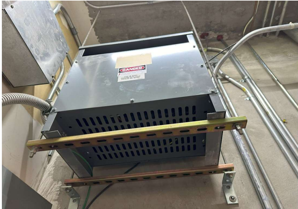
Transformer T91 – 30KVA
