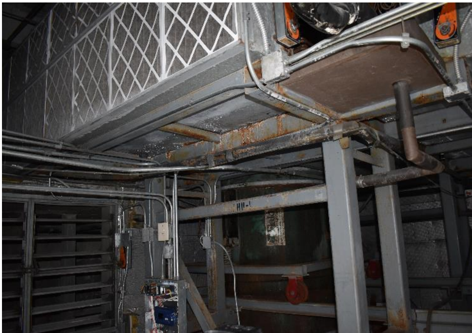
Corroded steel supports for the roof equipment
