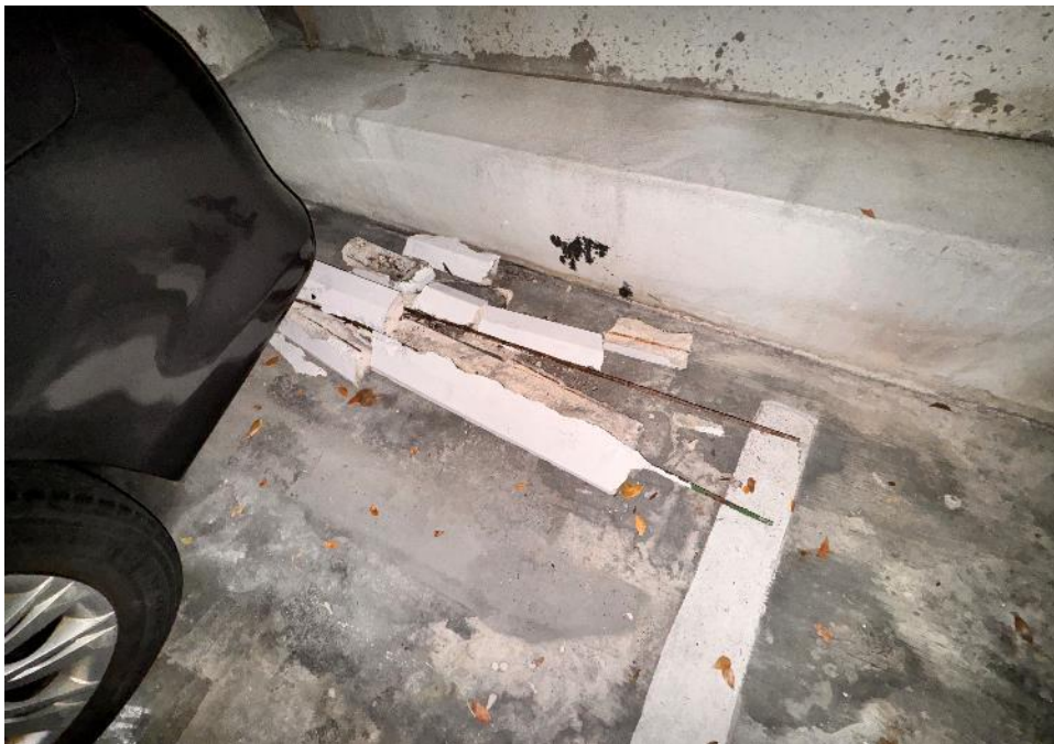
Broken concrete parking curb
