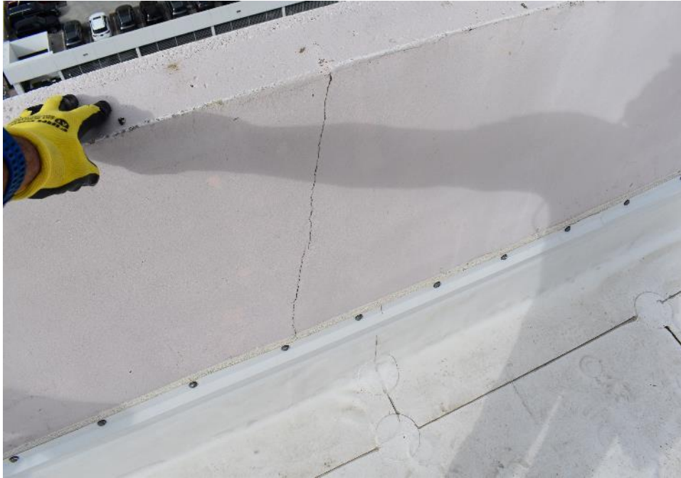
Additional cracks at the parapet walls
