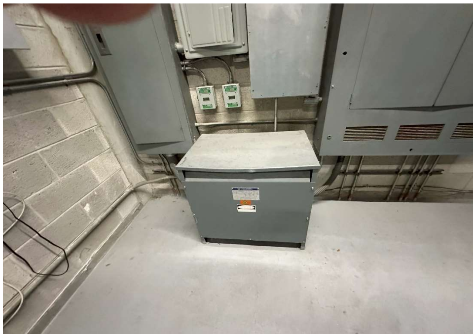
Transformer T2 – 75KVA – 480-208Y/120V
