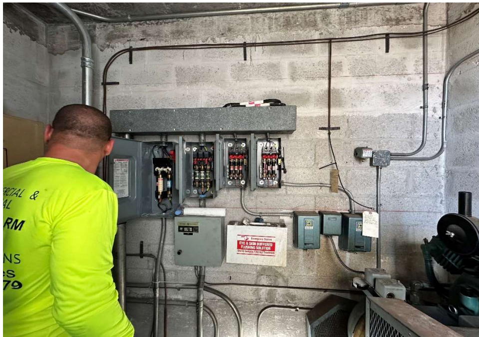
Elevator Disconnects Opened -
