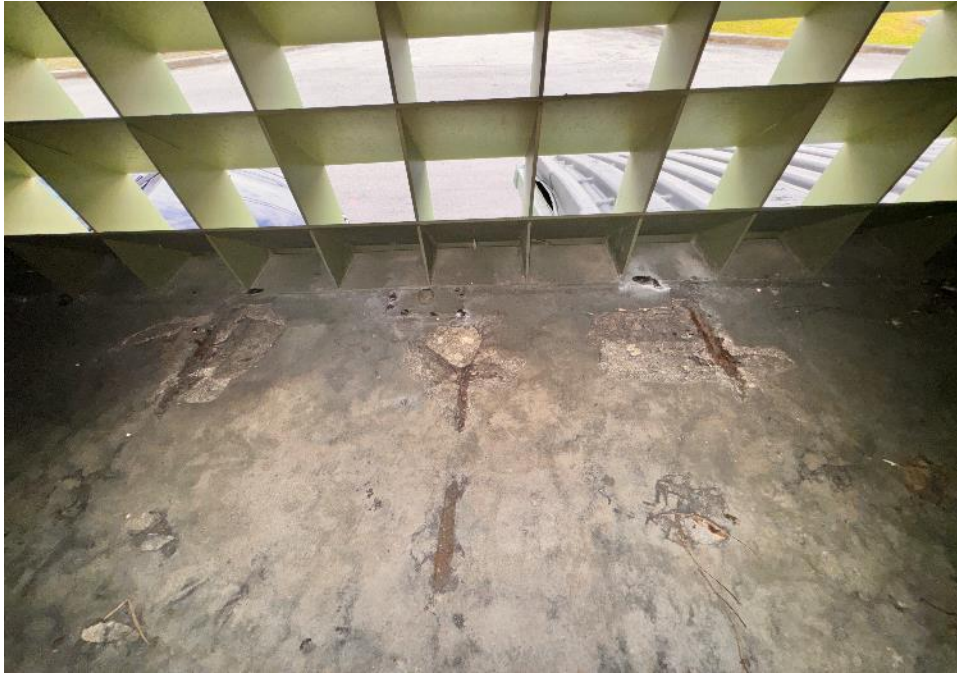
Typical spalling and exposed rebar near the louvers at garage 2 nd level
