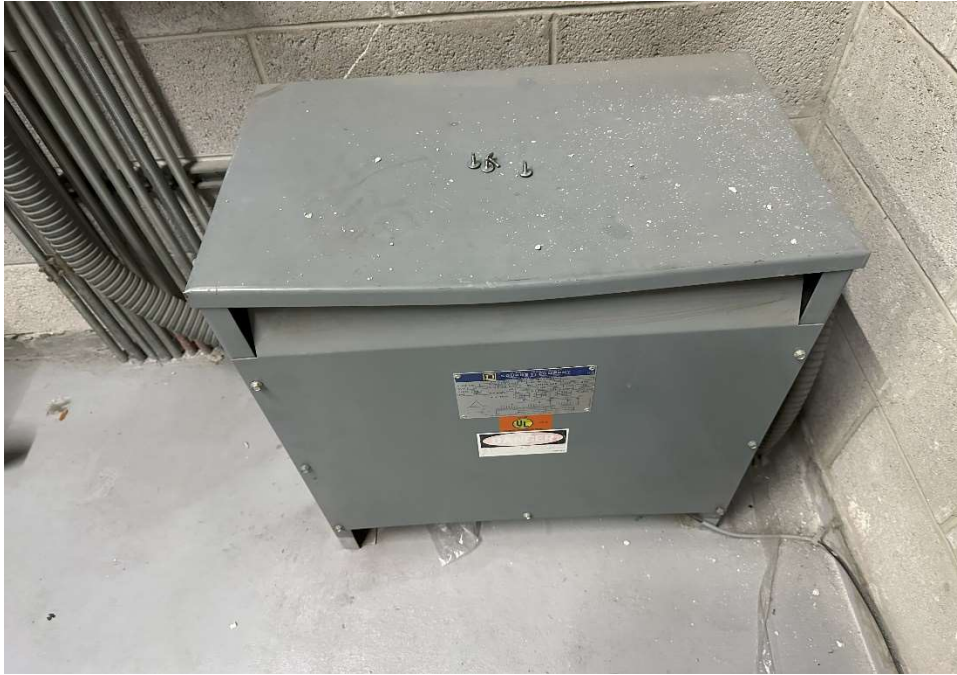
Transformer T1 – 45KVA – 480-208Y/120V
