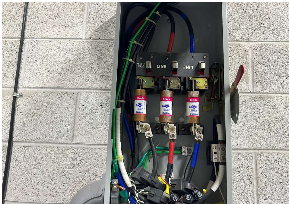
Transformer Disconnect Opened -
