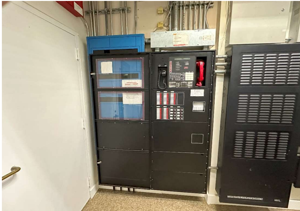
Fire Alarm Control Panel (FACP)
