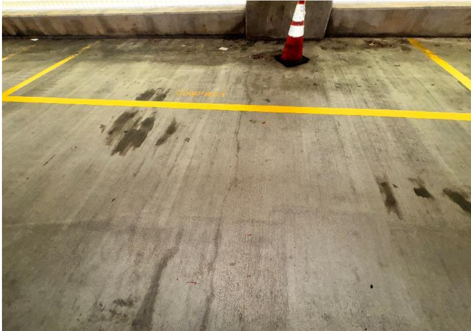
Typical linear cracks in the concrete decking at the garage levels
