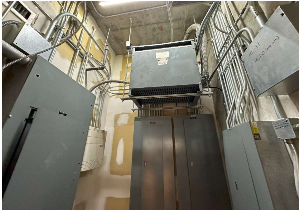
Transformer T112 – 75KVA
