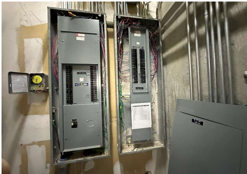
Panels NL12L and NL12R Opened -
