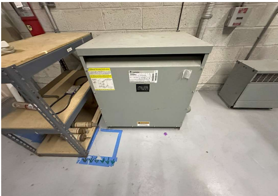
Transformer T4 – 75KVA – 480-208Y/120V
