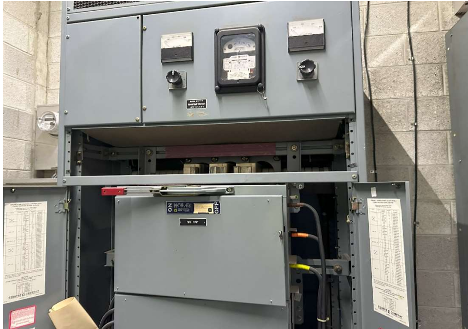
Main 1 of 5 Opened – 600 Amps – Emergency Main – Fire Pump
