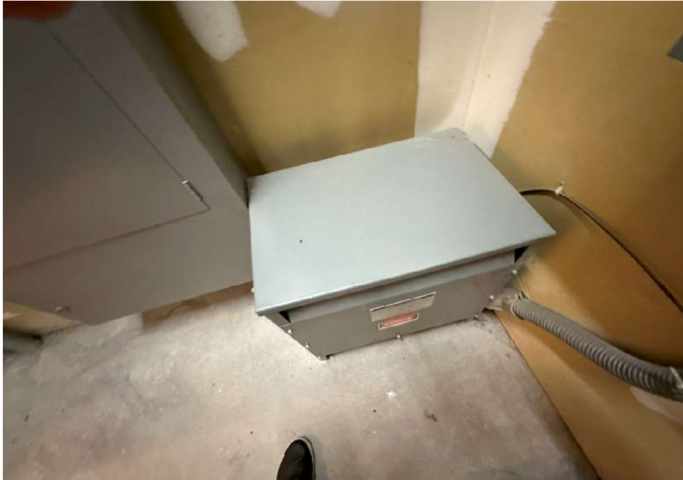
Transformer T101 – 30 KVA
