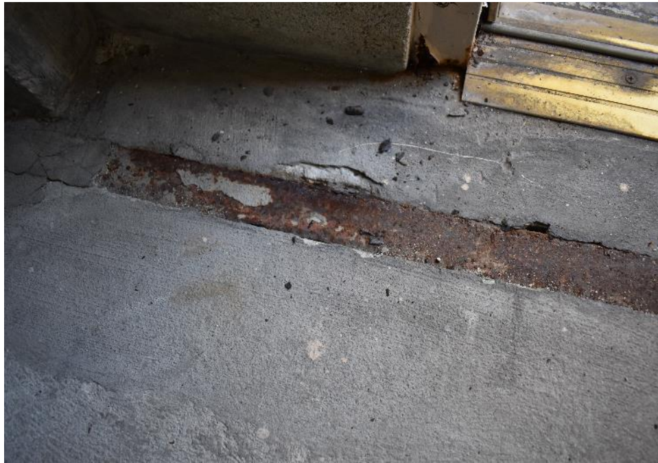
Typical corrosion at the landing near the exit doors
