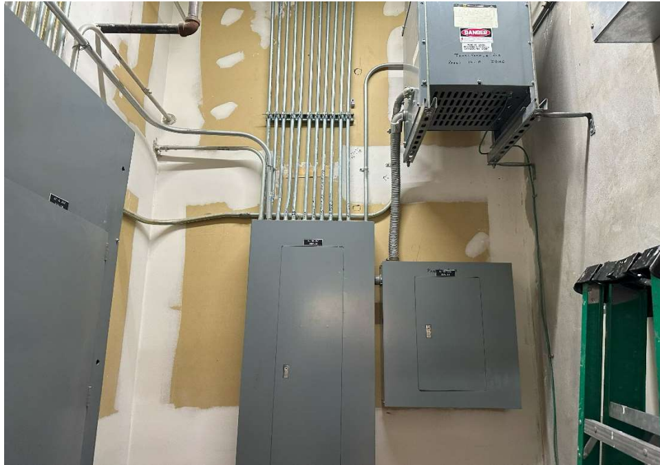
10 th Floor Electrical Room
