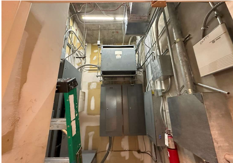
11 th Floor Electrical Room -
