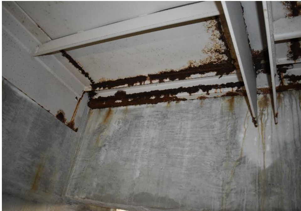
Typical corrosion on the underside of the metal stairs
