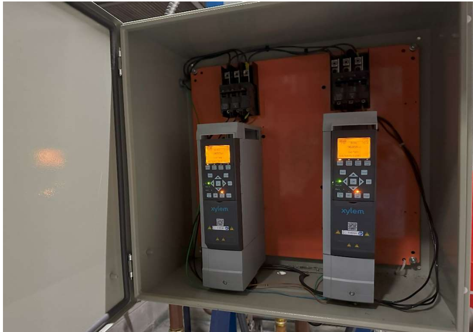
Fire Pump VFD's
