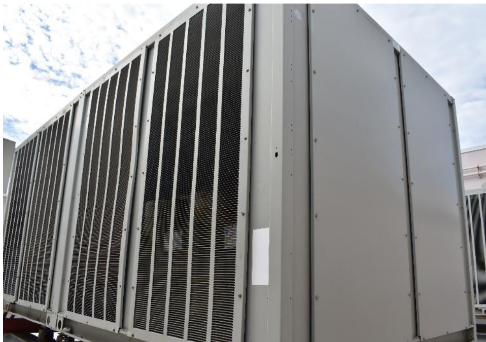
Additional roof top equipment
