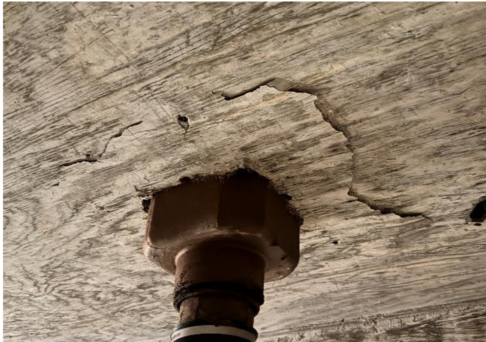
Spalling at the garage level
