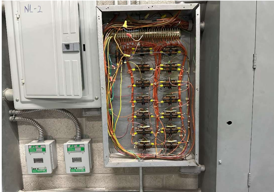
Control Cabinet Opened -
