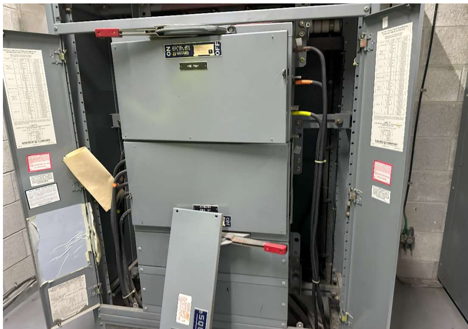
Main 2 of 5 Opened – 400 Amps – Emergency Main – Panel EDP
