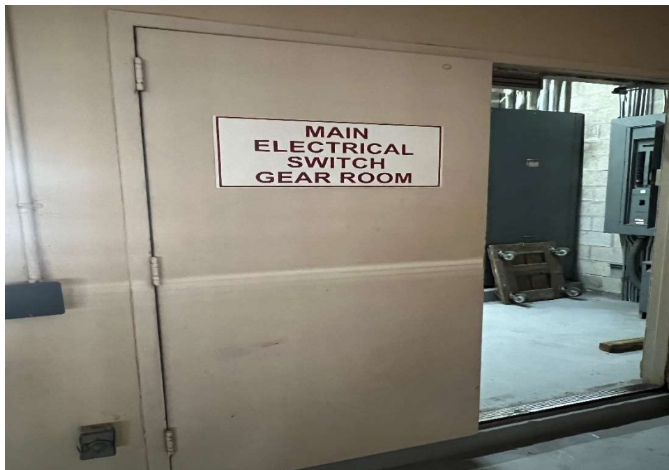
Service Entrance – Main Electrical Switchgear Room -
