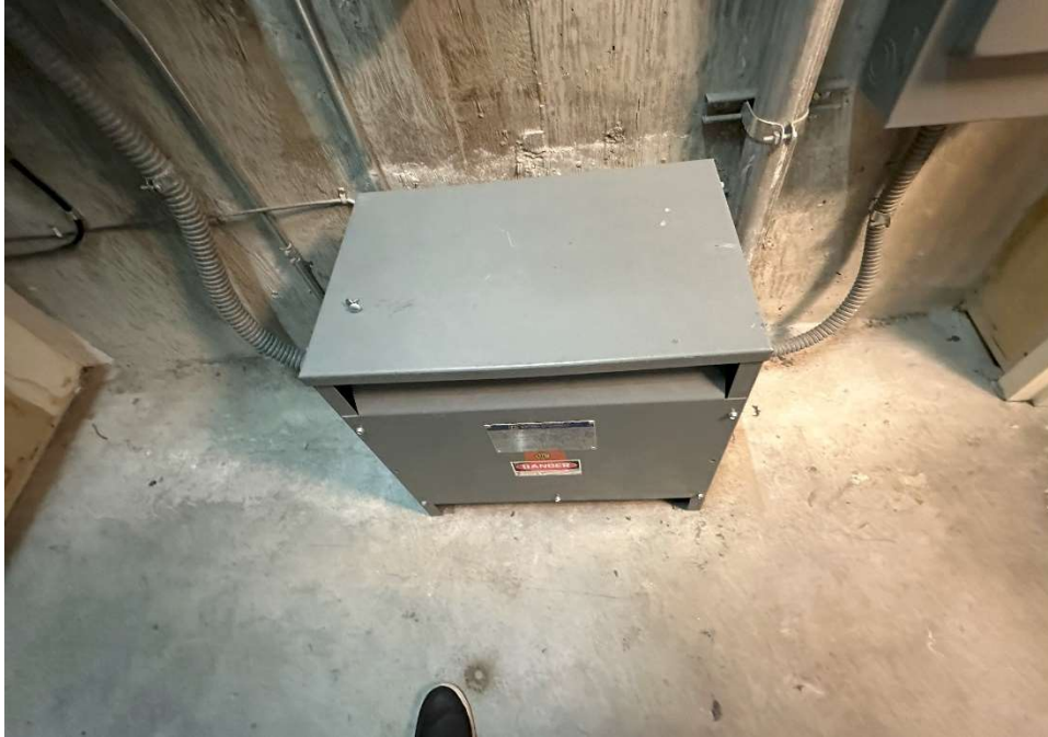
Transformer T121 – 75KVA
