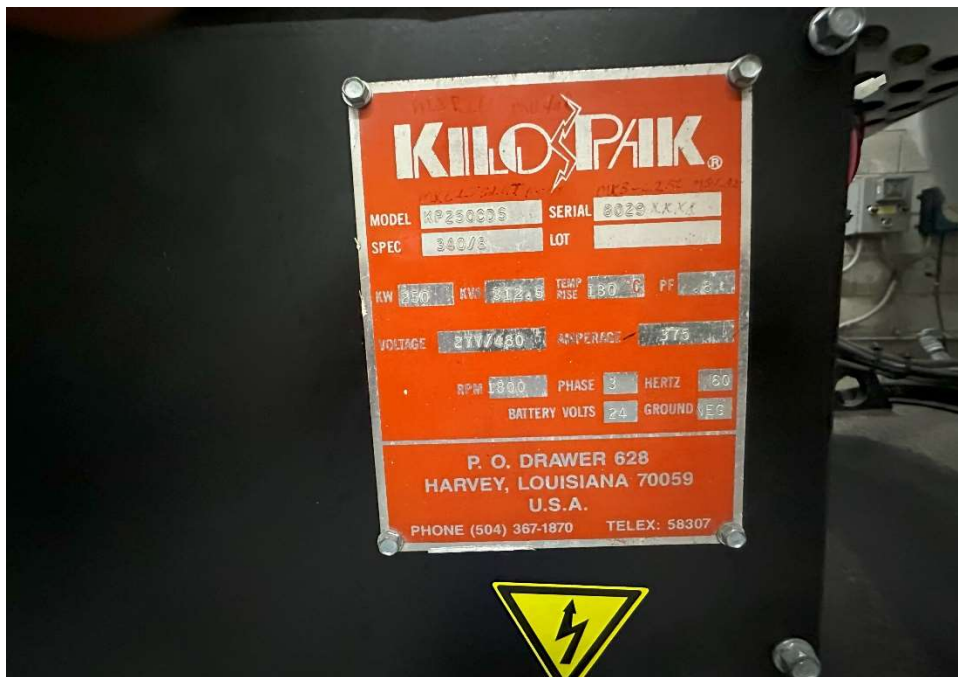
Generator Room Layout Nameplate -
