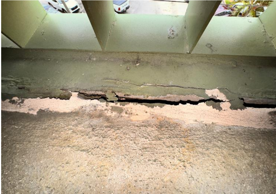
Deteriorated sealant at the bottom of louvers
