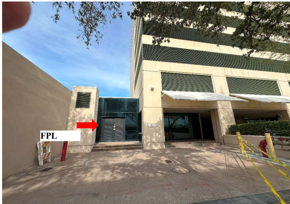
FPL Service: 3 Phase 277/480V, 4 Wire
