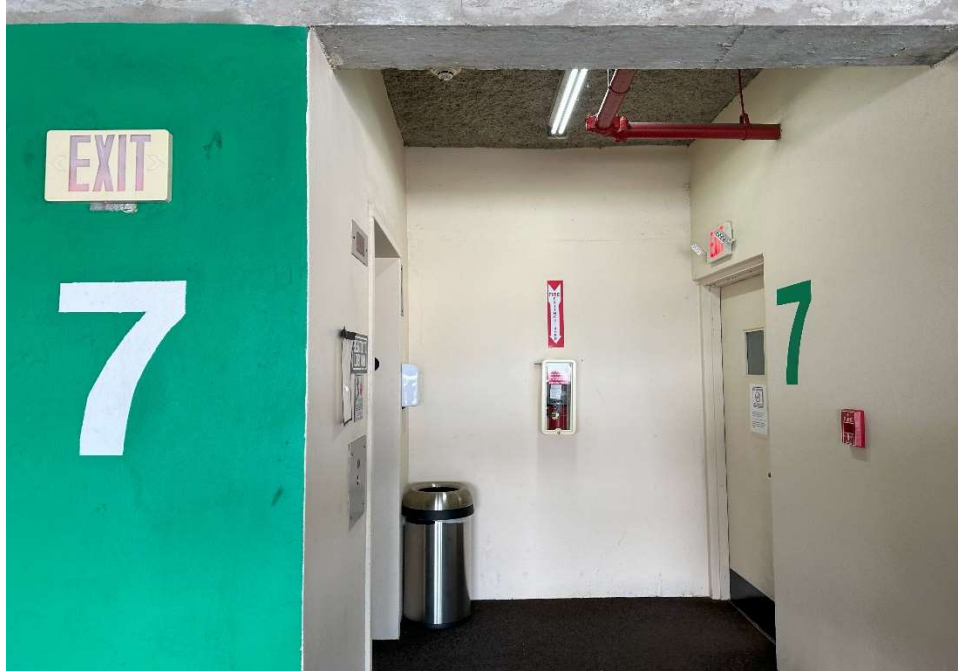
Emergency/Exit Lighting, Typical of garage Floors
