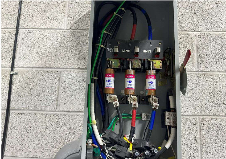
Transformer Disconnect Opened -
