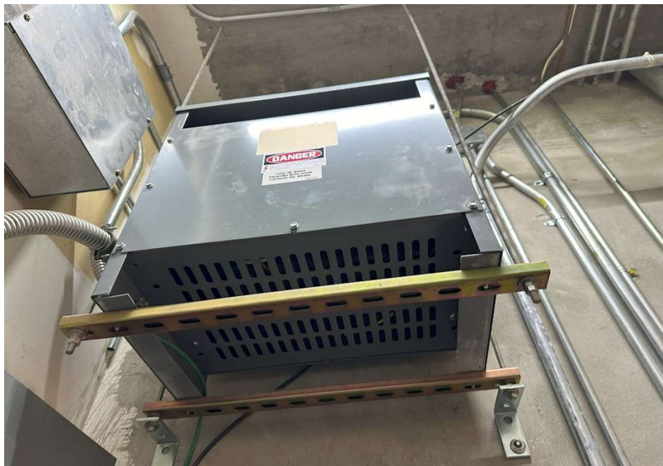
Transformer T91 – 30KVA
