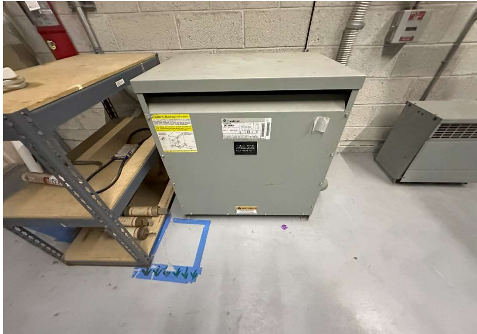
Transformer T4 – 75KVA – 480-208Y/120V
