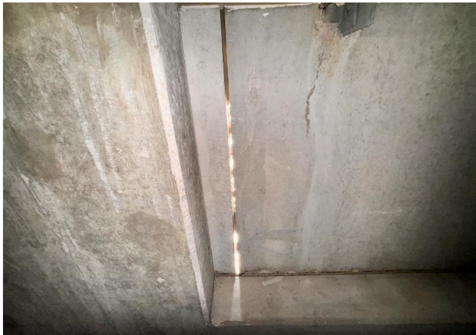
Typical view of deteriorated sealant from the interior
