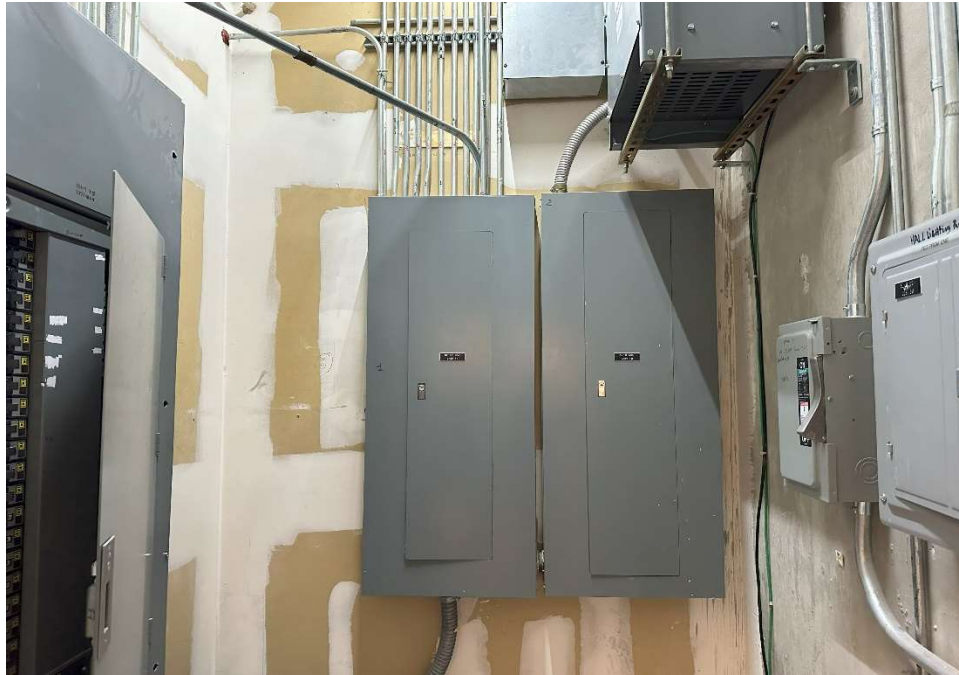
9 th Floor Electrical Room -
