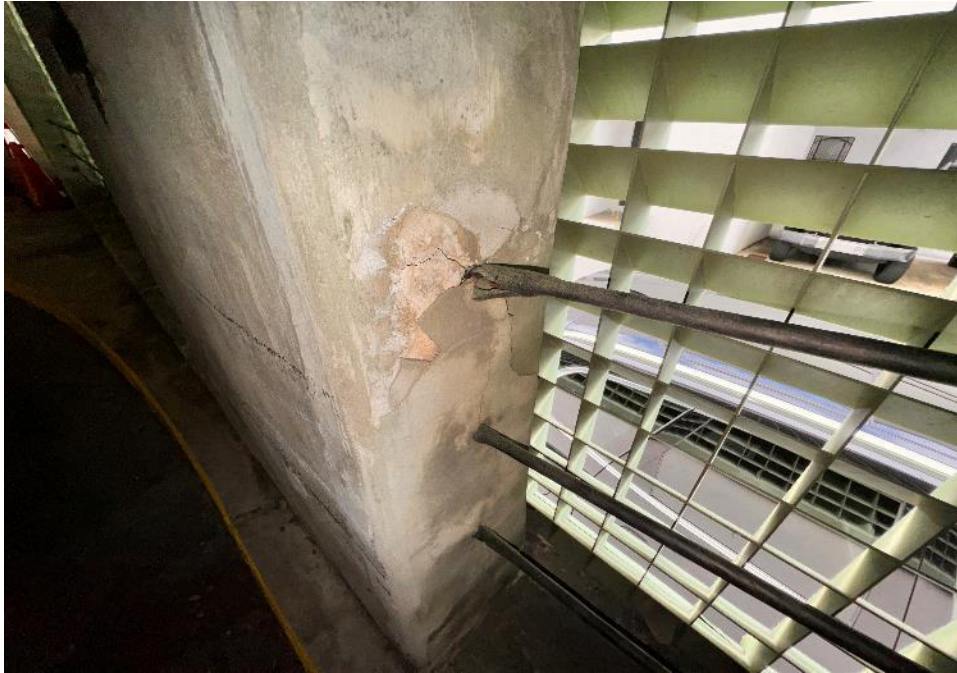
Spalling at the barrier cable to concrete connection
