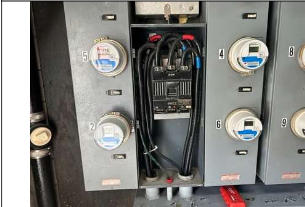
13. Wires and cables
