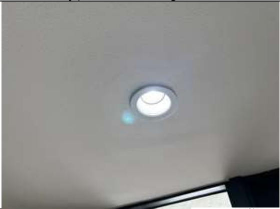
19. Building egress illumination
