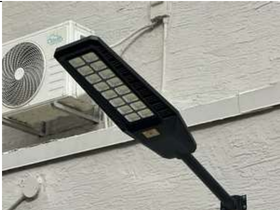
19. Building egress illumination
