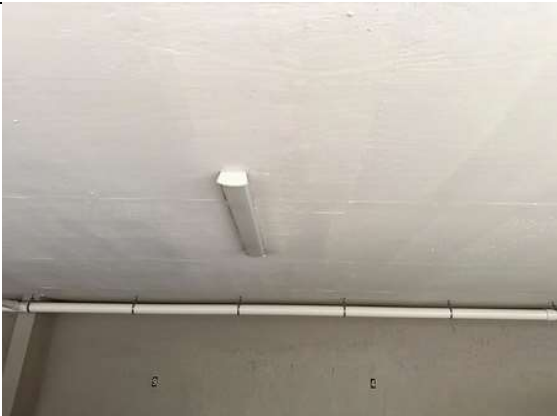
19. Building egress illumination
