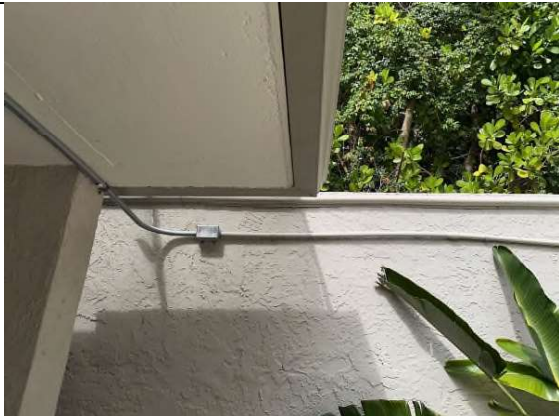
24. Wiring in open or under cover parking garage areas
