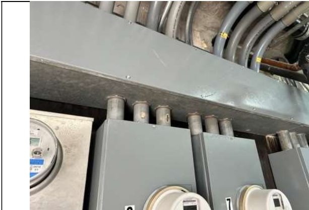
12. Service conductors conduit/raceways
