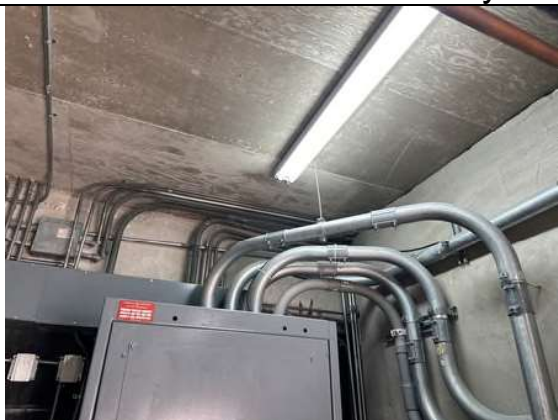
12. Service conductors conduit/raceways
