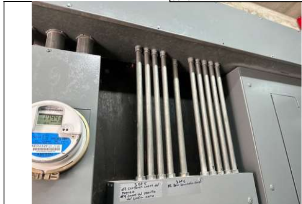
12. Service conductors conduit/raceways
