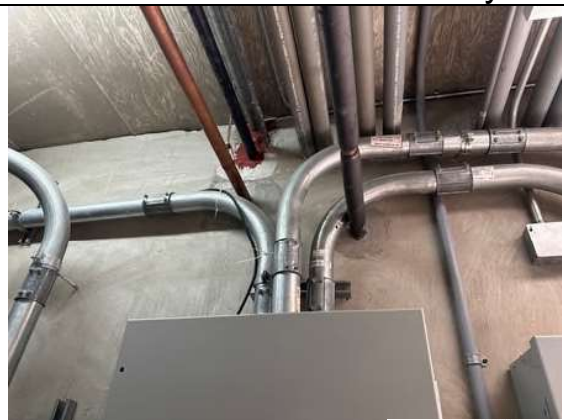
12. Service conductors conduit/raceways
