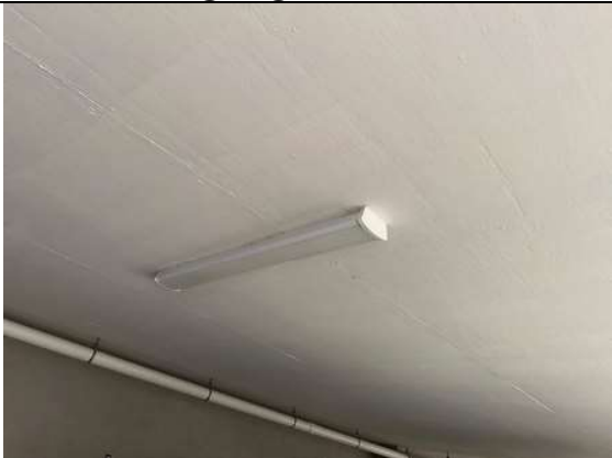
19. Building egress illumination
