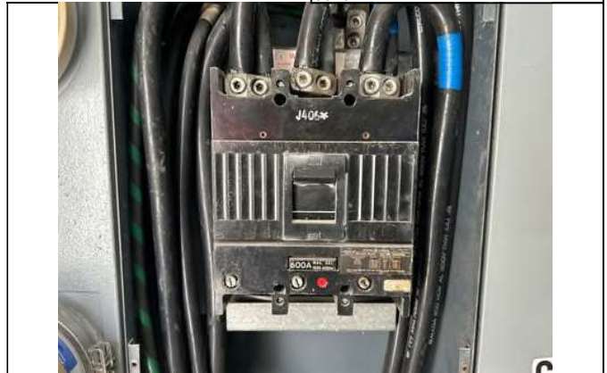
13. Wires and cables
