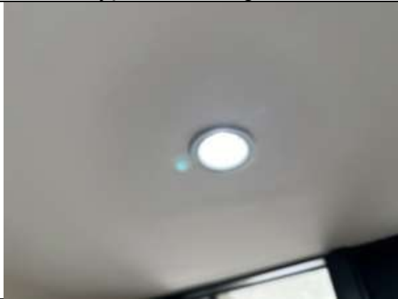
19. Building egress illumination
