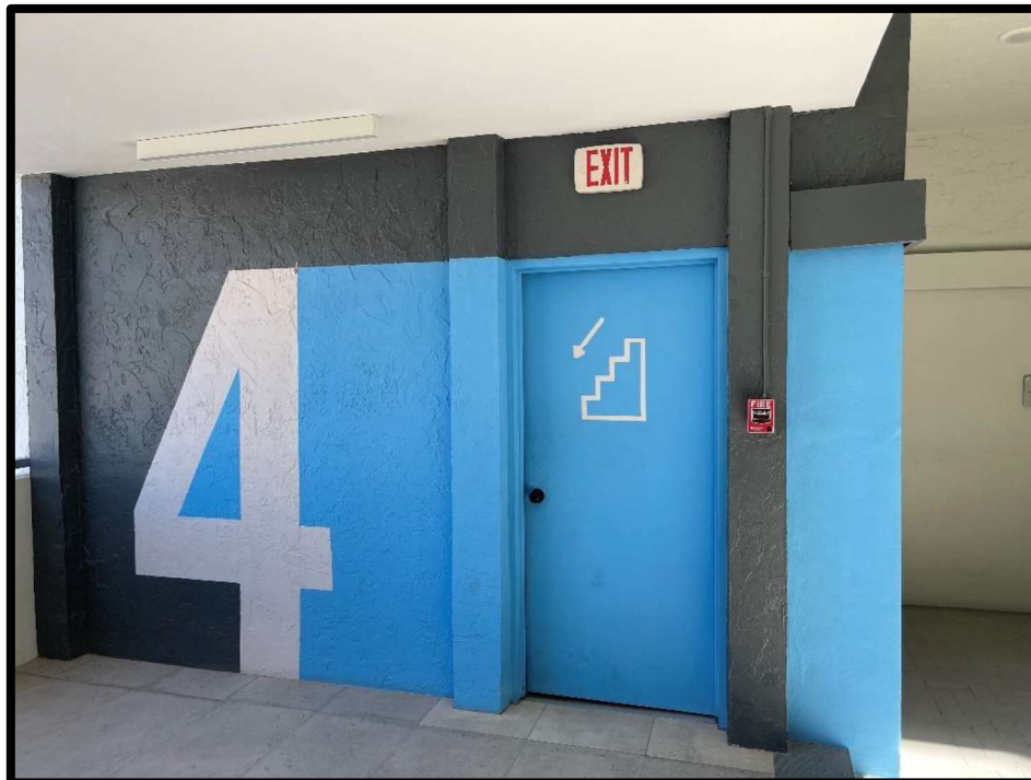
Photograph #135 Exit sign lights outdoor day time at 4th floors in the building in good working condition.
