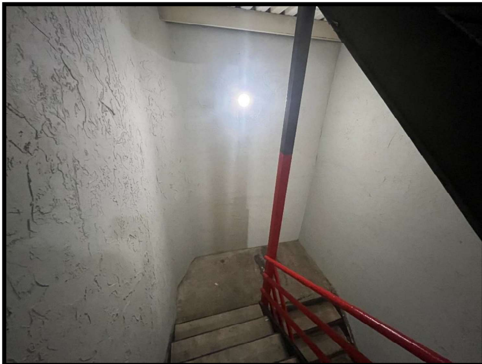
Photograph #171 The stairway landing properly illuminated.
