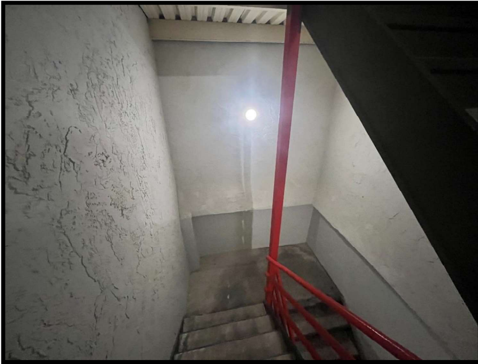
Photograph #168 The stairway landing properly illuminated.
