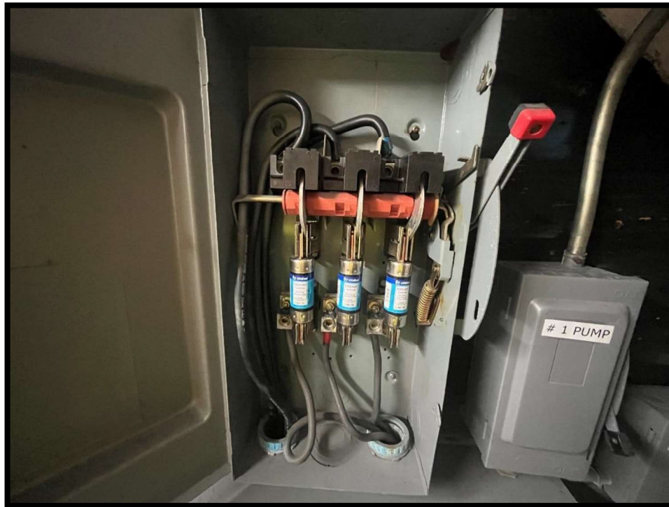
Photograph #67 Phases are properly identified and installed. Fuses are properly identified and installed.
