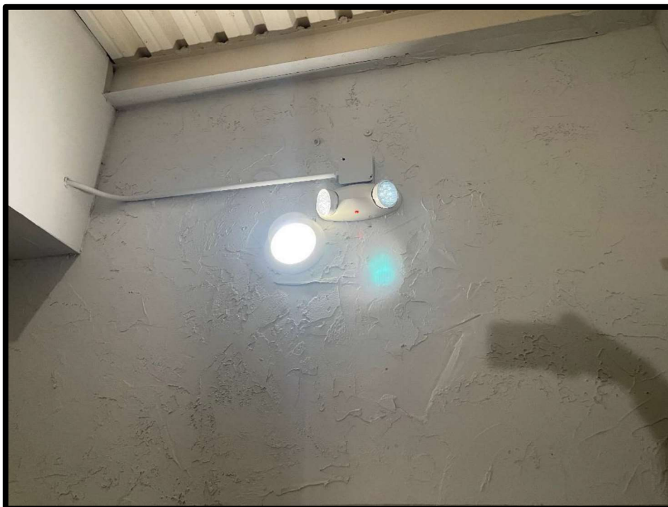
Photograph #211 Emergency light Properly installed and in good condition.
