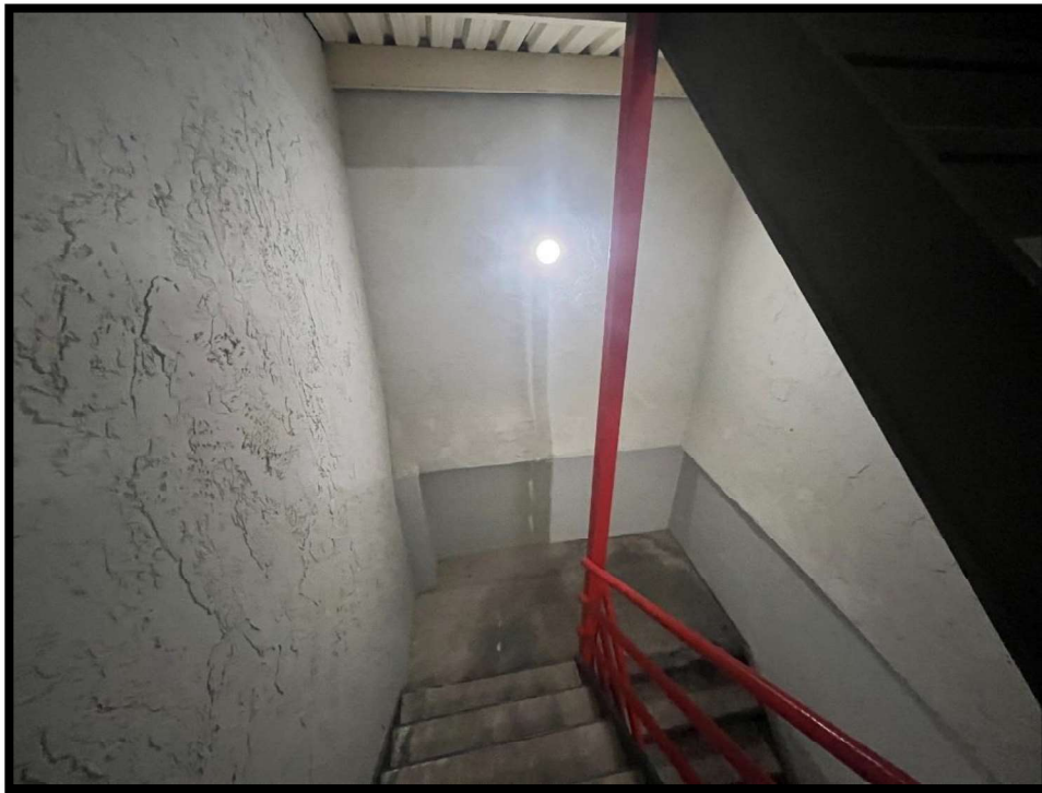
Photograph #168 The stairway landing properly illuminated.
