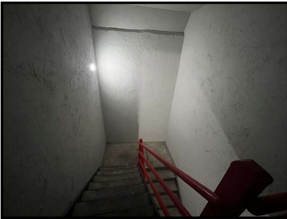
Photograph #165 The stairway landing properly illuminated.
