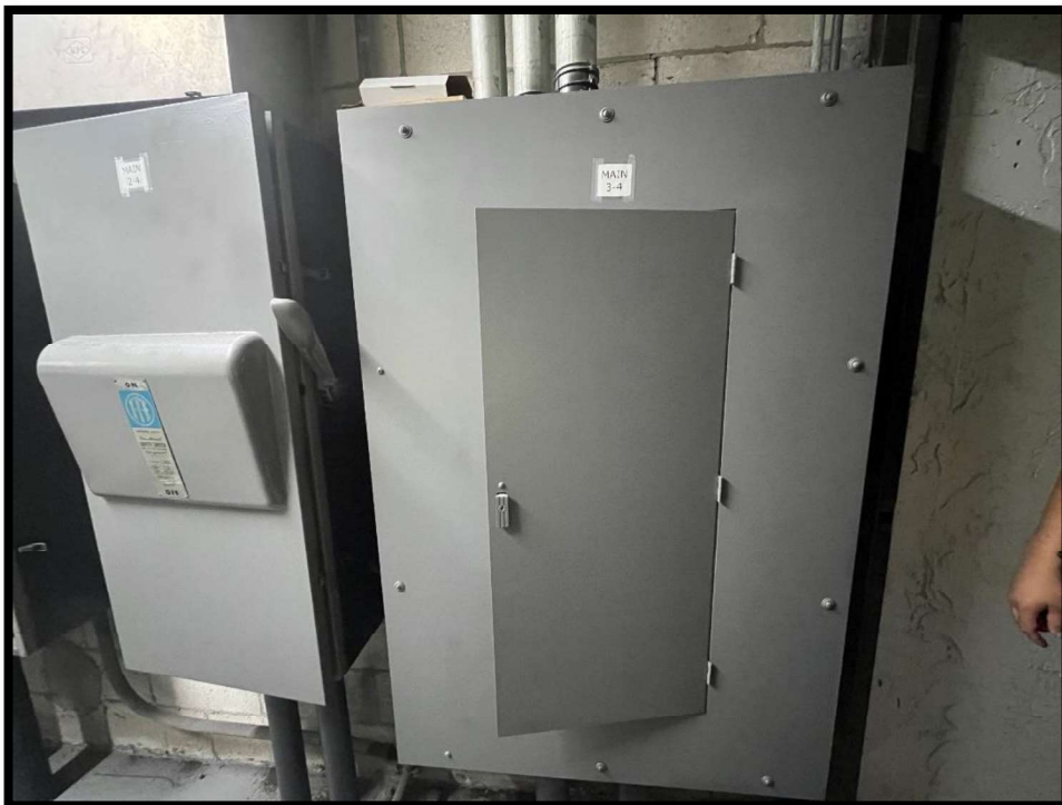
Photograph #9 The Main Panel 3-4 (800A) Branch circuits properly identified. The label shall be of sufficient durability to withstand the environment involved and shall not be handwritten. NEC 210.5 C (1) (b). In the 2020 NEC, Section 705.10, Section 11.12.2.1.5 in NFPA 1.
