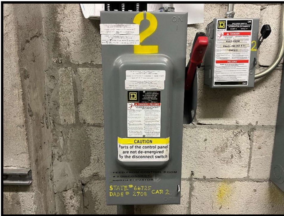
Photograph #48 The Disconnect #2 North Elevator is properly identified. The label shall be of sufficient durability to withstand the environment involved and shall not be handwritten. NEC 210.5 C (1) (b). In the 2020 NEC, Section 705.10, Section 11.12.2.1.5 in NFPA 1.
