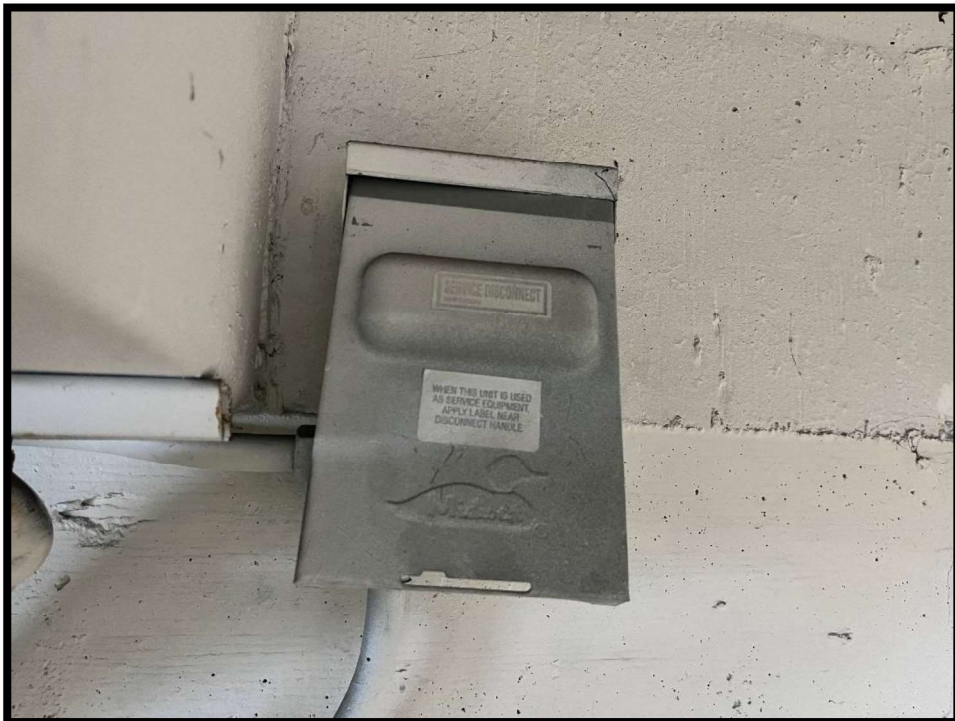
Photograph #60 AC Disconnect properly identified.
