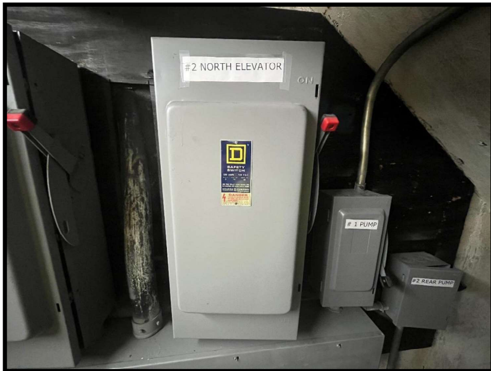
Photograph #66 The Disconnect #2 North Elevator is properly identified. The label shall be of sufficient durability to withstand the environment involved and shall not be handwritten. NEC 210.5 C (1) (b). In the 2020 NEC, Section 705.10, Section 11.12.2.1.5 in NFPA 1.
