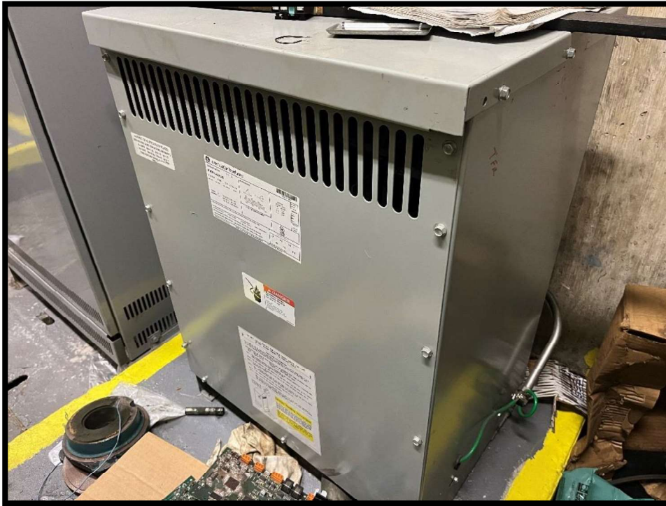
Photograph #47 Transformer 2 properly installed. Grounding is properly installed.
