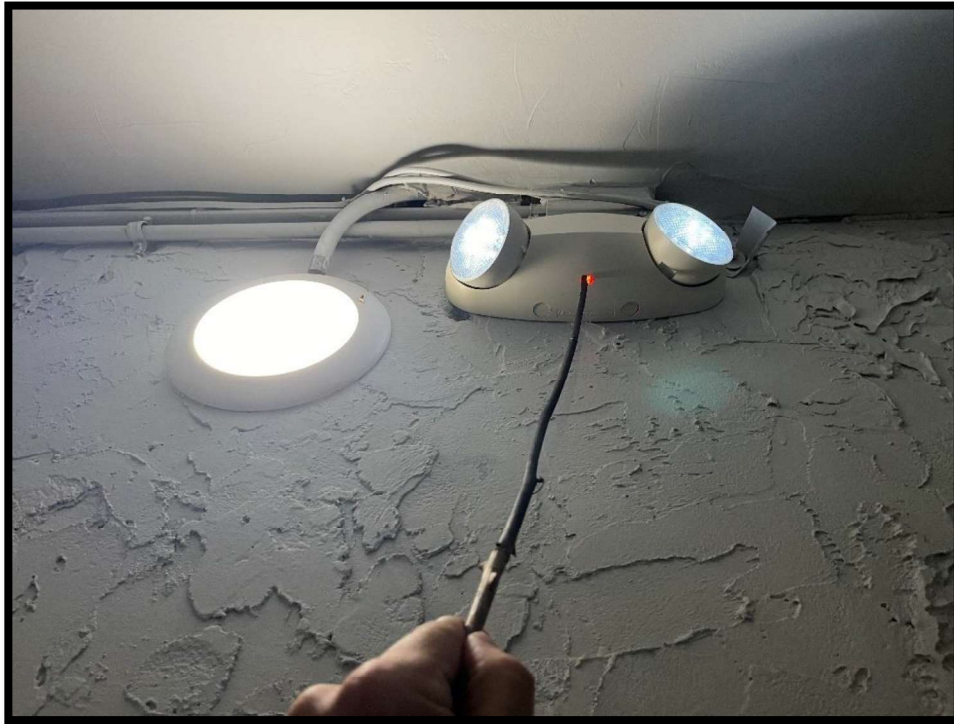
Photograph #170 Emergency lights properly installed and in good working condition.
