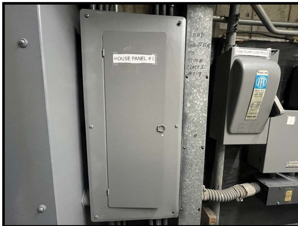
Photograph #17 Re-Inspection 05.20.2024. The Sub-Panel House #1 Branch circuits properly identified. NEC 210.5 C (1) (b). In the 2020 NEC®, Section 705.10, Section 11.12.2.1.5 in NFPA 1.
