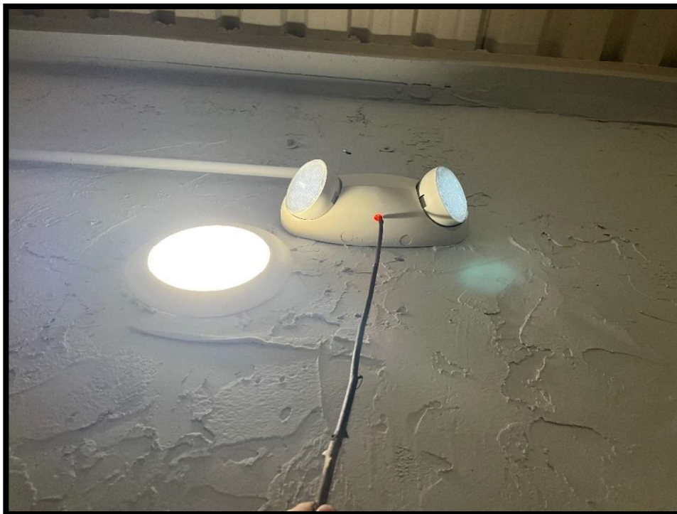
Photograph #173 Emergency lights properly installed and in good working condition.
