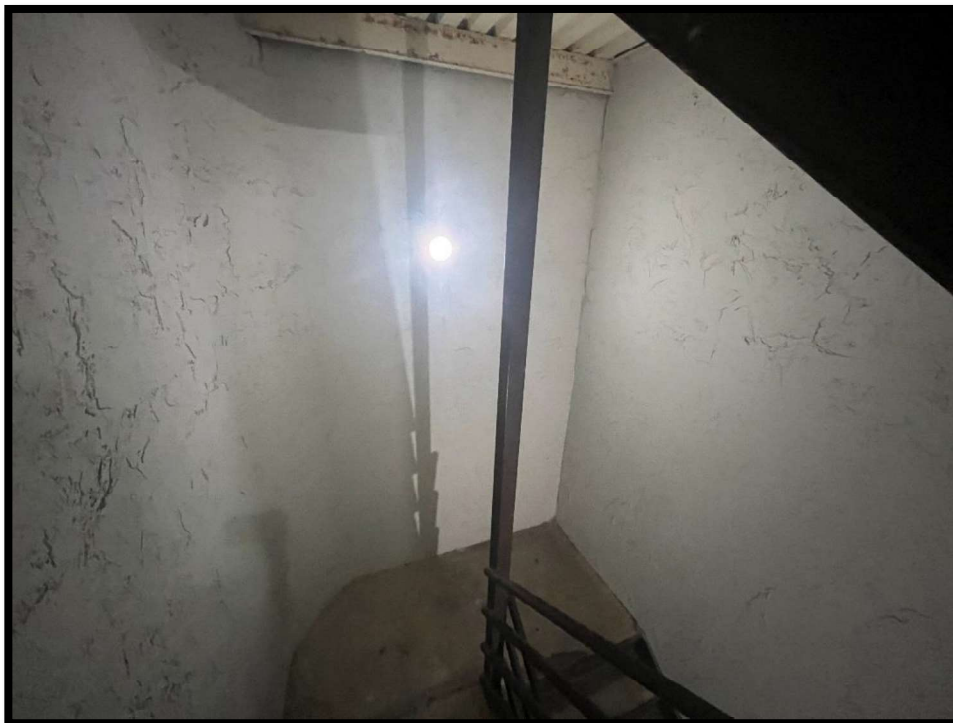
Photograph #181 The stairway landing properly illuminated.
