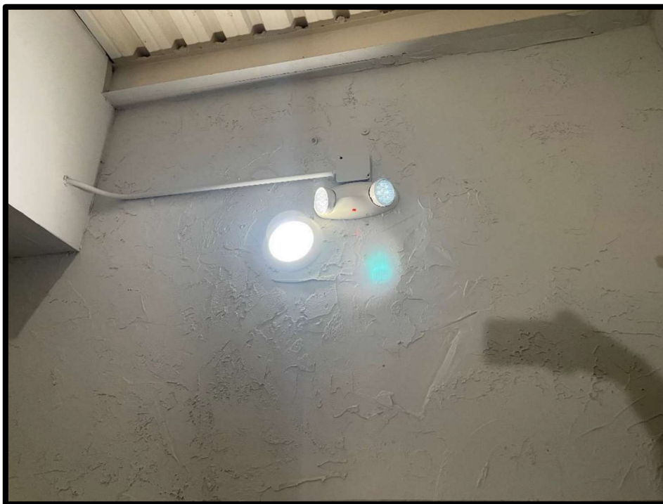
Photograph #211 Emergency light Properly installed and in good condition.
