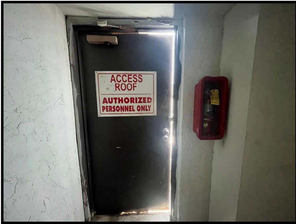
Photograph #153 Roof access is properly identified. Extinguisher is properly installed.
