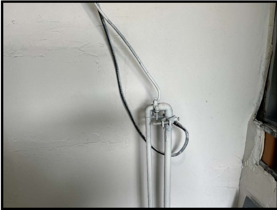
Photograph #97 Ground of the service is properly installed.
