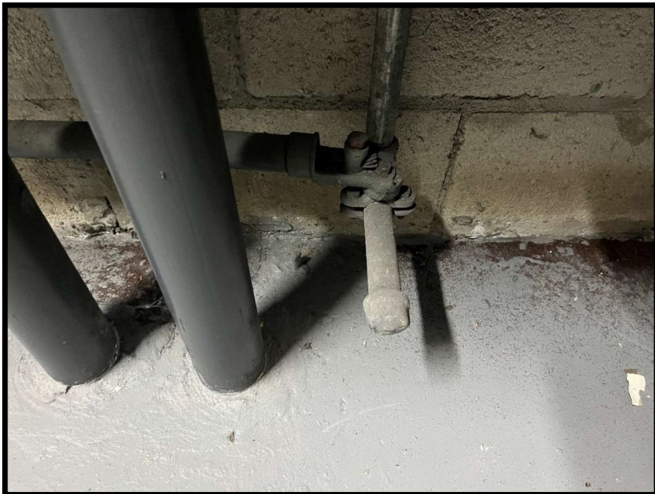
Photograph #36 Ground of the service is properly installed.
