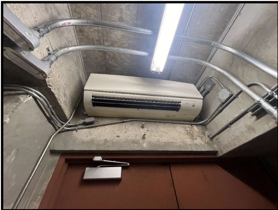
Photograph #58 Mechanical Room properly ventilated.
