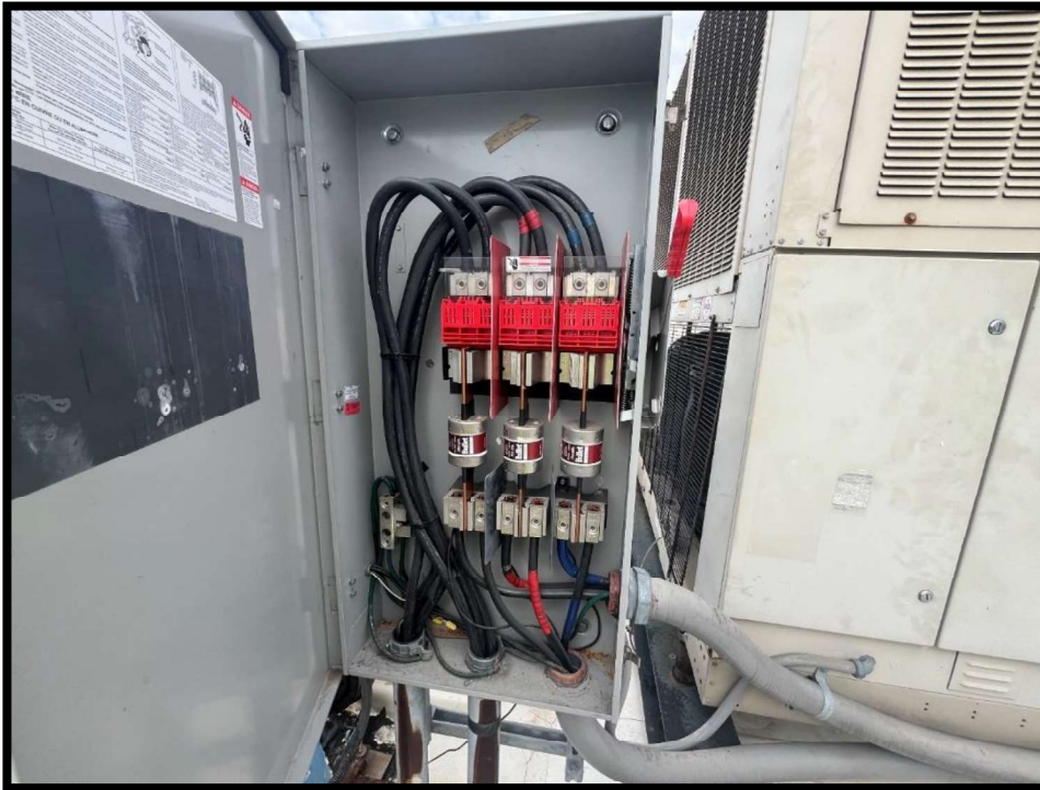
Photograph #157 Phases are properly identified and installed.
