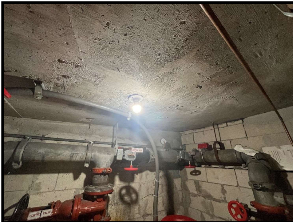
Photograph #80 Electrical Fire Pump Room 2 properly lit.
