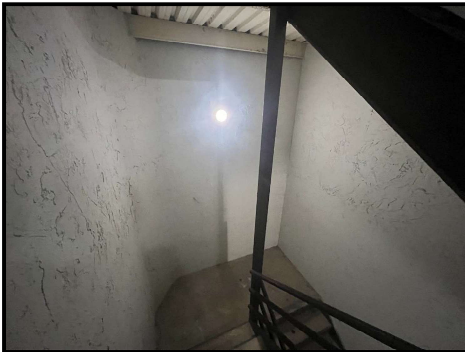
Photograph #179 The stairway landing properly illuminated.
