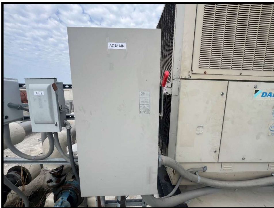
Photograph #156 The Disconnect AC MAIN is properly identified. The label shall be of sufficient durability to withstand the environment involved and shall not be handwritten. NEC 210.5 C (1) (b). In the 2020 NEC, Section 705.10, Section 11.12.2.1.5 in NFPA 1.
