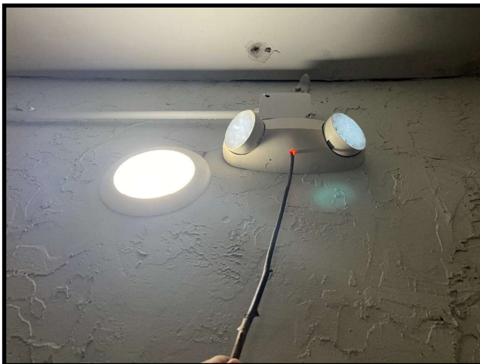
Photograph #167 Emergency lights properly installed and in good working condition.
