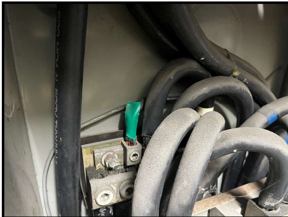
Photograph #5 Ground of the Disconnect is properly installed.
