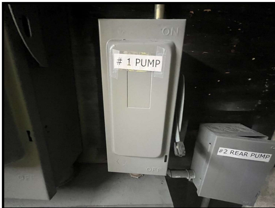
Photograph #68 The Disconnect #1 Pump is properly identified. The label shall be of sufficient durability to withstand the environment involved and shall not be handwritten. NEC 210.5 C (1) (b). In the 2020 NEC, Section 705.10, Section 11.12.2.1.5 in NFPA 1.
