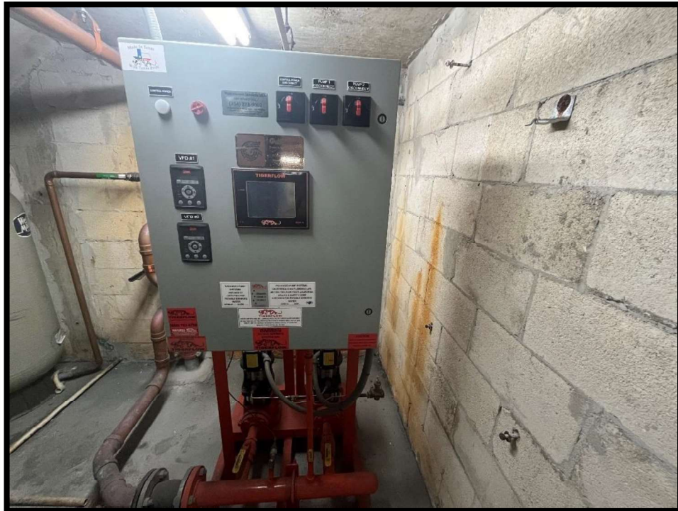
Photograph #74 Fire Pump properly installed and good standing.
