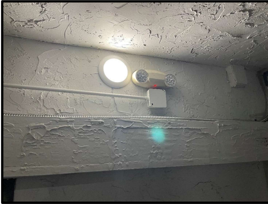
Photograph #210 Emergency light Properly installed and in good condition.
