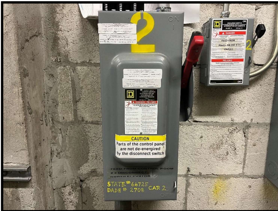
Photograph #48 The Disconnect #2 North Elevator is properly identified. The label shall be of sufficient durability to withstand the environment involved and shall not be handwritten. NEC 210.5 C (1) (b). In the 2020 NEC, Section 705.10, Section 11.12.2.1.5 in NFPA 1.
