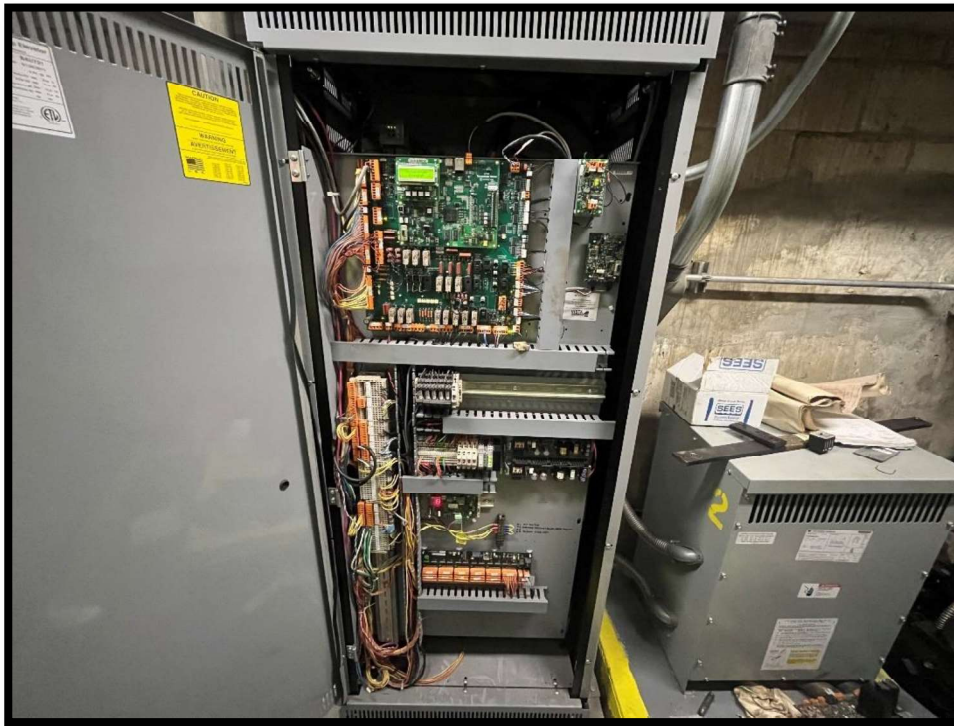
Photograph #45 Elevator Machine 1 properly installed.
