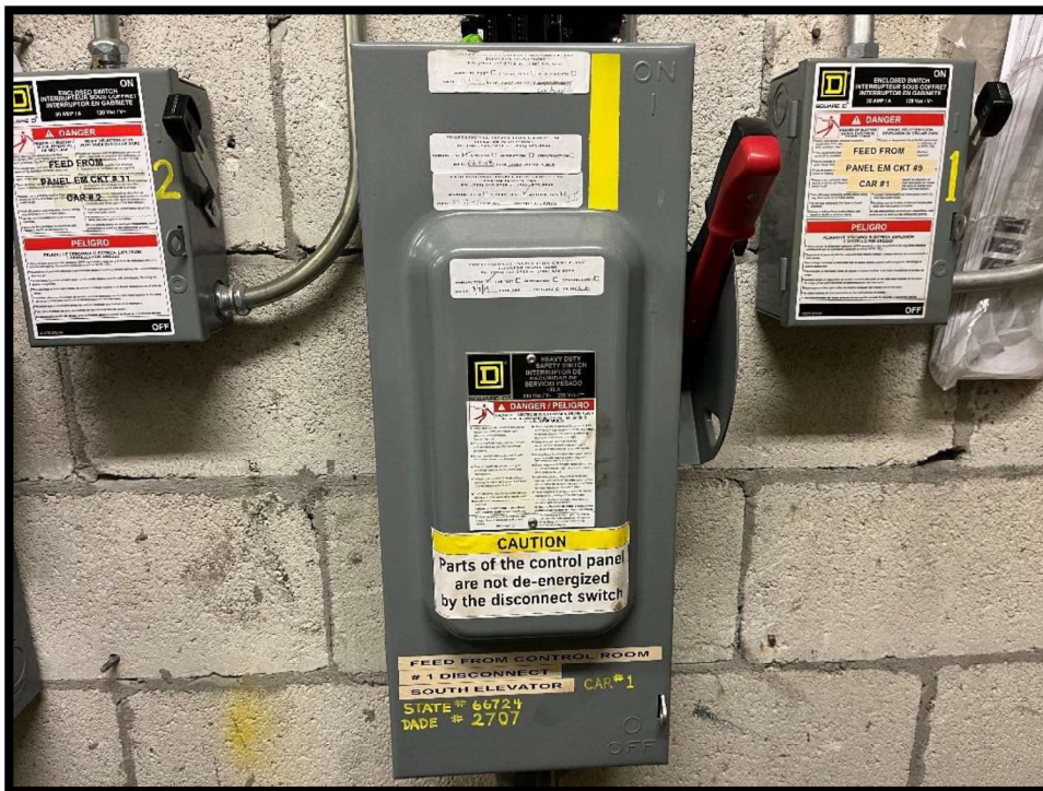
Photograph #52 The Disconnect #1 South Elevator is properly identified. The label shall be of sufficient durability to withstand the environment involved and shall not be handwritten. NEC 210.5 C (1) (b). In the 2020 NEC, Section 705.10, Section 11.12.2.1.5 in NFPA 1.
