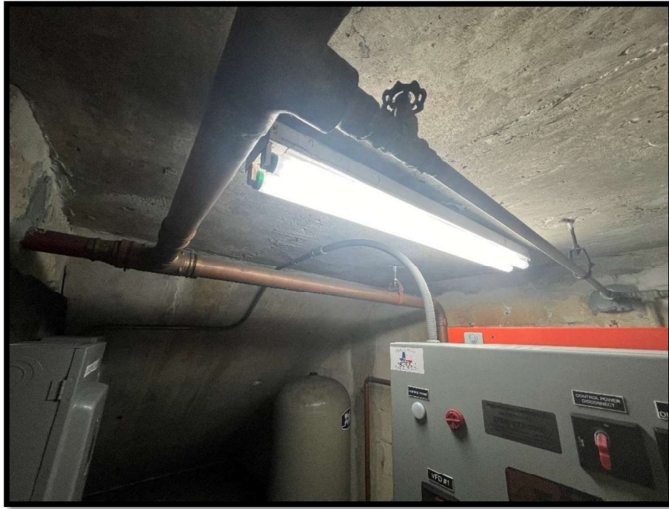
Photograph #75 Fire Pump Room 1 properly lit.
