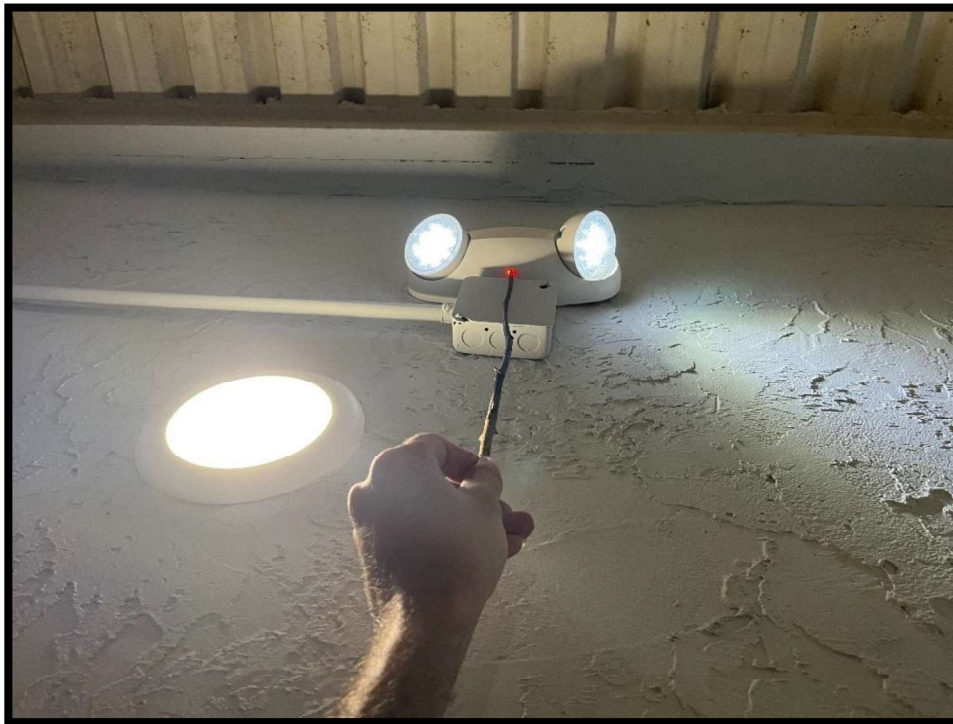
Photograph #176 Emergency lights properly installed and in good working condition.
