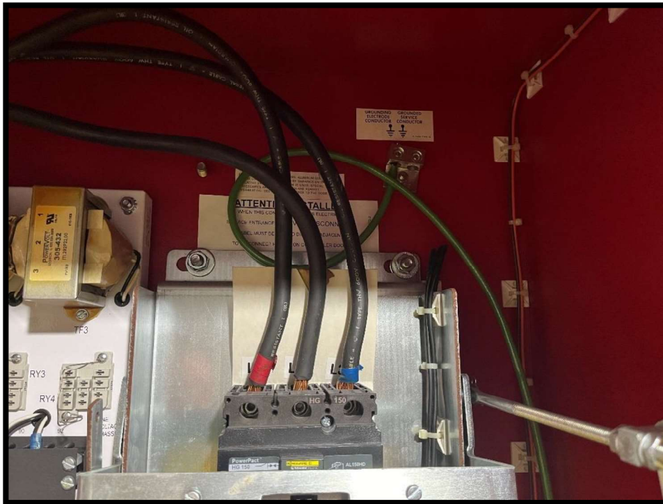
Photograph #79 Grounding is properly installed.
