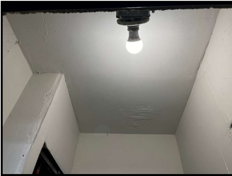
Photograph #134 Electrical room properly lit.
