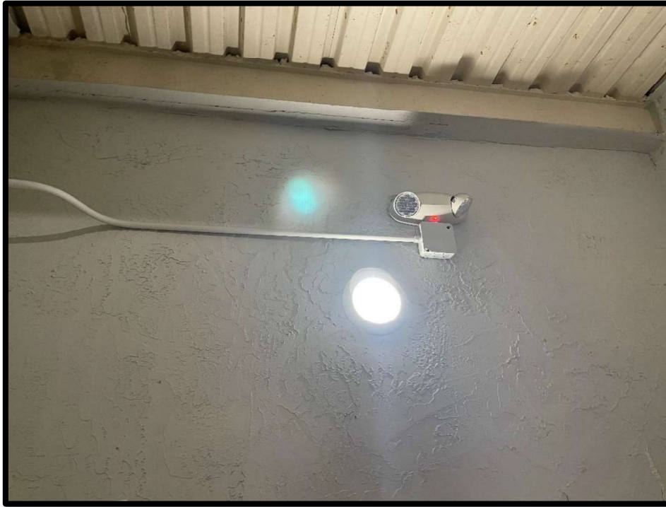
Photograph #208 Emergency light Properly installed and in good condition.
