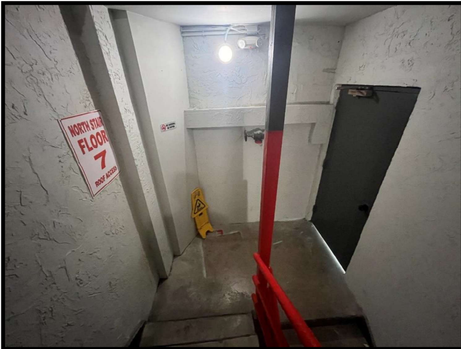
Photograph #169 The stairway landing properly illuminated. Emergency lights properly installed.
