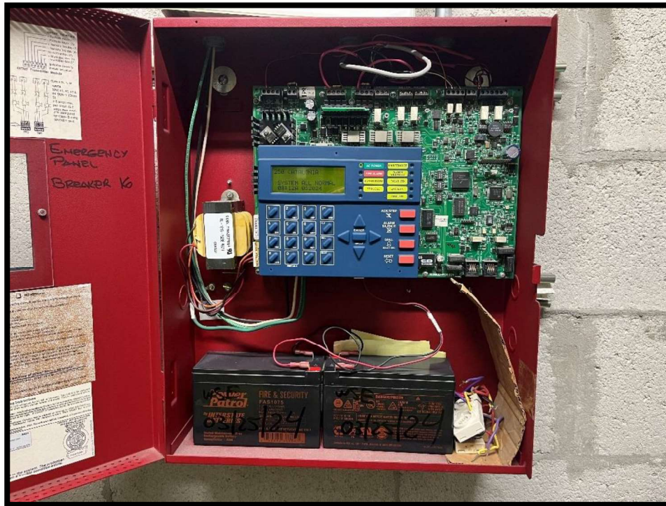
Photograph #24 Fire alarm control panel properly installed.
