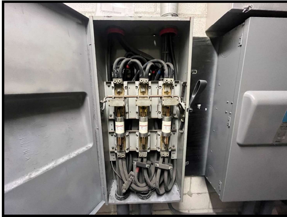
Photograph #4 Phases are properly identified and installed.
