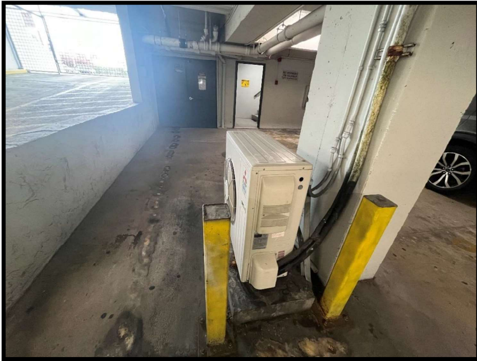
Photograph #59 AC properly installed.
