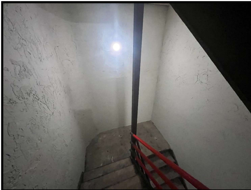
Photograph #177 The stairway landing properly illuminated.
