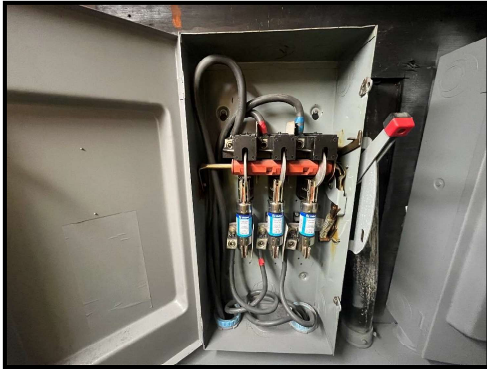
Photograph #65 Phases are properly identified and installed. Fuses are properly identified and installed.
