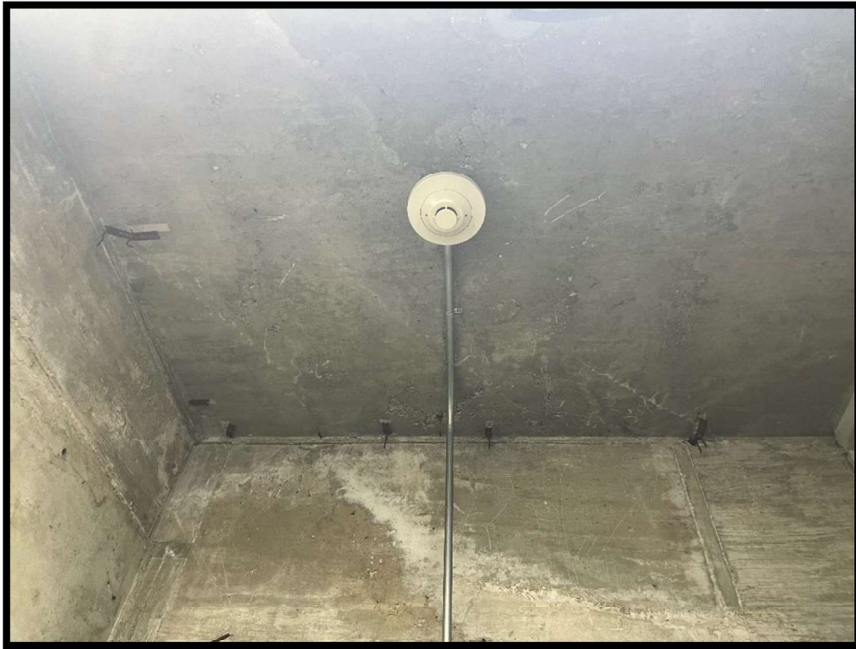
Photograph #37 Smoke detector properly installed.
