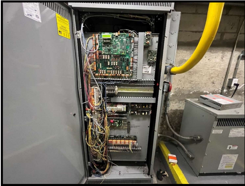
Photograph #41 Elevator Machine 1 properly installed.
