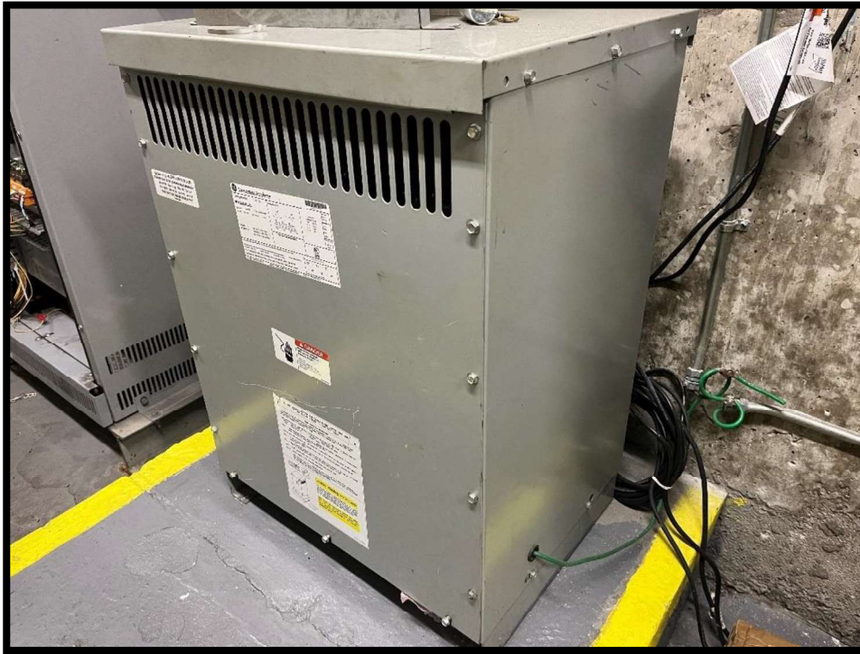
Photograph #43 Transformer 1 properly installed. Grounding is properly installed.
