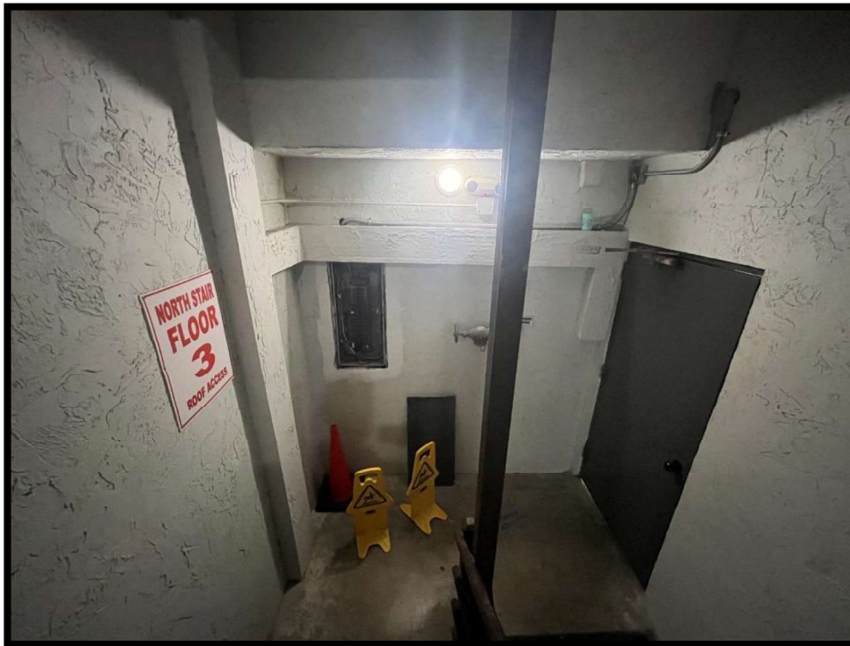
Photograph #180 The stairway landing properly illuminated. Emergency lights properly installed.
