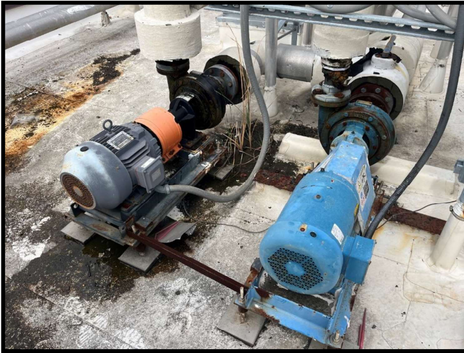
Photograph #163 Ground wire properly connected in the electric motors.
