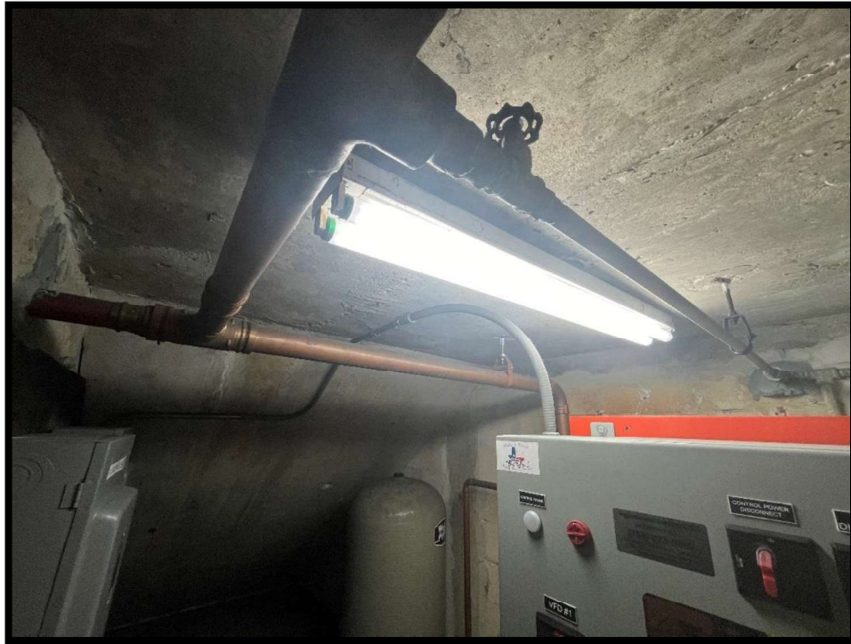
Photograph #75 Fire Pump Room 1 properly lit.
