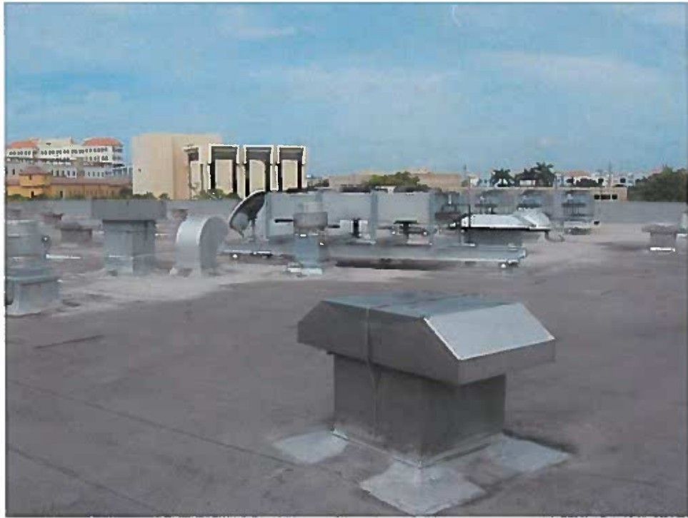
Picture 2: Existing Roof Top Units
