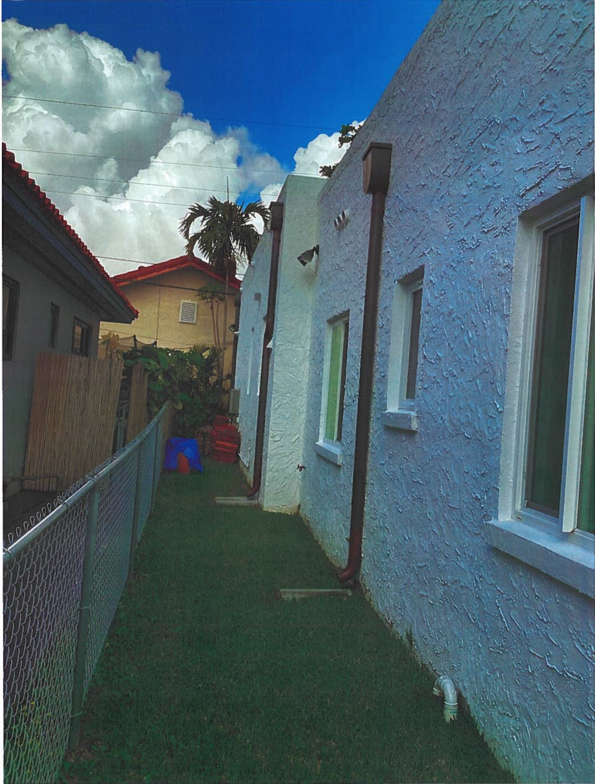
Remove the covered porch addition from the 1950s and replace it with a new Mediterranean Revival style addition
