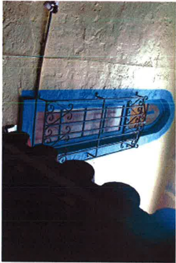
Window at main stair was restored to keep original size and shape.
